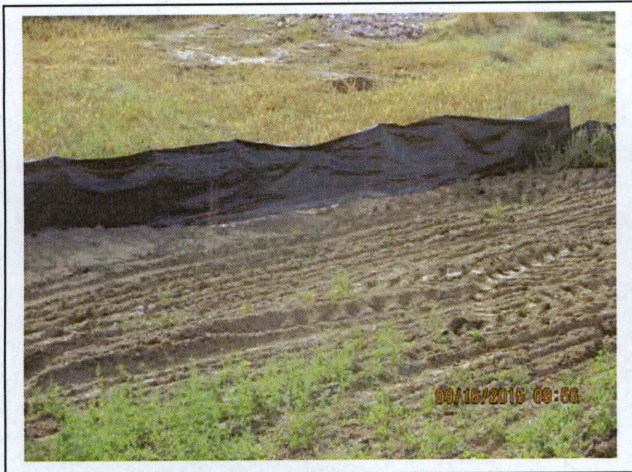
1. West of pond, silt fence installed incorrectly (not keyed in)
