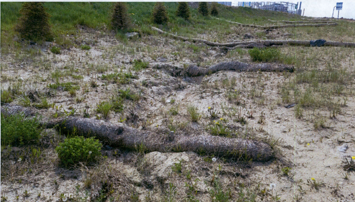
Photo 2 & 3. Wattles along southern edge of Parcel 2 near access road. Rilling/erosion has occurred under the wattles. Recommend re-contouring/grading and replacing ECDs.
