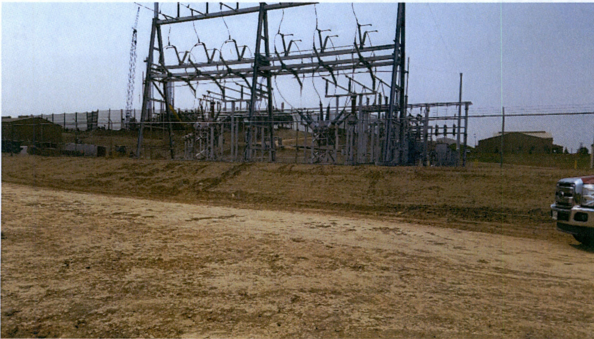
Photo 4. Looking south at electrical substation located within Parcel 3.
