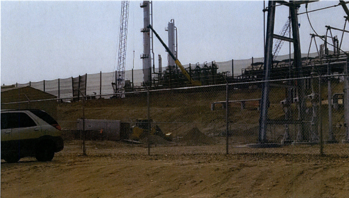
Photo 1. Looking southeast at LMGP IV from electrical substation in Parcel 3. Construction still underway with restoration activities to follow.
