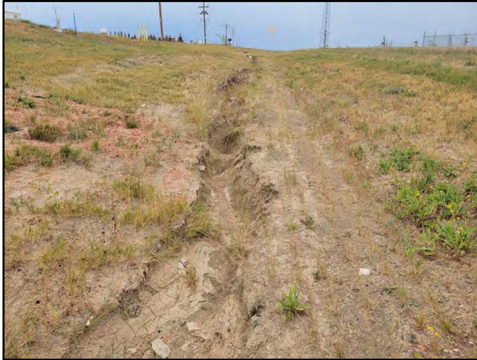
Photo 4. Erosion in the Road ditch on the east side of 125th Avenue NW.
