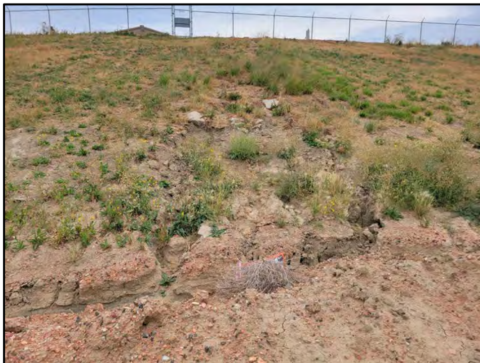
Photo 2. View of run-off erosion from the parking lot of the LMGP, likely due to lack of established vegetation planting.
