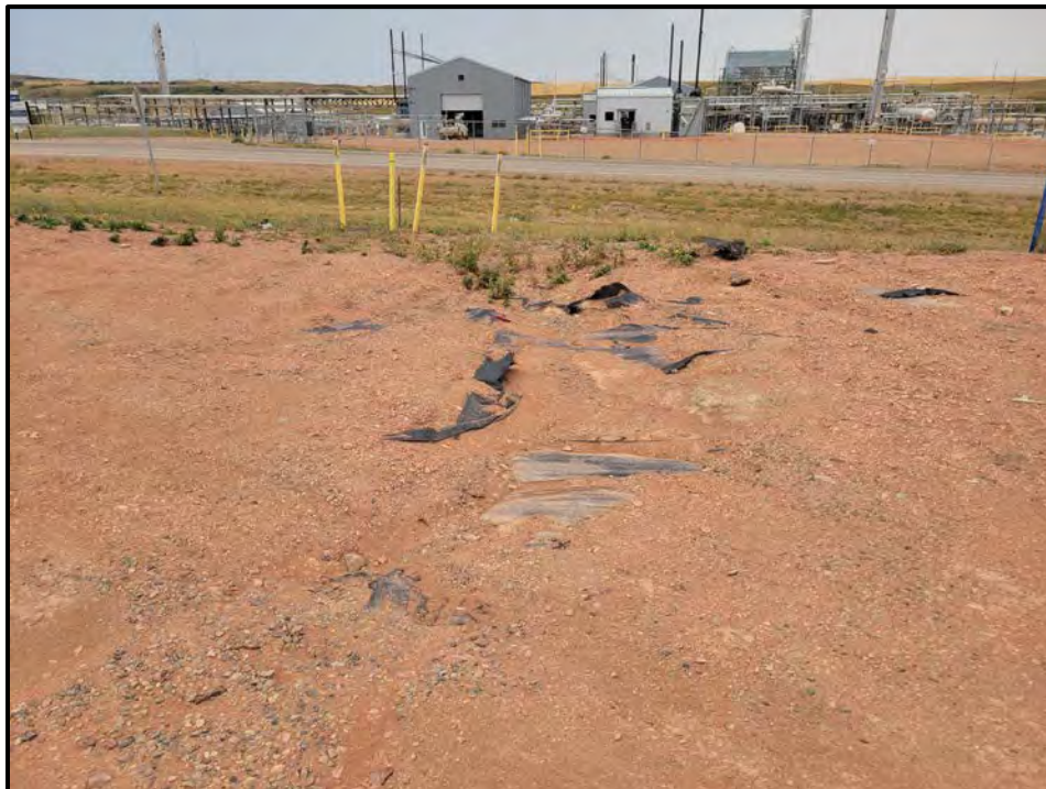
Photo 1. View of surface flow erosion in the main parking area of the Targa Badlands LMGP.
