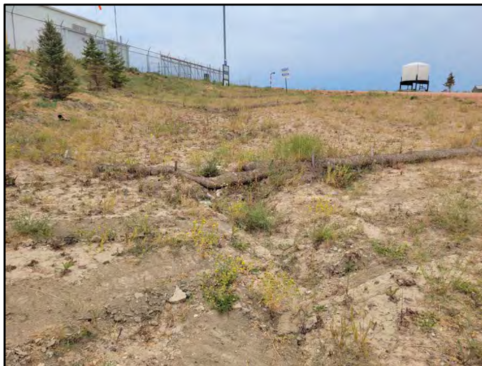
Photo 3. A contoured drain with un-maintained straw waddles. A lack of established grass planting has resulted in erosion.
