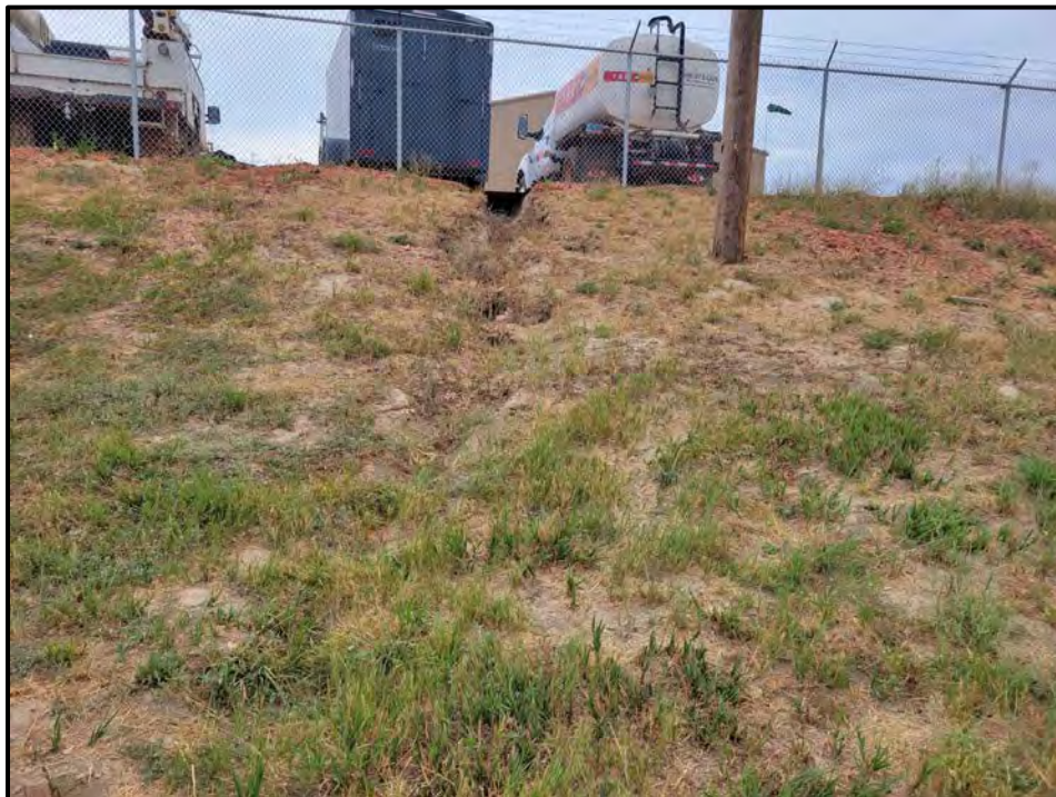
Photo 5. Surface flow erosion coming from parking area in Parcel 2.
