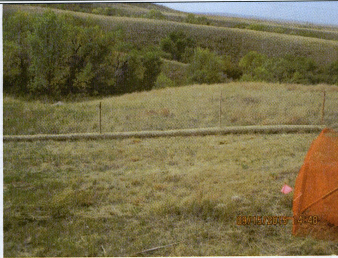
Photograph 9: Station # 281+00, one of many locations of straw logs not properly installed.
