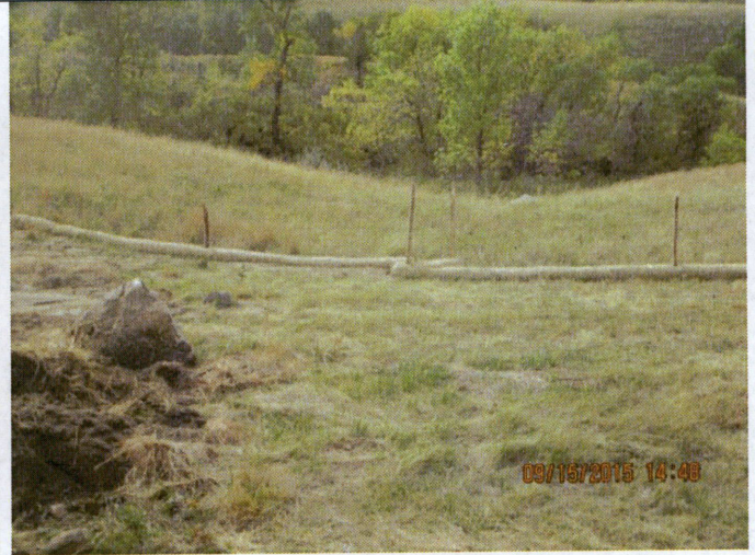
Photograph 10: Station # 283+00, straw logs more than 50% contained with sediments and not installed properly.
