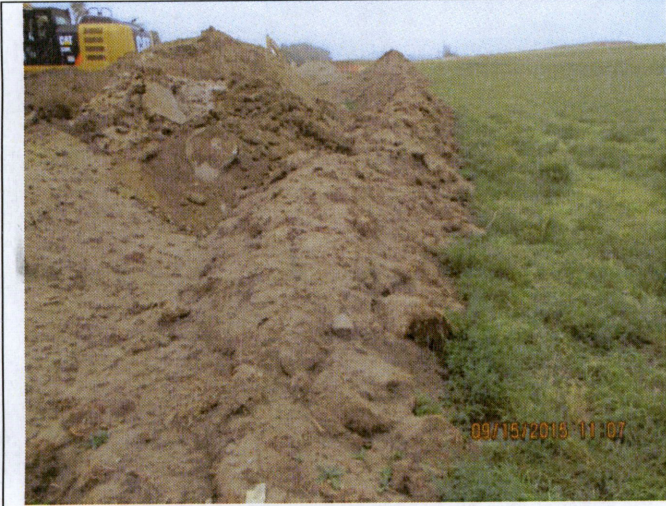
Photograph 1: Station # 984+00, spoil stored up onto stored top soil, top soil is also outside of staked project limits.
