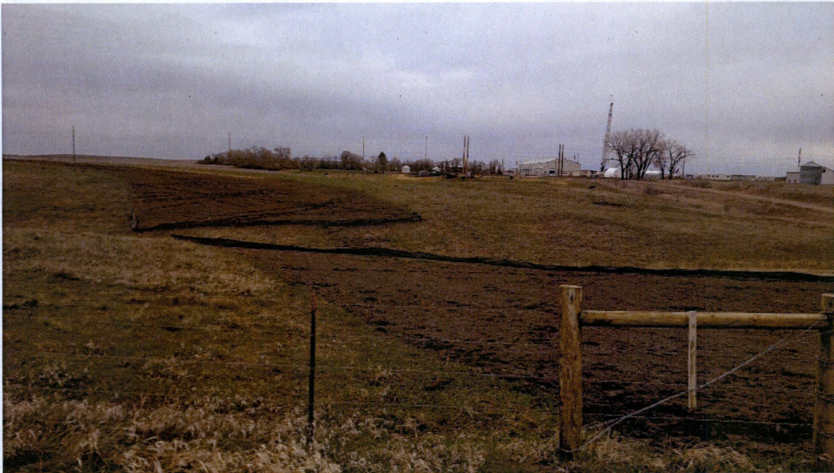
Photo 5. Facing north along the ROW, silt fences providing a barrier for the wetland which had been HDD.
