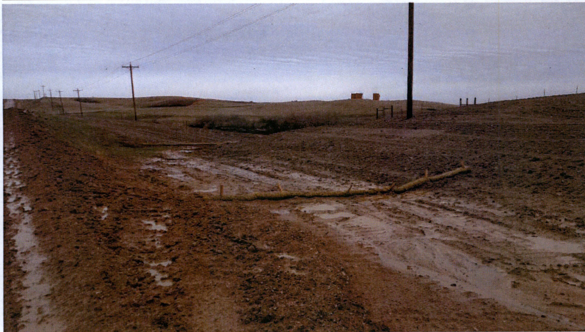
Photo 3. Properly-installed waddles east of the ROW filling with sediment.
