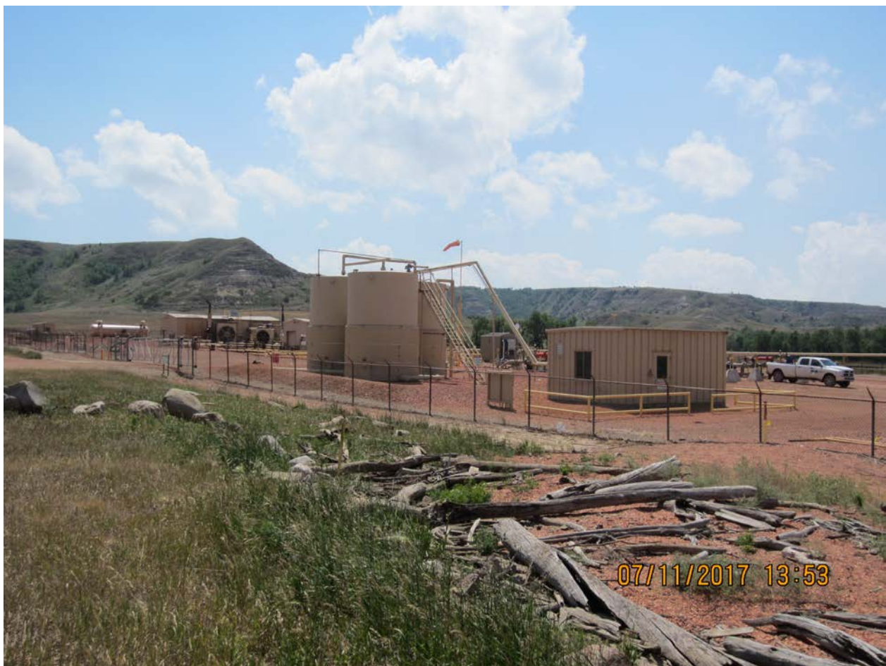
Photo 15: Looking north at the North Charlson Compressor Station
