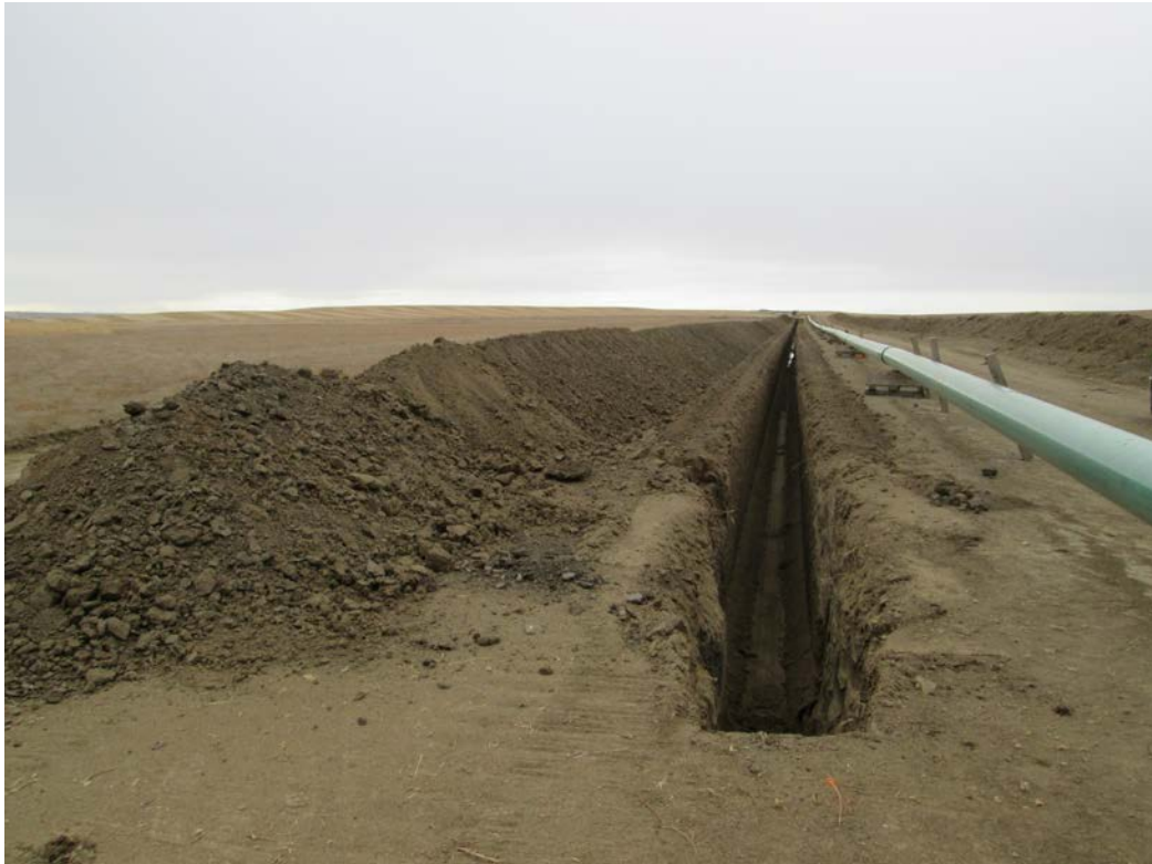
Below: Photo 18 (pt. 213) – Pipe strung next to trench. Subsoil to the left and topsoil pile to the far right. Looking south-southwest.
