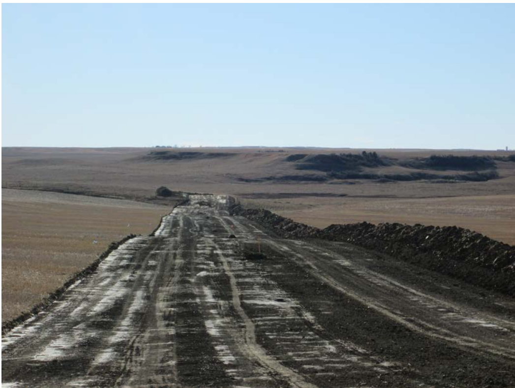
Below: Photo 10 (pt. 208) – Topsoil stripped; can see area that was side-sloped/two-toned in the distance. Topsoil was moved to opposite side; ROW area was leveled. Looking southwest.
