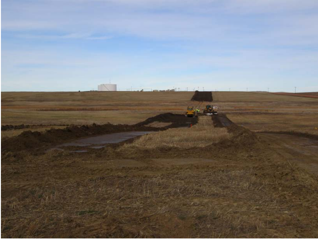
Above: Photo 3 (pt. 202) - Direction looking north toward Skunk Hill Station. Start of topsoil stripping. Parallel pipeline to the right on photo (yellow and orange flags). In some areas soil is lighter near parallel pipeline's ROW.
