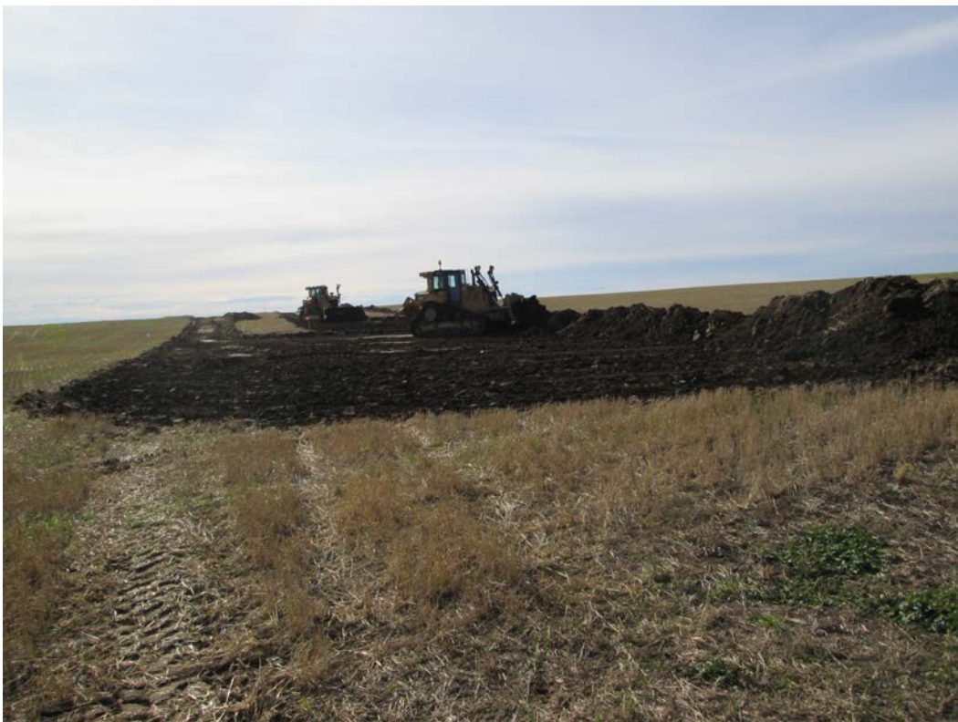
Below: Photo 2 (Point 200) – Direction looking south by Skunk Hill Station. Start of topsoil stripping.
