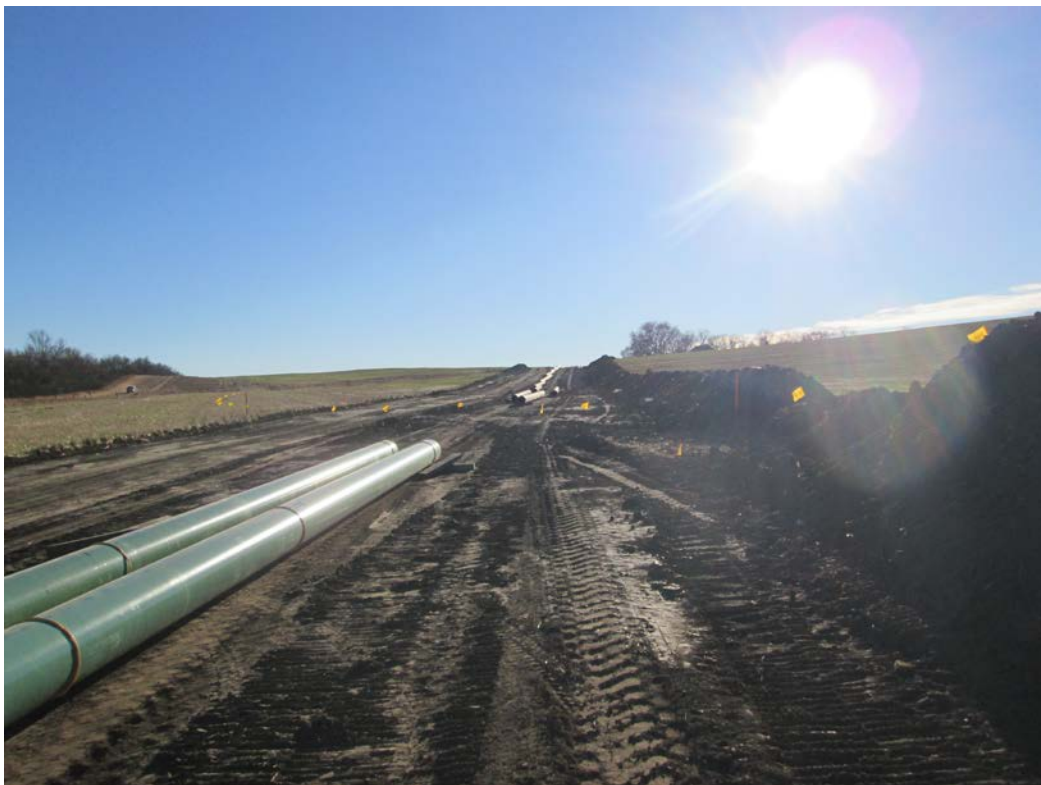
Below: Photo 16 (pt. 212) – Pipe strung in ROW. Two-toning/side-sloping at the top of hill. Yellow pin flags cross through ROW, indicate other pipeline. Looking south-southwest.
