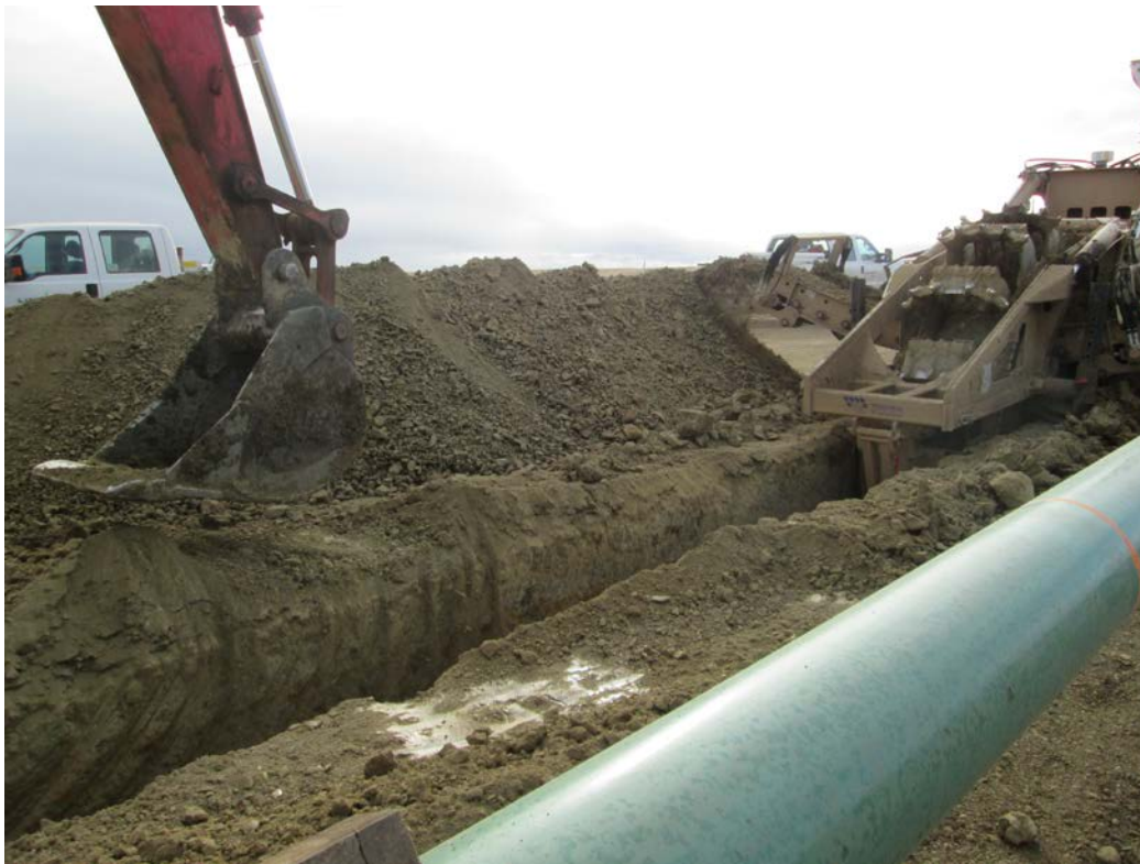
Above: Photo 21 (pt. 215) – Trenching machine removing subsoil. Subsoil pile to the left. Looking south.
