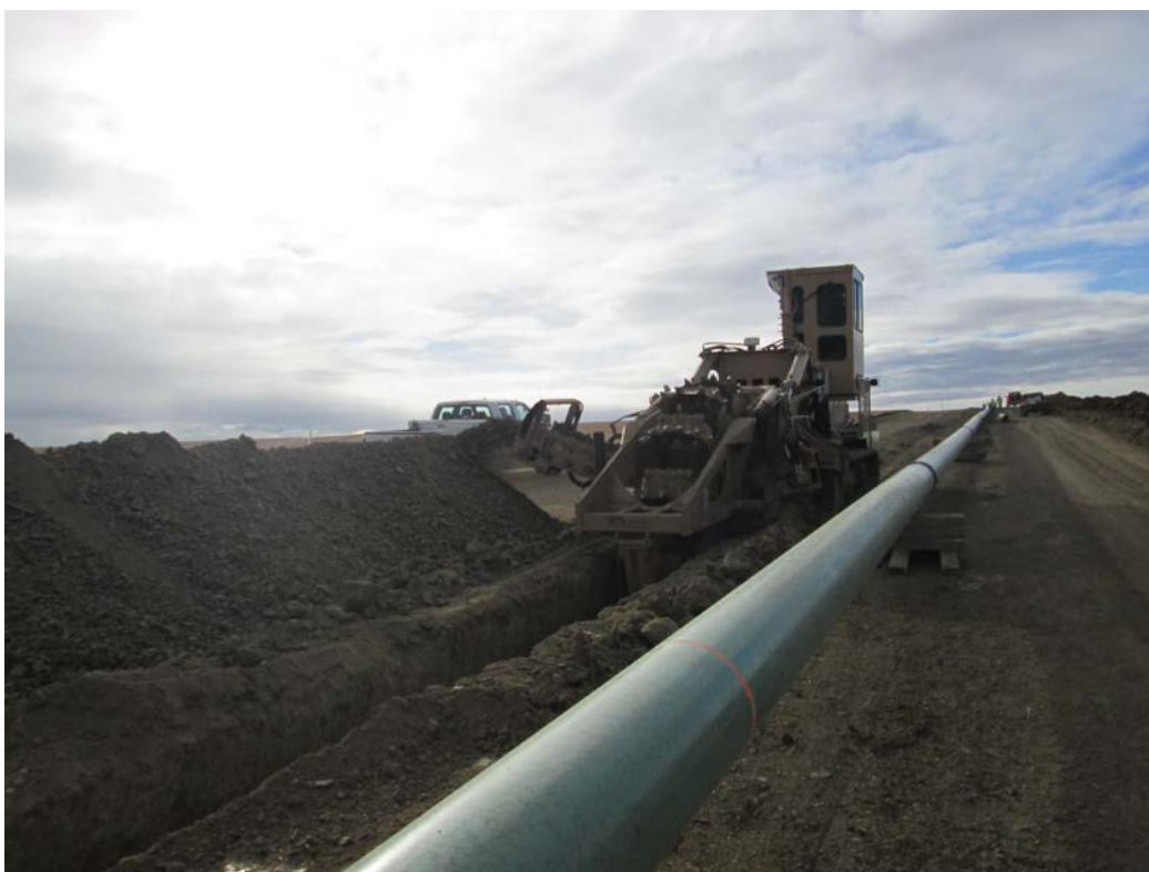
Below: Photo 22 (pt. 215) – Trenching machine removing subsoil. Subsoil pile to the left. Looking south.
