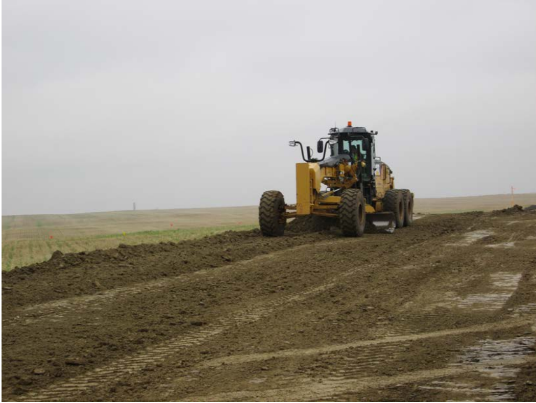
Above: Photo 7 (pt. 204) – Direction looking south. Topsoil stripped, area being finished (leveled off, smoothed and flattened).
