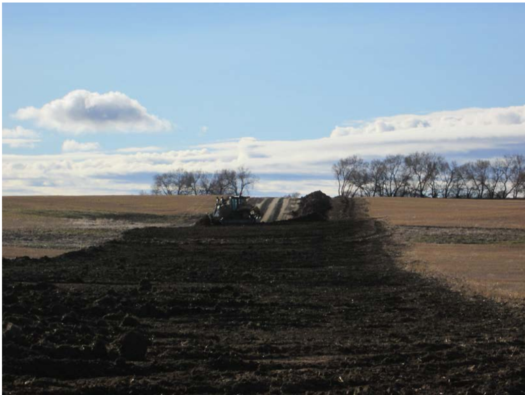
Below: Photo 26 (pt. 219) – Dozer replacing topsoil back over ROW ground. Looking southwest.
