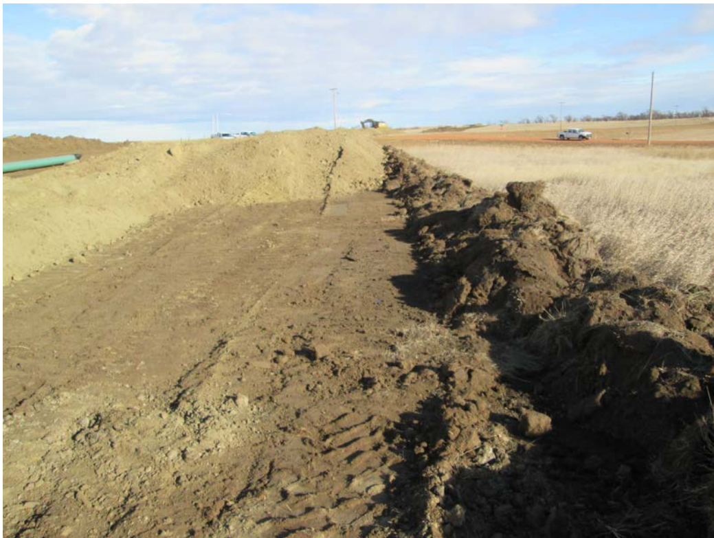
Below: Photo 24 (pt. 217) – Topsoil pile to left of pipe on far left of photo. Bell hole subsoil pile shown in middle of photo is touching small second topsoil pile on far right (darker color) from where they extended the ROW to 100ft. Looking north-northeast toward 30 th St.
