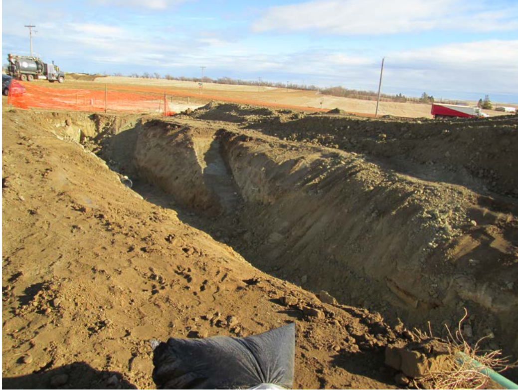
Above: Photo 23 (pt. 217) – Bell hole needed for tie-ins. Larger amount of subsoil needed to be removed for slope and work space. Looking north-northeast toward 30 th St.
