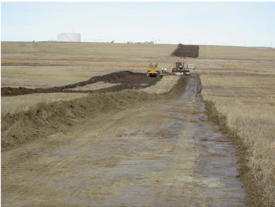
Below: Photo 4 (pt. 202) – Direction looking north toward Skunk Hill. Parallel pipeline to the right on photo (orange flags). In some areas soil is lighter near parallel pipeline.
