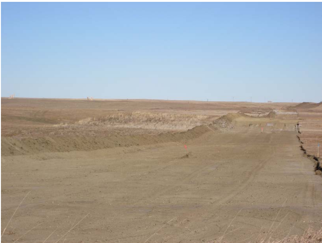
Below: Photo 12 (near pt. 209) – Pipeline ROW, topsoil to the left. There are two white areas that appear to from saline/alkaline deposits. Looking north-northeast.
