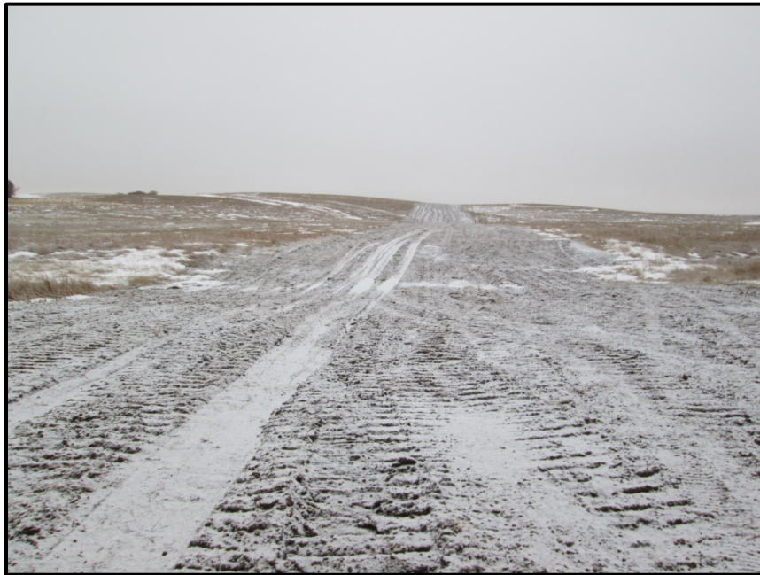
Photo 2. Direction: Southwest (GPS Point #223). Open cut wetland, did not use the full ROW to reduce impacts to the area. This wetland was not originally on Bridger's maps, but their environmental inspector said it was a wetland (note cattails on edges in photo).
