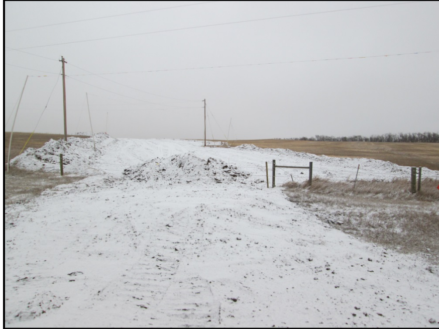
Photo 3. Direction: Northeast (GPS Point #224). Road bore work area for unnamed road used 100ft ROW. Topsoil piles observed on the sides, subsoil pile in middle, not all subsoil has been replaced.
