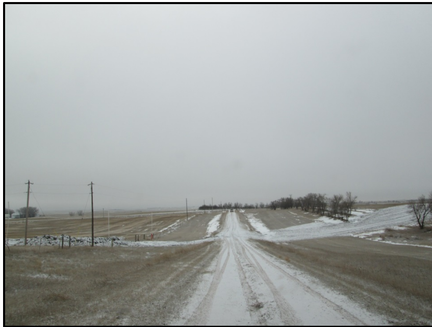
Photo 4. Direction: South (GPS Point #224). Road bore (unnamed road); pipeline passed through a break in a tree row (on right); avoided impacts to trees within ROW. On the right of the road, soil has been replaced; on the left of the road, topsoil and some subsoil still had to be replaced.
