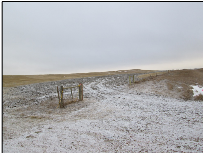
Photo 8. Direction: Southwest (GPS Point #228). Road bore work area; pipeline going west through agriculture field.
