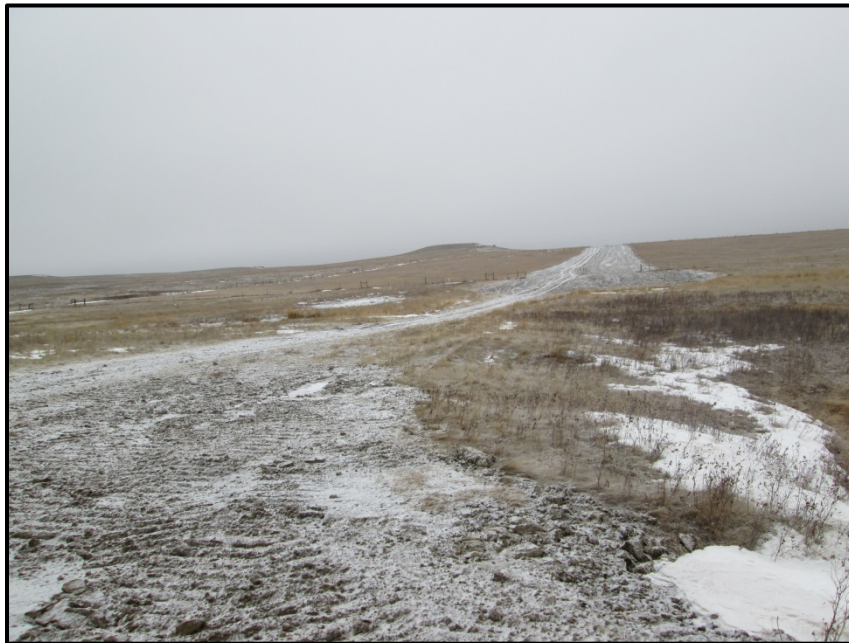
Photo 6. Direction: North (GPS Point #226). Pipeline bored underneath wetland with minimal impact. Trucks had been driving on higher frozen ground near wetland; this could be an area of concern for soil compaction, especially if area is wet rather than frozen.
