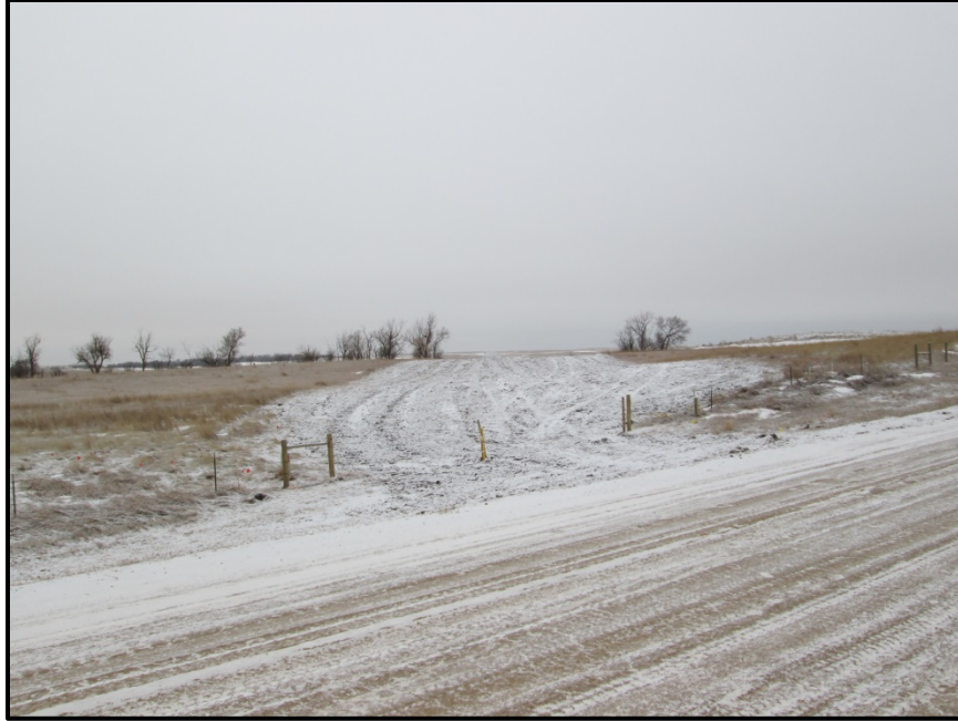
Photo 1. Direction: Southwest (GPS Point #222). Road bore work area for 30 th St. used 100ft ROW.
