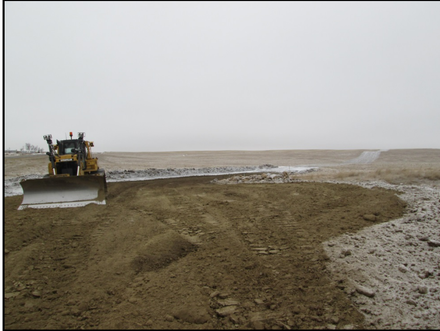
Photo 5. Direction: North (GPS Point #225). Pipeline road bore area for 32 nd St. bore. Topsoil piles visible along sides of ROW. Backfilling area had just been completed.
