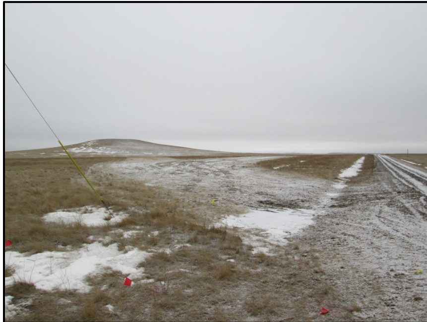
Photo 10. Direction: West (GPS Point #230). Road bore area near 134 th St. (not pictured). Pipeline continues on to Forest Service Land, which is prairie.
