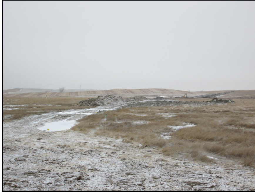
Photo 7. Direction: North (GPS Point #227). Pipeline bored underneath wetland area, topsoil piles along sides, extended ROW to 100ft for bore pull-back/work area. Topsoil had been replaced on south bore side, but not north side. Discing and reseeding have not been completed for any of the project. Trucks have been driving on higher frozen ground near wetland; this could be an area of concern for soil compaction, especially if area is wet rather than frozen.
