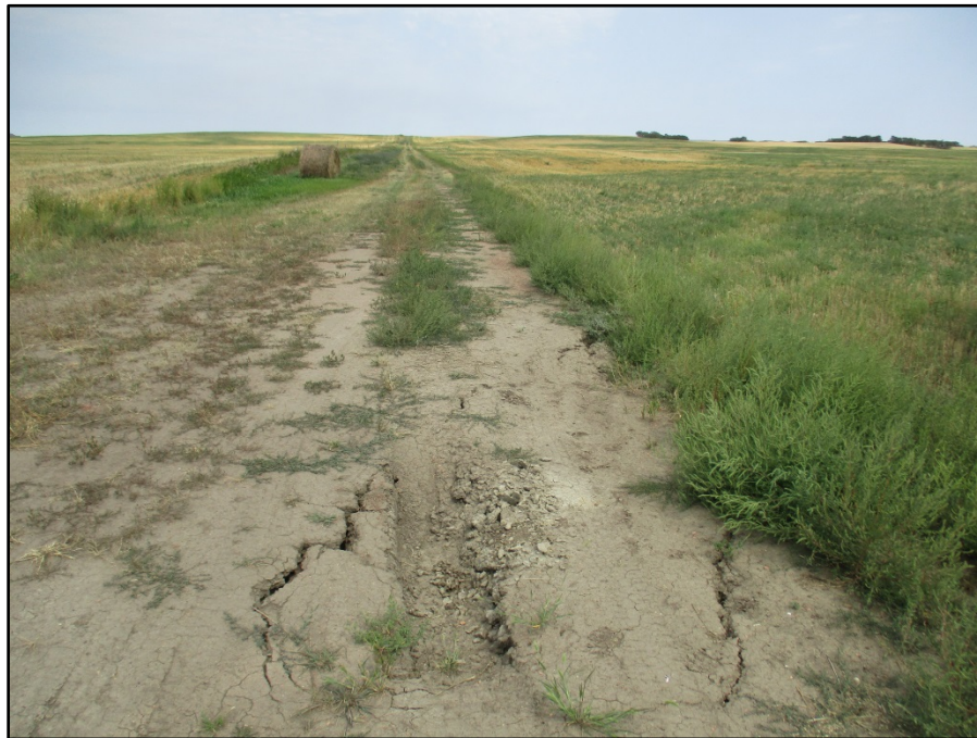
Photo 18. (GPS Point #476) – Pipeline ROW veering off to the right of photo. The two-track road is an unimproved section line. The company used bore pipe here and went down deeper than the typical ROW (as needed for an unimproved section line). There is soil subsidence in road area. The company is aware of this soil subsidence and will be addressing it soon. Direction: North.
