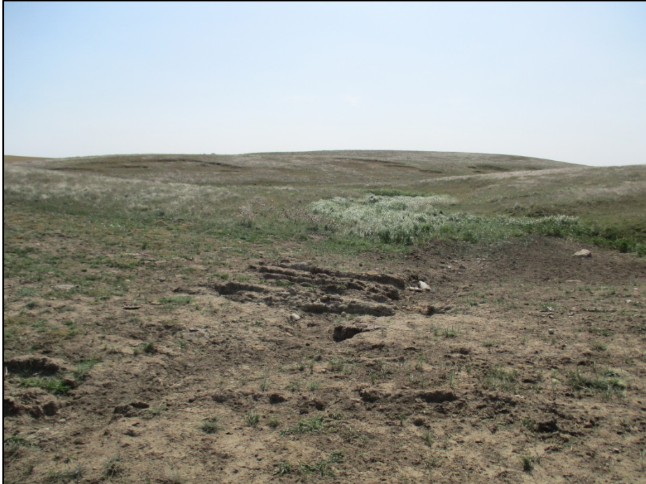
Photo 14. (GPS Point #473) – Upland drainage area, which has started to erode. Area will need to be fixed and erosion control devices should be added. Bridger is aware of this location and will be addressing and should provide documentation to PSC.
