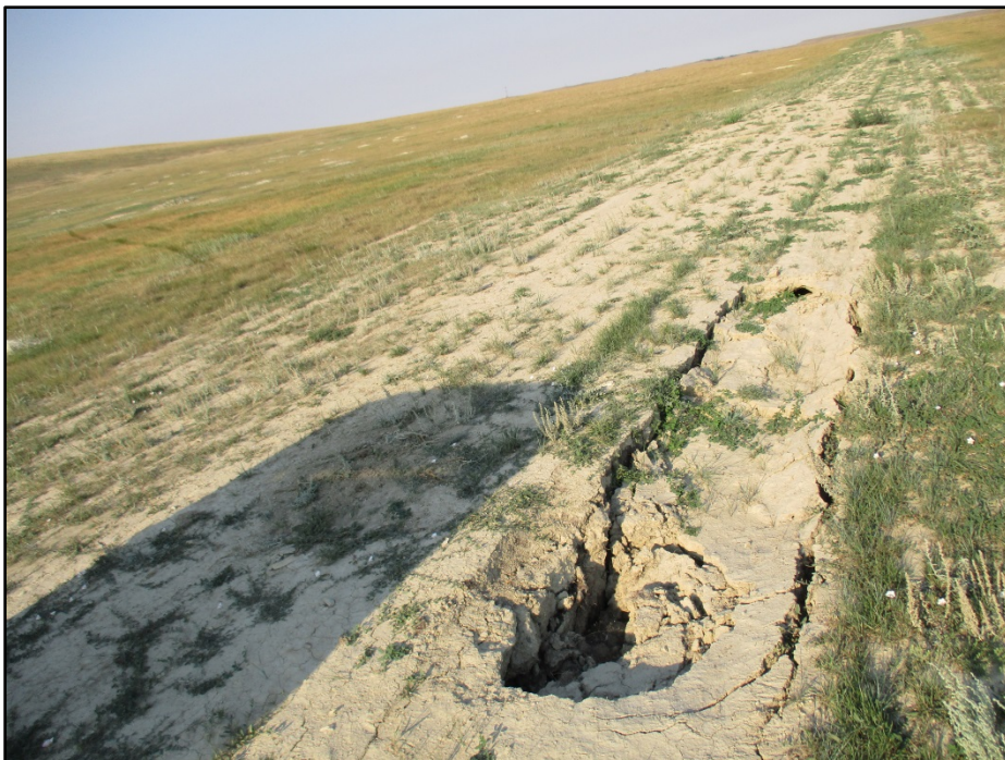
Photo 2. (GPS Point #461) – Soil subsidence in grassland on USFS lands. This area will need to be restored. Bridger is aware of this and will address the settling issue soon. Notice the narrow ROW, this area was double ditched as requested by the U.S. Forest Service. Direction: West.
