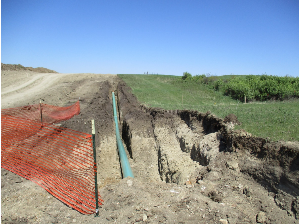
Above: Photo 23 (pt. 292) – Open trench, with only partial fence around area.
