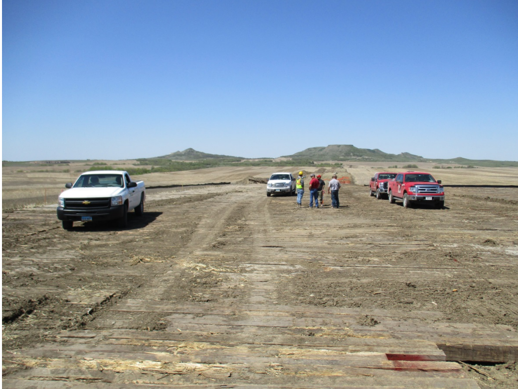
Above: Photo 35 (pt. 294) – Lake Sakakawea bore location with mats and some silt fences placed along area. Observed May 17, 2016. Direction looking west.
