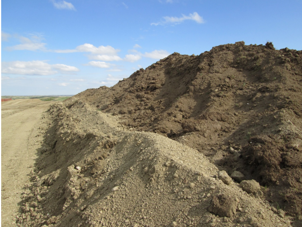
Above: Photo 17 (pt. 286) – Topsoil pile to the right of photo. Subsoil pushed on top of the bottom of the topsoil pile.
