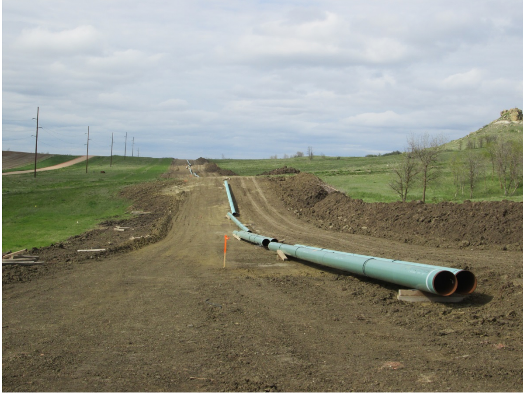
Above: Photo 13 (pt. 282) – Topsoil pile to the right of photo. Topsoil pile was moved from the left to the right side of the ROW. Direction looking north.
