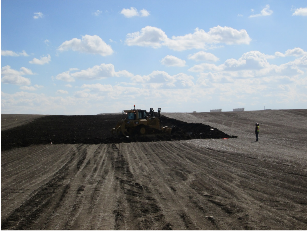
Above: Photo 5 (pt. 233) – Start of topsoil stripping on cropland near the Keene terminal. Spotter to the right of photo to make sure topsoil pile stays in the ROW. Soil was dry. Direction looking south.
