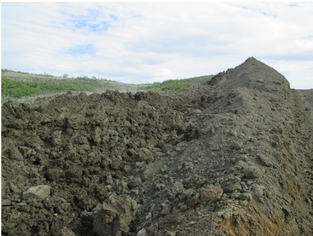
Below: Photo 14 (pt. 283) – Two-tone area. Subsoil pile appears to be pushed into and on top of the topsoil pile. There needs to be separation between the topsoil and subsoil piles. Direction looking south.
