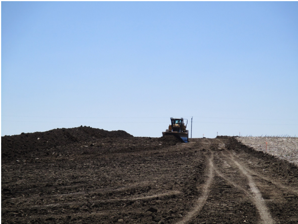
Below: Photo 28 (pt. 298) – Dozer stripping topsoil, pile to the left of photo.
