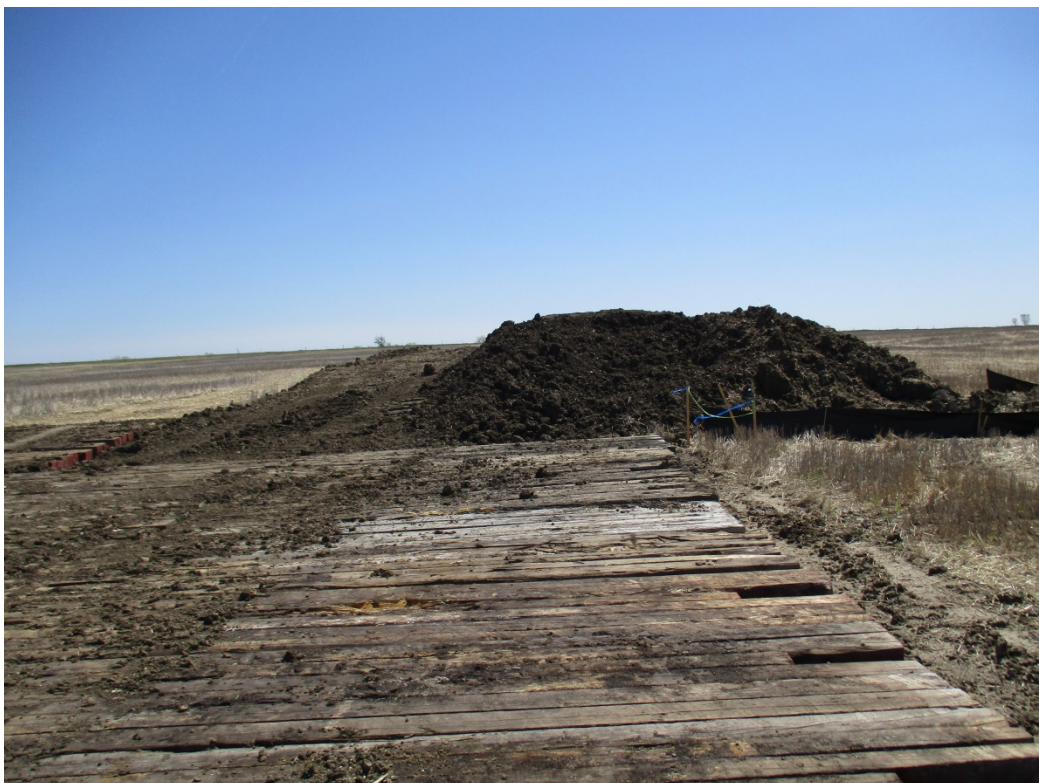
Below: Photo 36 (pt. 294) – Lake Sakakawea bore location with mats and some silt fences placed along area. Topsoil pile near mats with partial silt fence. Direction looking east.
