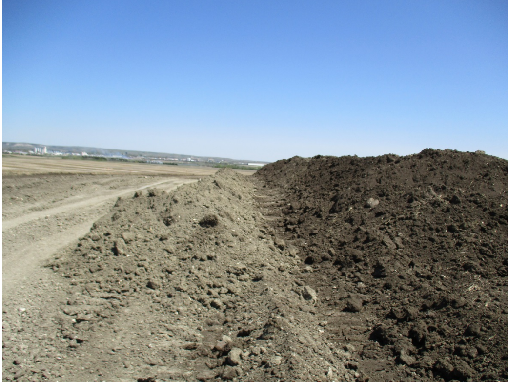
Above: Photo 27 (pt. 296) – Topsoil and subsoil pile with space between them. Work done after May 12, area observed on May 17, 2016.
