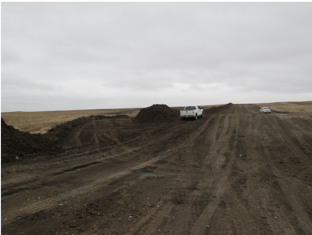
Below: Photo 6 (pt. 234) – ROW and bore pull back area. The additional ROW to the left of the photo is for additional work space for the bore. Direction looking east.
