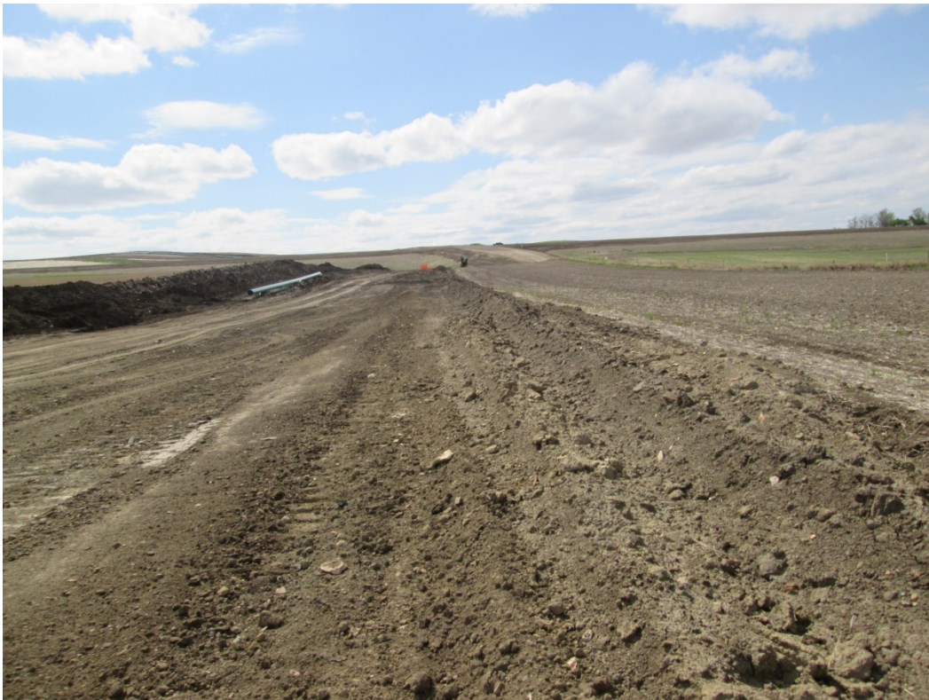
Below: Photo 10 (pt. 279) – Topsoil stripped, on far left; Subsoil was on right side. Pipe has been buried; area still needs to be finished/smoothed. Direction looking east.
