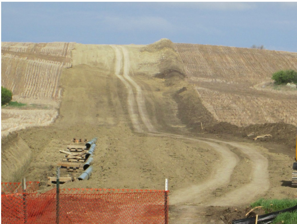
Below: Photo 18 (east of pt. 288) – Most of the trench has been backfilled to the left of photo. Topsoil on the right, notice the light soil colors in the piles and consistent volume excavated across the topography. Direction looking east.
