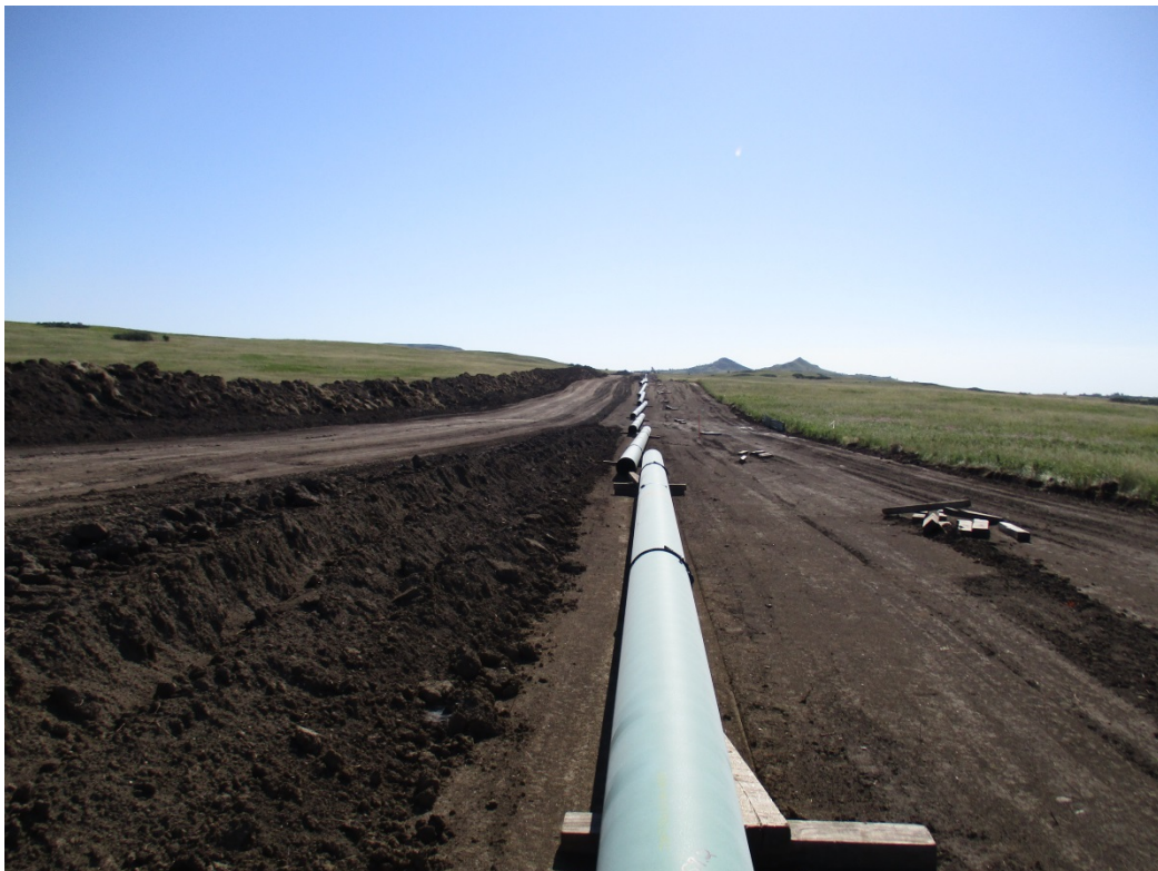
Below: Photo 30 (pt. 443) – Two-tone area, topsoil pile to the left. Looks to be an inadequate amount of topsoil was stripped. Notice the dark colored two-tone subsoil pile area.
