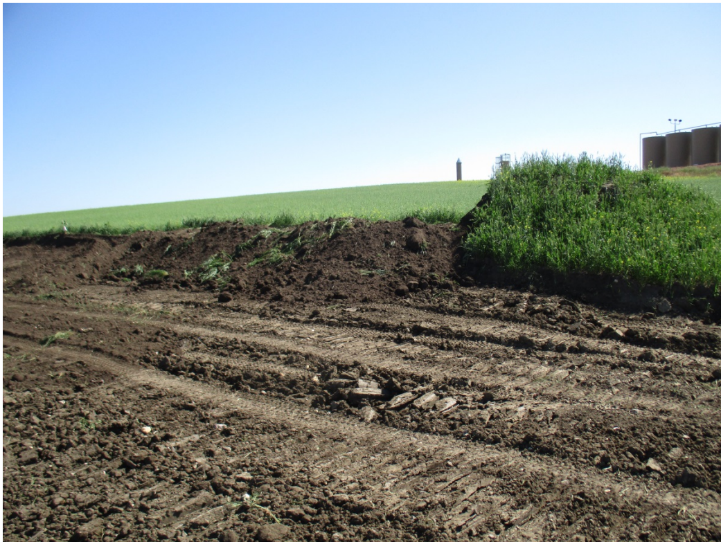
Below: Photo 32 (pt. 445) – Unfinished, started topsoil replacement. Vegetation growing on topsoil pile, part of pile replaced back on ROW. Direction looking northeast.
