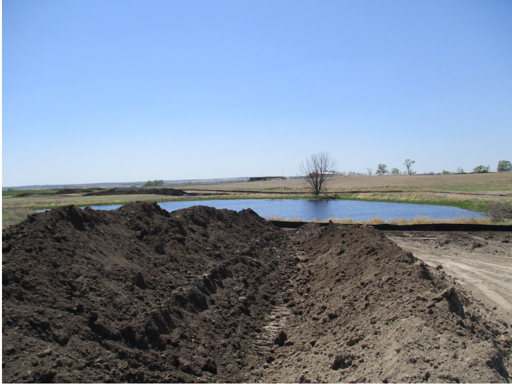
Above: Photo 29 (pt. 300) – Bore area near wetland. Access road located on the right, going around the wetland. Topsoil and subsoil piles have space between them. Silt fence near wetland. Direction looking west.
