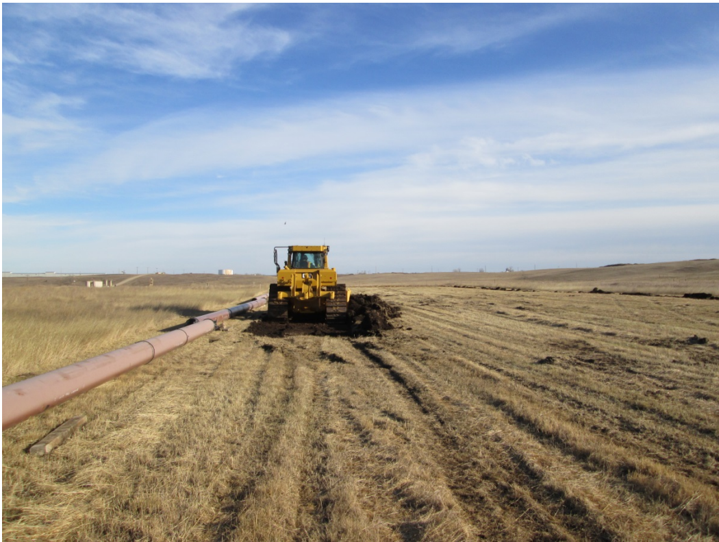
Below: Photo 2 (Point 232) – Start of topsoil stripping. Bore pipe along the left side. Direction looking north toward Palermo station.
