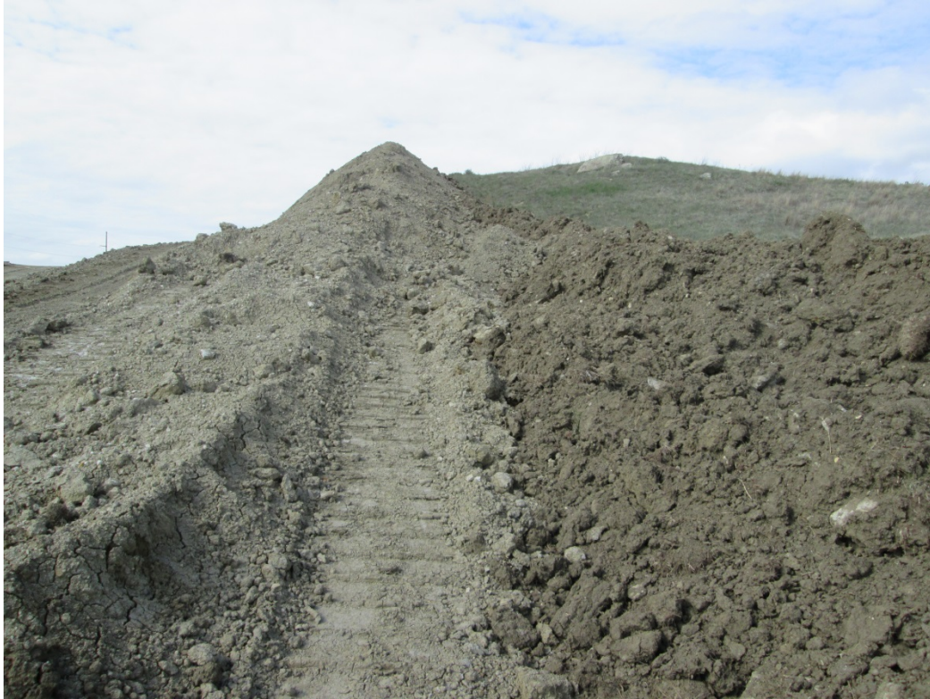
Above: Photo 15 (near pt. 283) – Two-tone area. Subsoil pile appears to be pushed into and on the topsoil pile. There needs to be separation between the topsoil and subsoil piles. Looking north.
