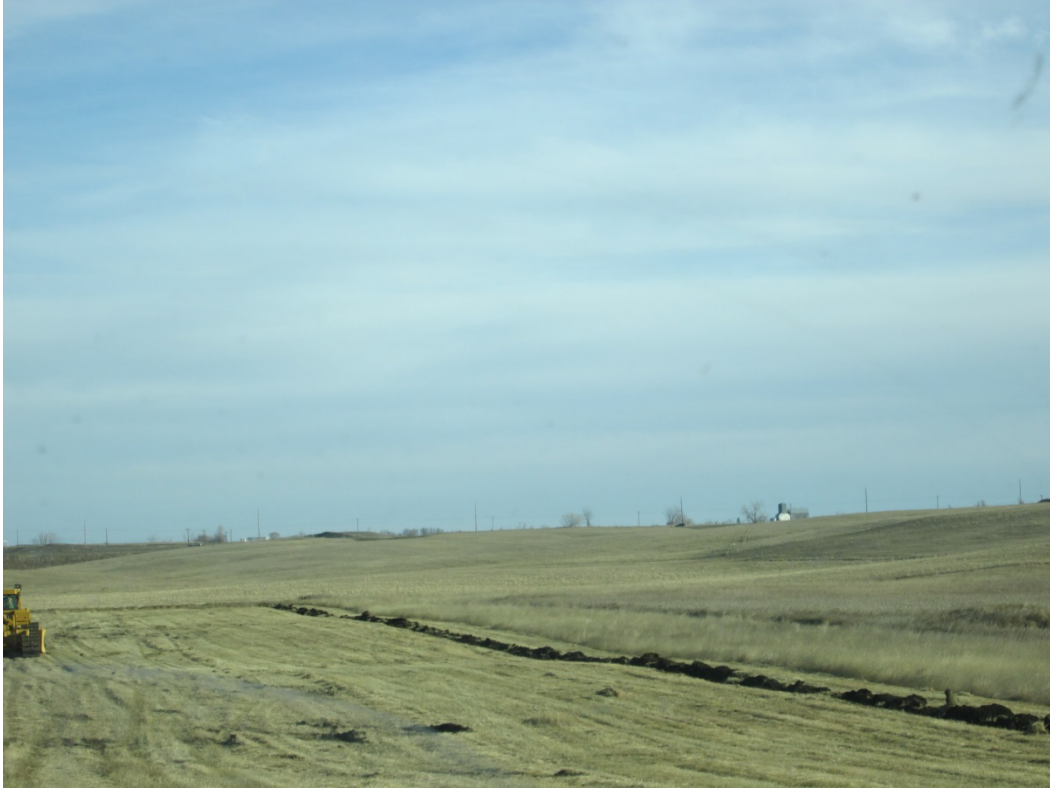
Above: Photo 1 (Point 232) – Start of topsoil stripping. The far right of the photo you can see where the dozer scraped a line in the ground for the topsoil pile to be placed, to stay in the ROW. Grass was previously mowed. Direction looking north.
