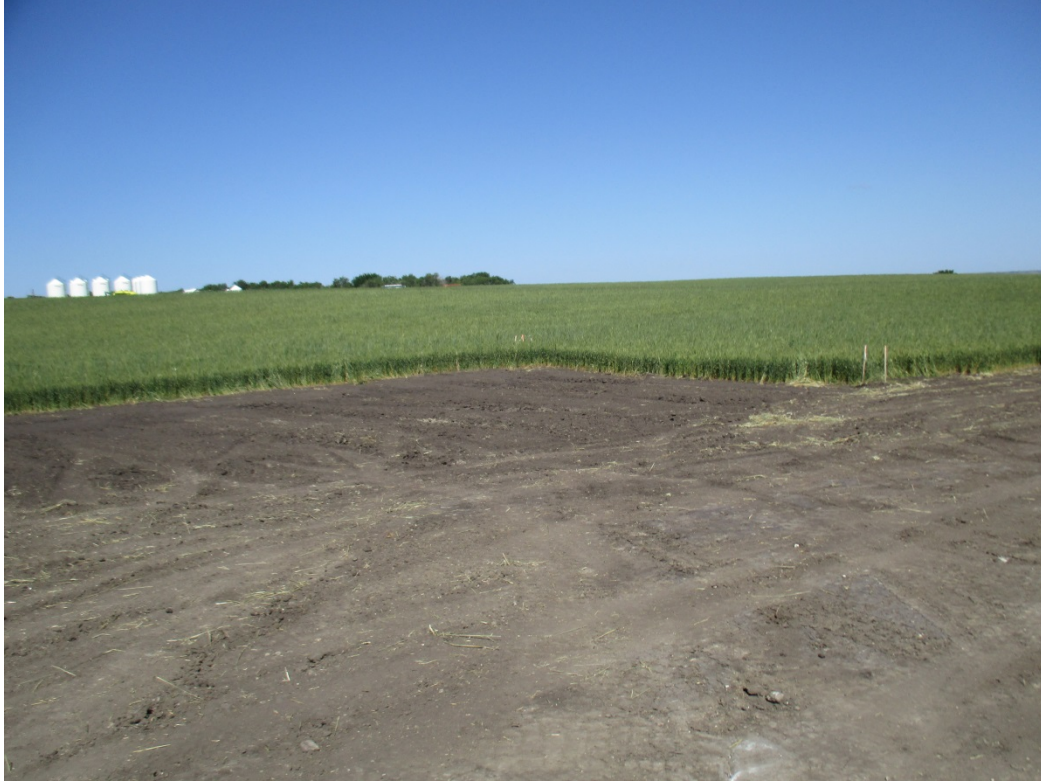
Above: Photo 33 (pt. 447) – Topsoil replaced on ROW and extended ROW for bore area. Contours appear to match up. Direction looking northwest.
