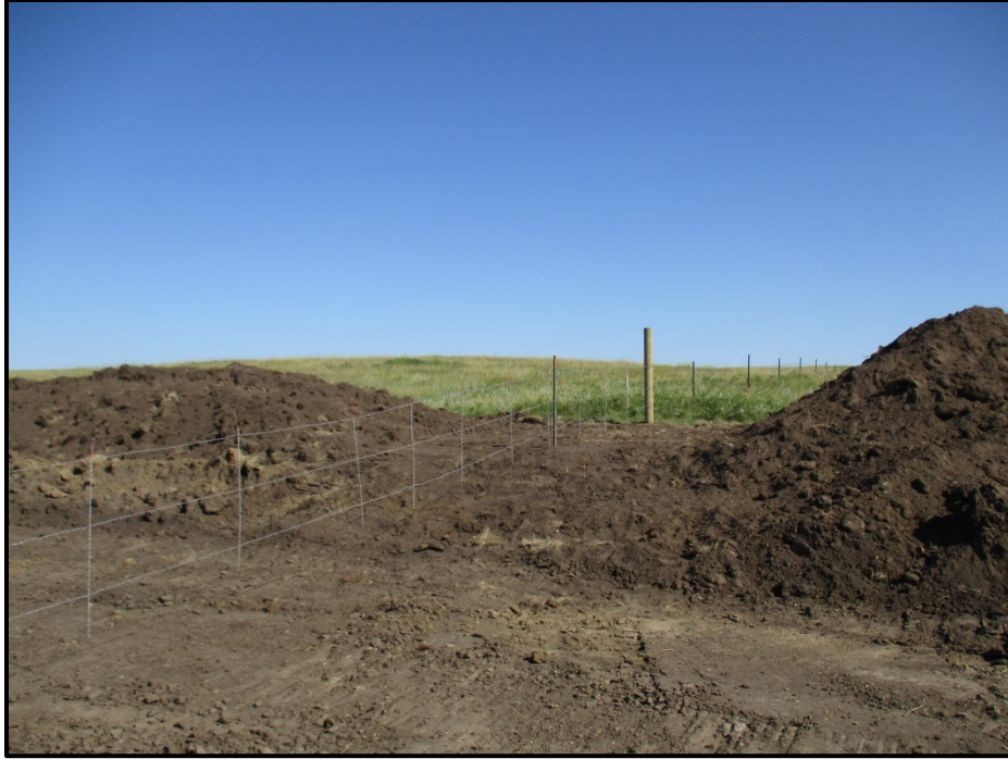
Photo 1. (GPS Point #443) – Temporary gate for fence put up across the ROW. Site visit 7/21/2016.
