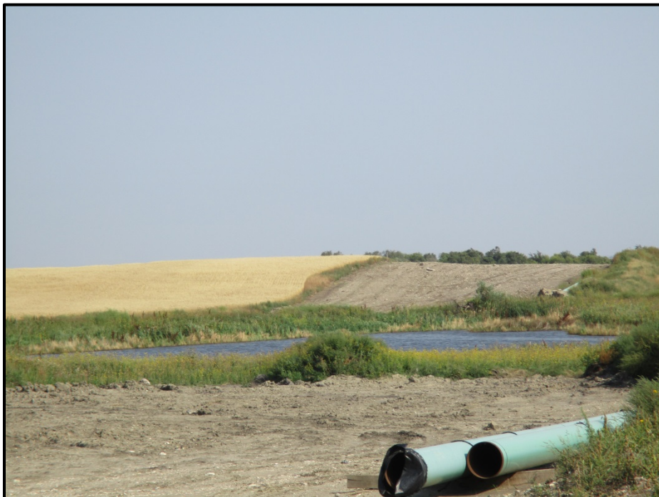
Photo 22. (GPS Point #485) - Pipeline ROW goes down the hill in the distance and wetland was bored under. No erosion control devices observed. Direction: North
