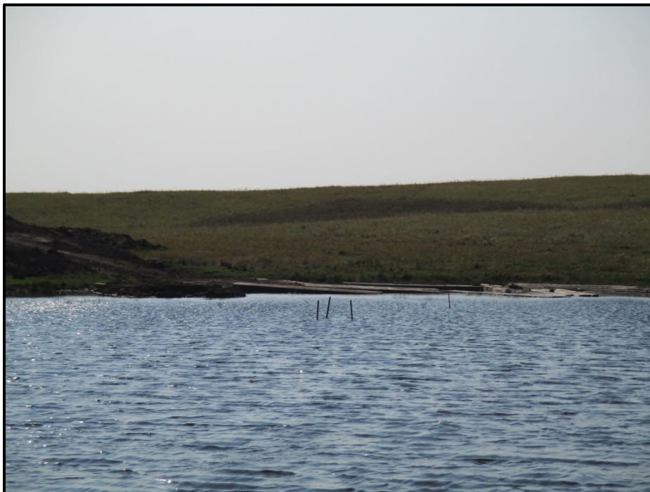
Photo 20. (GPS Point #483) - Swamp mats floating in wetland. Dirt pile in water seen to left of photo on wetland edge. No erosion control devices observed. Direction: South
