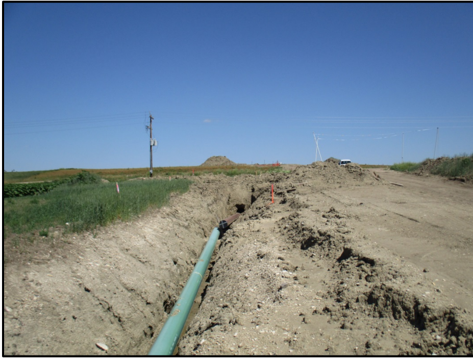
Photo 13. (GPS Point #444) - Area near rural water line break. Open trench to the left of photo. No standing safety fence observed. Environmental inspector thought they hit the rural water line while they were doing boring activities. Direction: North
