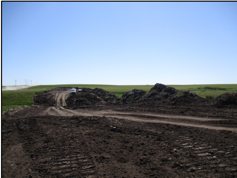
Photo 2. (GPS Point #446) – Drainage area intersected by ROW. No erosion control devices were in place and the corridor had not been necked down in this area to reduce disturbance. Direction: East.
