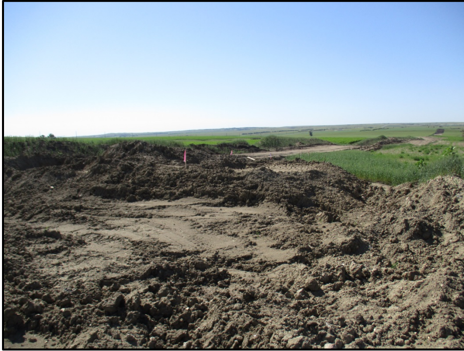
Photo 15. (GPS Point #444) - Area near rural water line break. Looks like subsoil had been pushed around, there was some ponded water in back of photo. Direction: South
