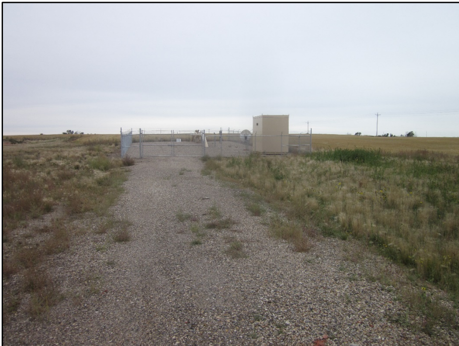
Photo 12. (GPS Point #614) Direction: South. Valve setting in corner of wheat field on south side of 56 th St NW. Setting and access road appeared to be well-maintained. Fenced and locked facility. Vegetation around facility had been disturbed during construction and was primarily annual weeds and foxtail barley.
