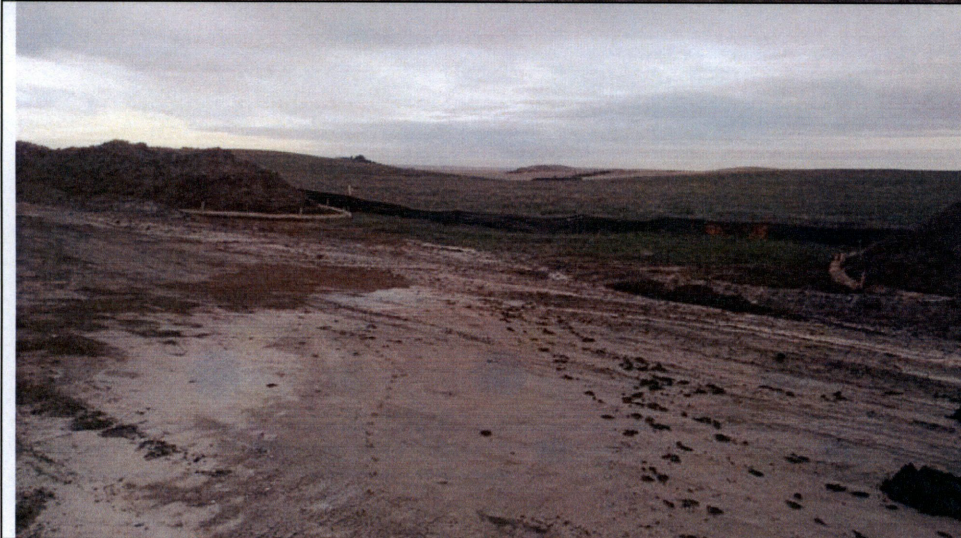
Photo 9: Looking south in Section 31 at erosion control at a drainage swale along the ROW.
