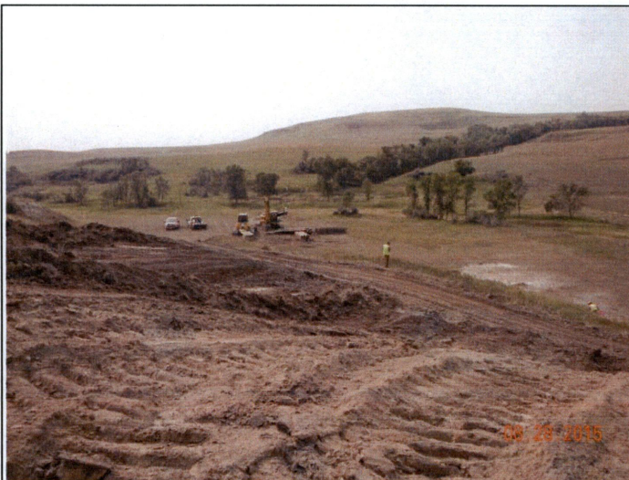
Photograph 3: Viewing southward from near Sta. 110+00 (MP 2.1) across Wetlands 1 and 2 at ongoing work to begin installation of travel lane through Wetland 2.
