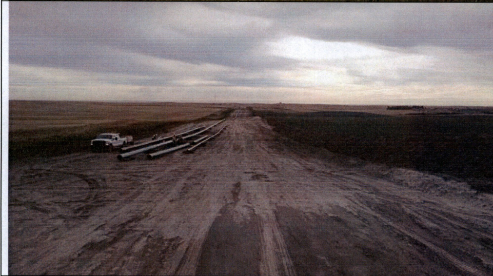
Photo 8: Looking east at east-west portion of pipe line ROW in Section 31. 18-inch Cherry Creek Line (green) is assembled. Portions of Cherry Creek and NGL to be bored under 138 th Ave NW are also shown.
