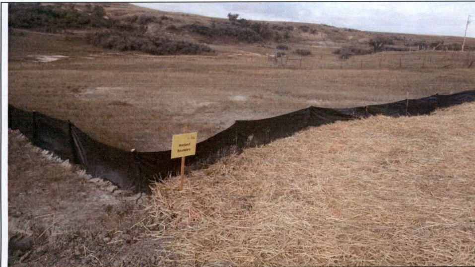
Photo 10: Looking southwest at silt fence and mulch upstream of Wetland 01 in Section 6.
