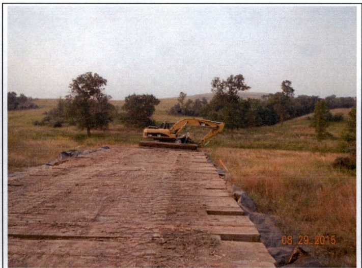
Photograph 4: Viewing southward from Sta. ~118+00 (MP 2.2) at the installation of a travel lane through Wetland 2.
