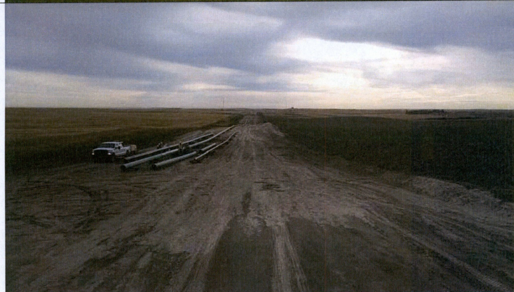
Photo 8: Looking east at east-west portion of pipe line ROW in Section 31. 18-inch Cherry Creek Line (green) is assembled. Portions of Cherry Creek and NGL to be bored under 138 th Ave NW are also shown.
