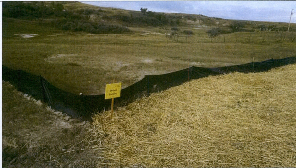
Photo 10: Looking southwest at silt fence and mulch upstream of Wetland 01 in Section 6.
