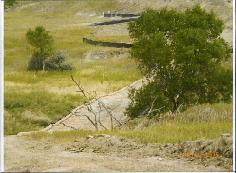
Photograph 6: Viewing southward from Sta. 121+50, (MP 2.3) viewing the completed travel lane between the trees with no impacts to woody vegetation. Wetlands 2 and 1 are in the background.
