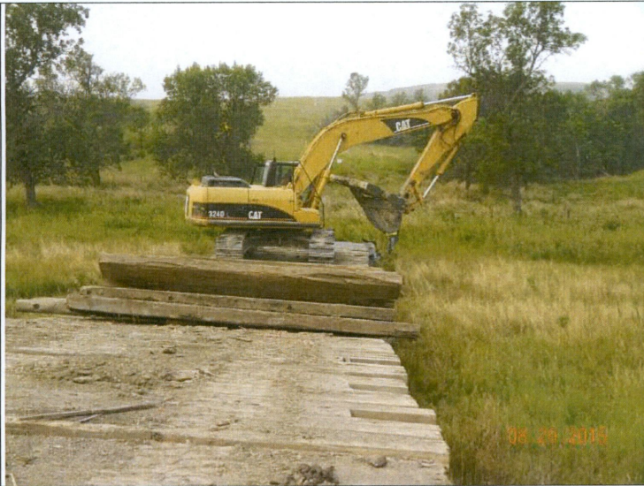
Photograph 5: (Close up view of Photograph 5) Viewing southward from Sta. ~118+00 (MP 2.2) at the installation of a travel lane through Wetland 2
