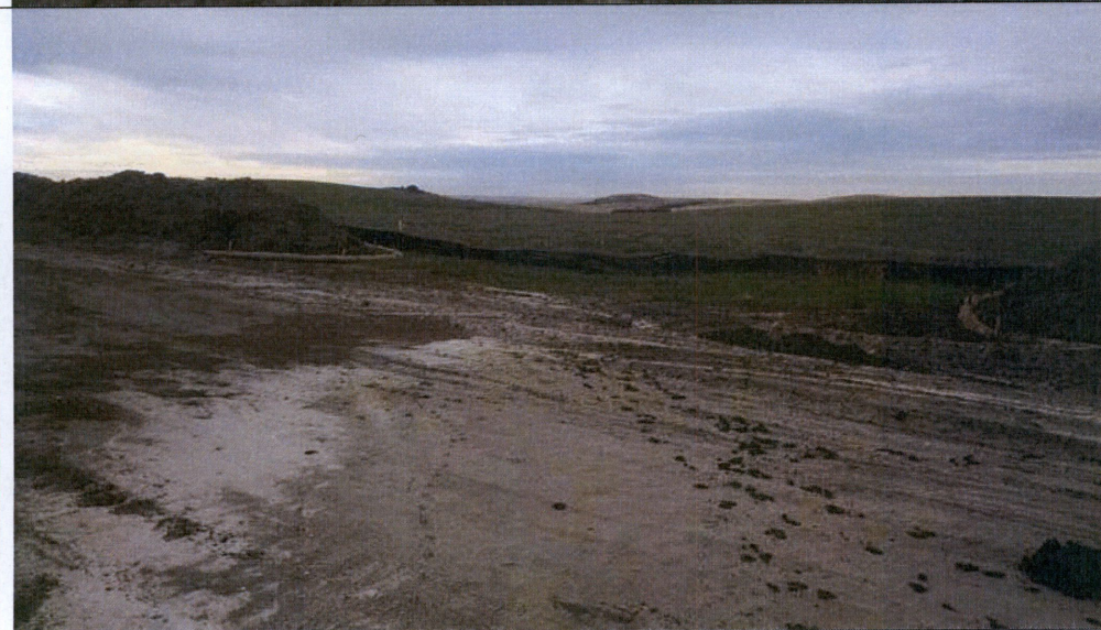
Photo 9: Looking south in Section 31 at erosion control at a drainage swale along the ROW.
