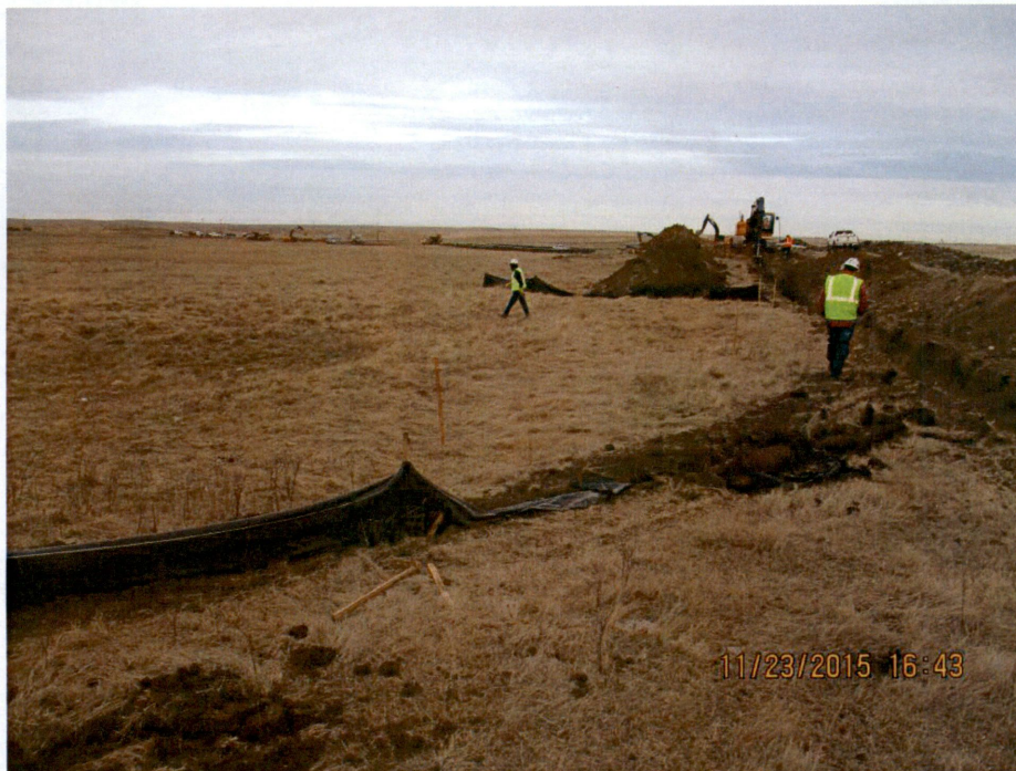
Figure 70. Photo of ditch construction along wetland boundary and silt fencing damaged. The Tomahawk maintenance crew was notified to repair the fence.
