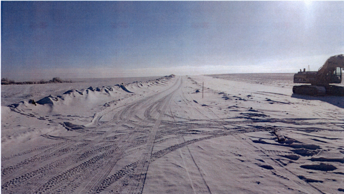
Figure 8. View of the travel route onto a construction site, the topsoil pile that is laid off to the side, and construction equipment that are all entirely found within the 100-ft wide ROW.
