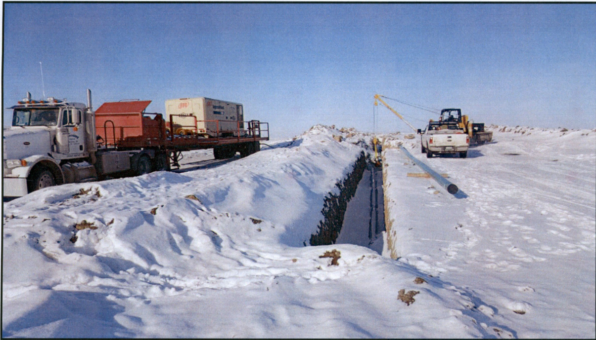
Figure 5. Open trench and compressor tank on the back of the truck where the pipeline inspection for the “pigging” process was being done.
