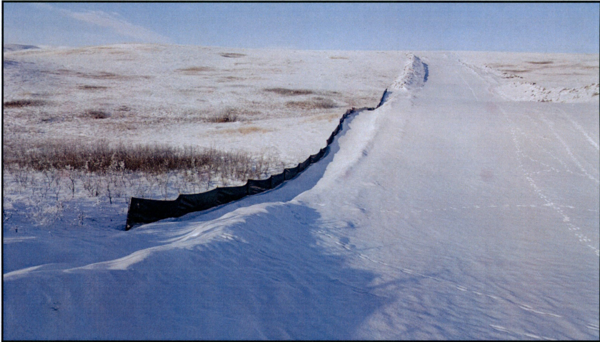
Figure 7. Silt fencing around the construction area to prevent soils from eroding off the ROW during the initial ground breaking activities and during spring snowmelt.
