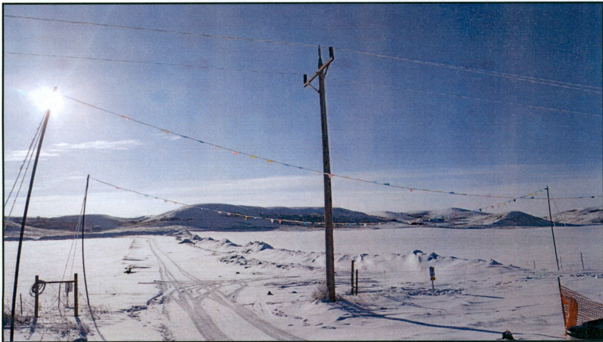
Figure 2. Overhead protection in place while working around the powerlines and preparing to bore under the road. Wooden matting was also installed for easier access onto the site.
