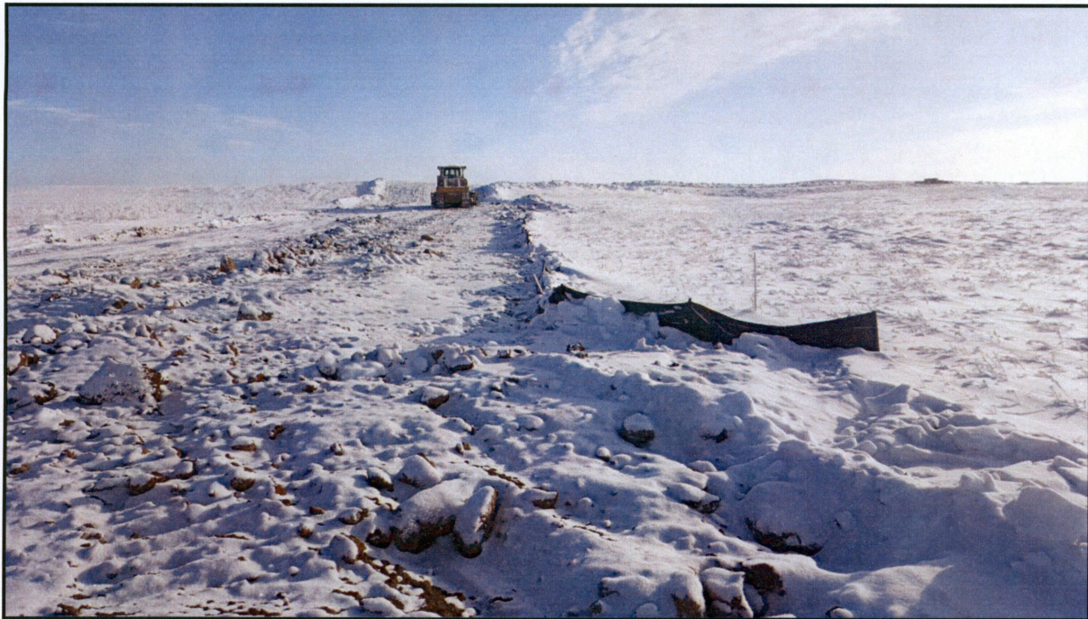
Figure 6. Installed silt fence that is in place separating the construction ROW from a small wetland. The silt fence is partially buried to prevent any soil from escaping underneath the silt fence into the wetland.
