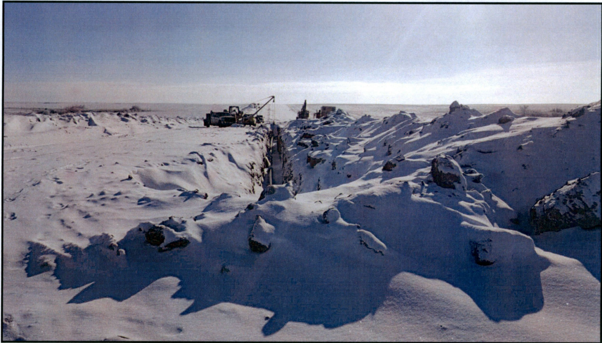
Figure 3. Beginning location for the pipeline's "pigging" process. The pipeline was pressurized and the "pig" was being sent north to the very end of the pipeline. Proper indicators and safety practices were in place.
