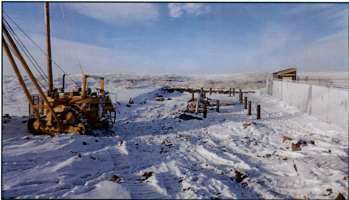
Figure 4. The northern end of the pipeline where the tie-in is located into the already existing Vantage pipeline. Also where the "pig" was being directed to for the pipeline's quality inspection. A monitor observing the process is always present.
