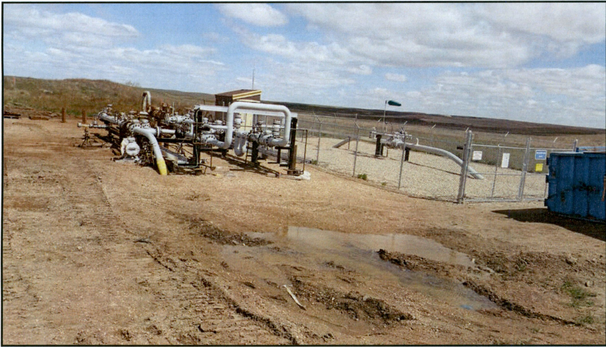
Figure 1. Photo taken from the ROW looking north at the final valve connection to the existing ONEOK Pipeline. Connecting "T" is scheduled to be installed on June 23 rd , 2016.
