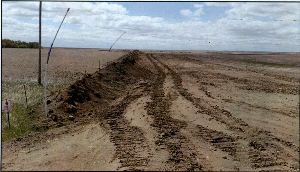
Figure 3. Photo taken facing south across Section 32, T160N, R101W from 85 th Street NW. Overhead electrical line flagging is in place. Topsoil is waiting to be replaced.
