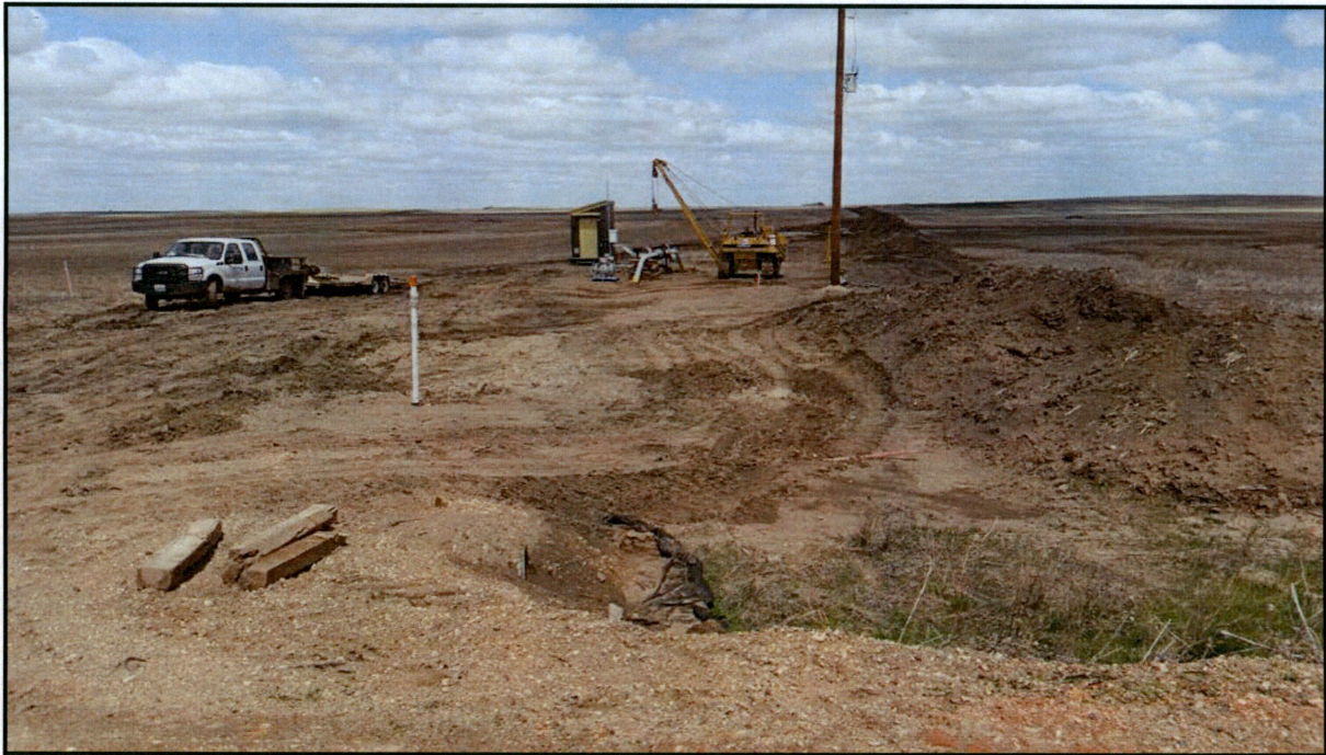
Figure 8. View looking north from 76 th Street NW at block valve 2.
