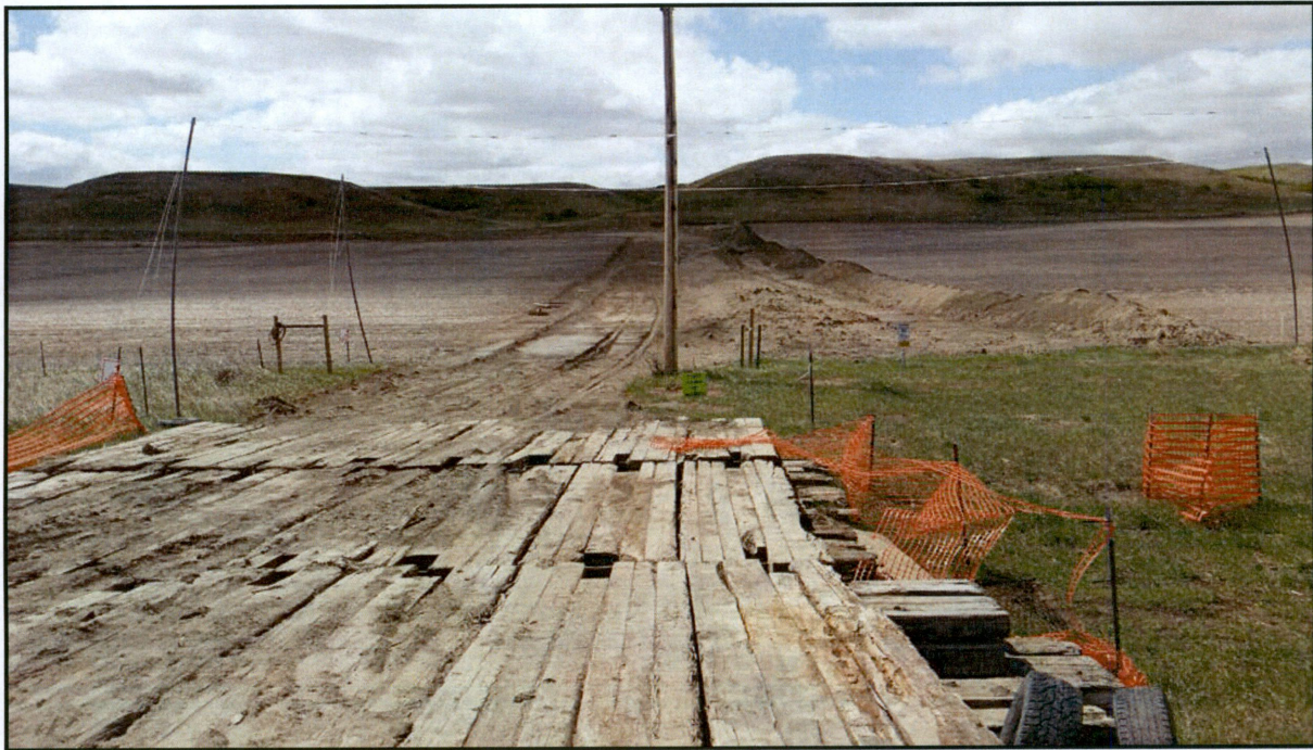
Figure 5. Photo looking south from crossing of Highway 50. Overhead electrical line flagging is in place. Topsoil has not been spread.
