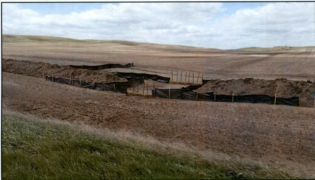
Figure 6. Installed silt fence and straw bales that are correctly placed and functioning. The silt fence is partially buried to prevent any soil from escaping underneath the silt fence and off the ROW.
