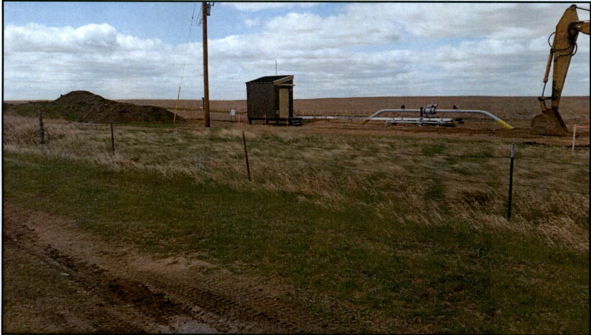
Figure 4. Photo of block valve 3 in Section 12, T159N, R102W.
