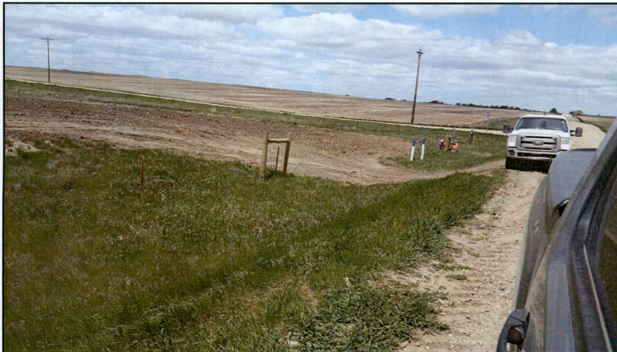
Figure 10. Photograph taken facing north from 147th Avenue NW. Fencing crews are replacing fence disturbed by the pipeline.
