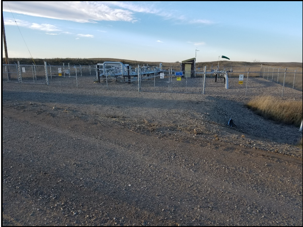
Figure 2. View looking north at the main-line block valve in Section 21, T161N, R100W.
