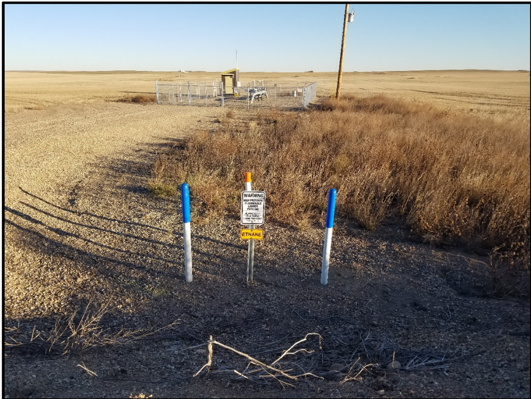
Figure 9. View looking north at the above ground valve station ins Section 11, T158N, R102W. Canada thistle was noted at this location.
