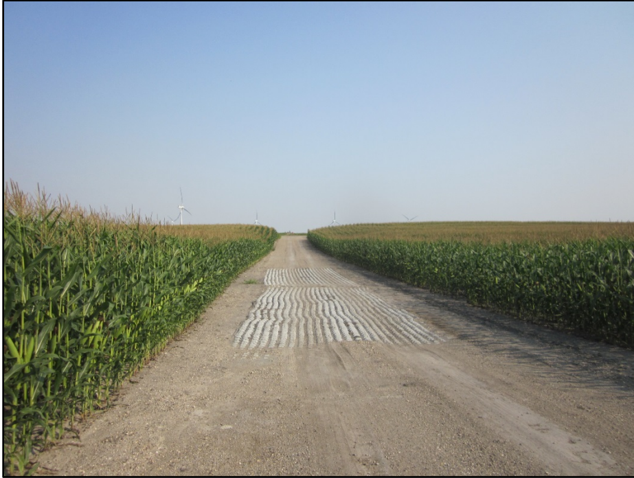
Photo 5. (GPS Point #550) – View of low water crossing that was installed on an access road. The concrete is approximately 6-inch depth to help stabilize the road. Direction: North.
