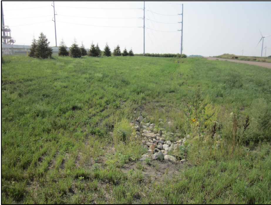
Photo 9. (GPS Point #552) – Courtenay Wind Farm Substation to the left of photo. Culvert with rocks were installed, no sedimentation or erosion were observed. This area had previously been washed out but has been reclaimed. Direction: Southeast.
