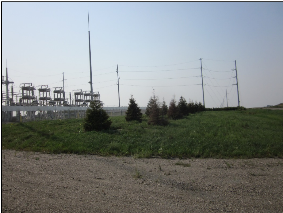
Photo 10. (GPS Point #552) – Courtenay Wind Farm Substation to the left of photo. Trees were planted near fenced area. Trees were to be planted in front of the substation to help screen the view of the substation as per an agreement with a landowner. A few of the trees appear to be dying. Direction: Southeast.
