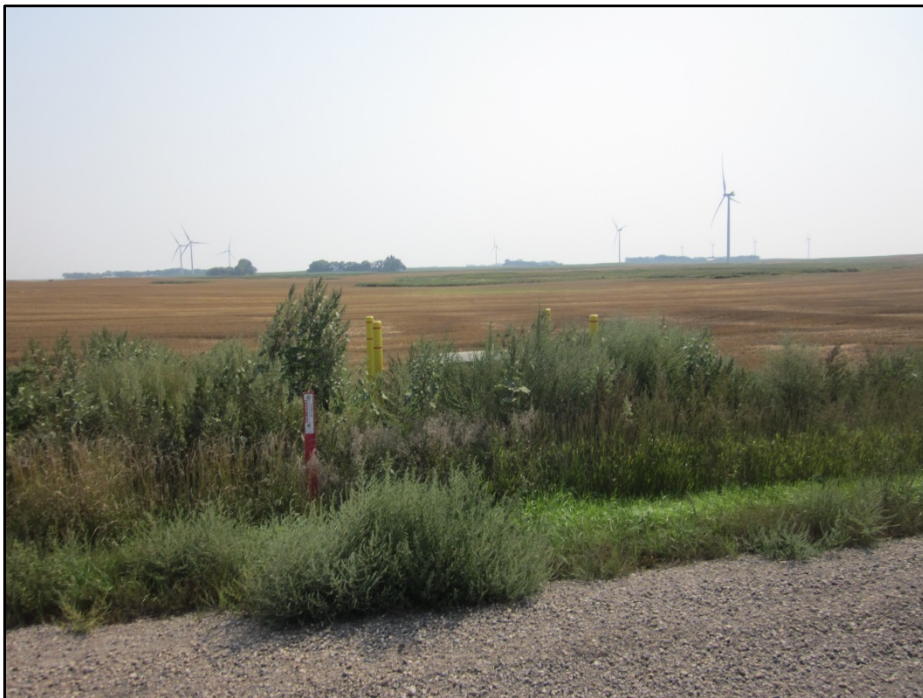
Photo 12. (GPS Point #553) – Underground line marker by road. Lines connect to substation. Junction box has cement bollards surrounding it. Annual weeds should be sprayed or mowed to keep junction box clearly visible. Direction: East.
