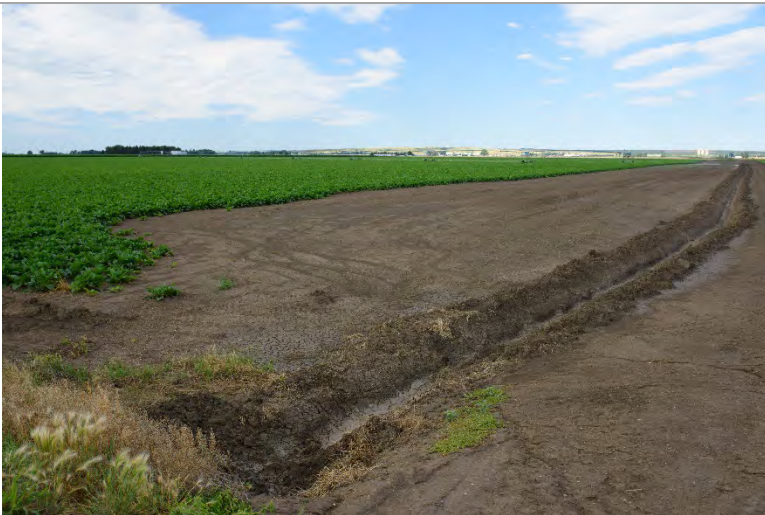
Photo 6: Reclamation (facing Southwest). Irrigation trench dug by landowner after landowner accepted reclamation of pipeline construction.
