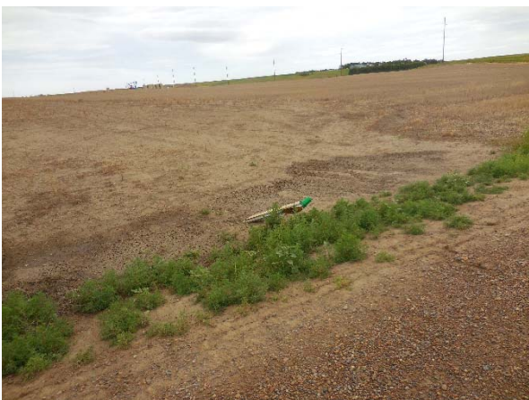
Photo 24: Pipeline signage in need of repair. At 154 th Avenue NW, facing east.
