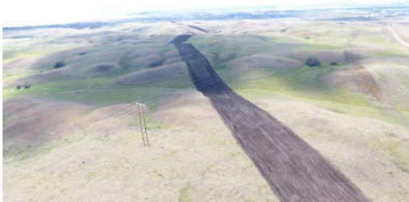
Picture 65: Station 1824+50.00; Latitude: 47°59'54.30"N Longitude: 102°26'16.88"W Looking south, pipeline to the right of recent reclamation
