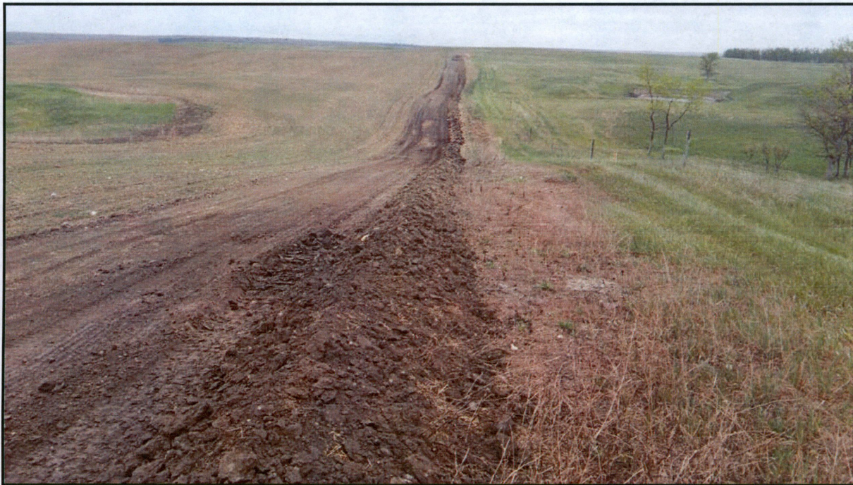
Figure 6. Photo taken looking west down the access road to Turbine B-9. Topsoil has been stripped and stored on the north side of road.
