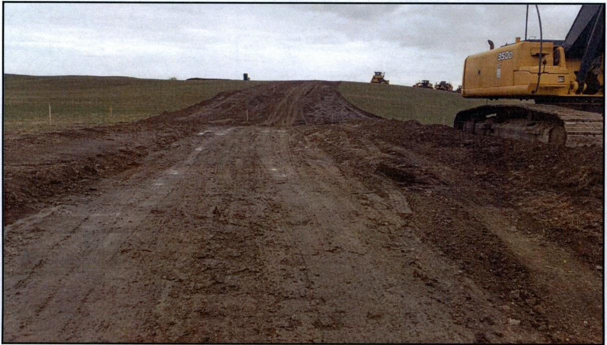
Figure 3. Photo taken facing north from 72 nd St. NW. Topsoil was stripped and stored for the access road to Turbine B-10. ROW markers were in place. Due to rain, a shallow layer of topsoil had been re-spread to protect subsoil.
