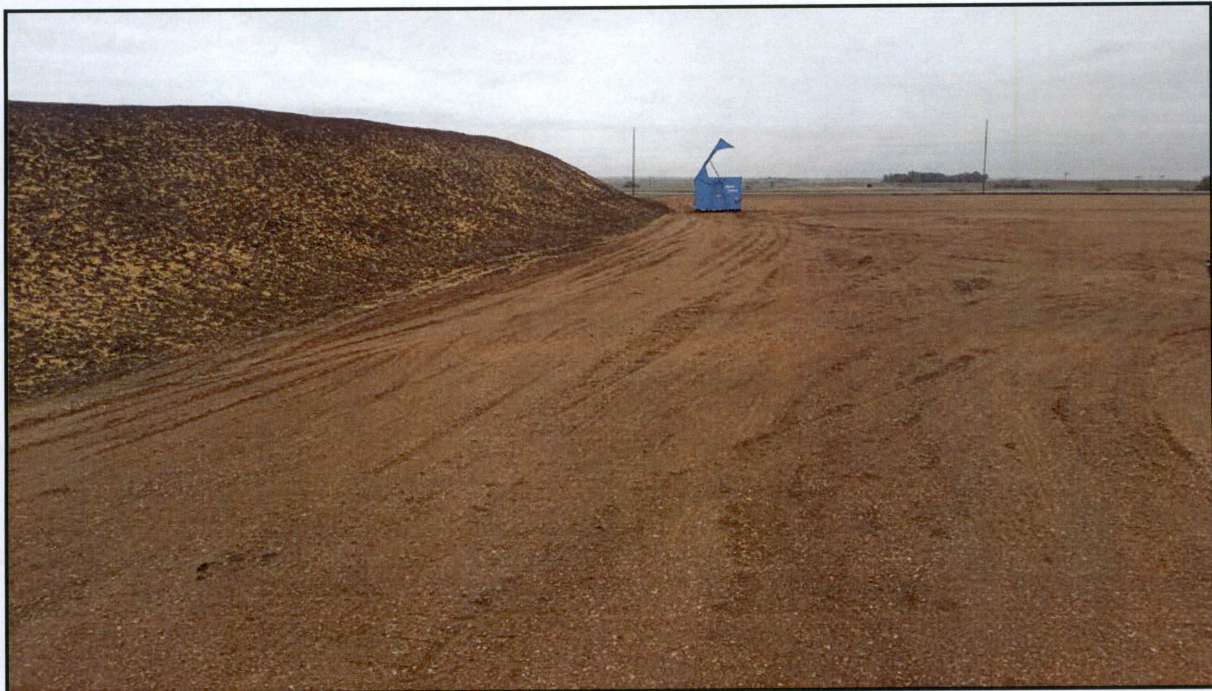
Figure 1. Photo taken facing east from the northwest corner of the lay down yard. Segregated topsoil and surfaced yard can be seen.
