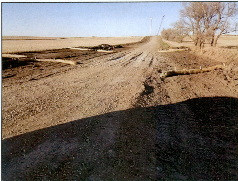
Figure 11. Photo taken along access road, north of turbine F8. Additional rock placed in road for a high-water crossing and straw waddles in place for erosion control.
