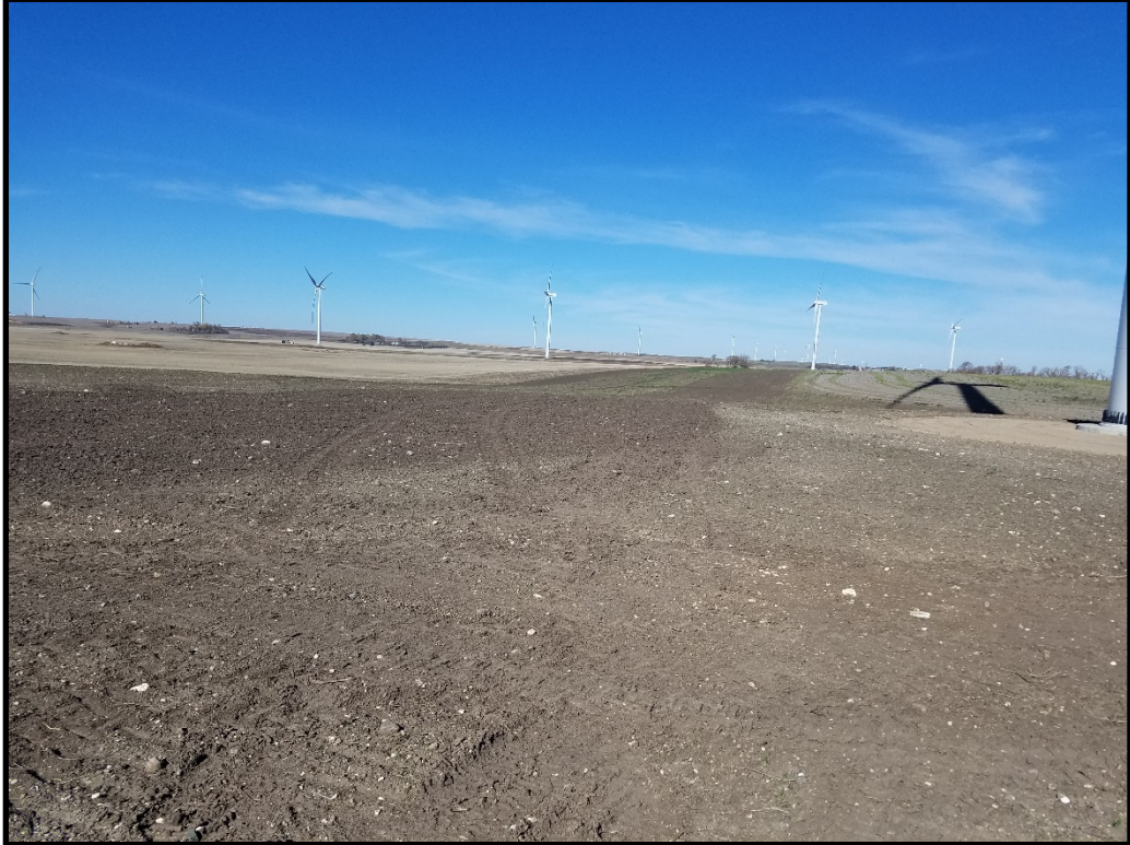
Photograph 5. View looking north at the reclaimed underground collection line / crane path in the SW1/4 of Section 17, T158N, R95W.
