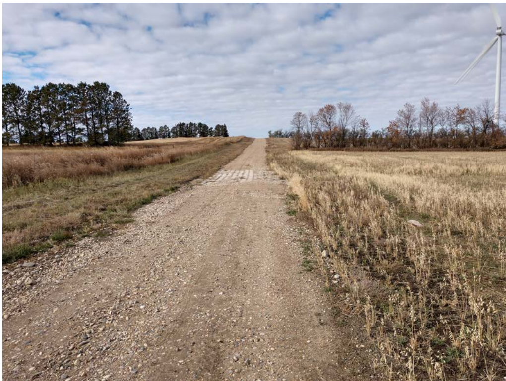
Photo 2. Photo of revetment mat at low water crossing on access road near Turbine D7 (looking west).
