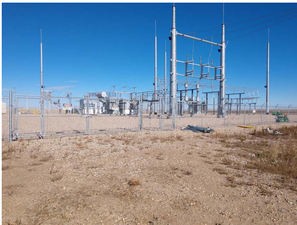
Photo 8. Photo of substation (facing northeast).
