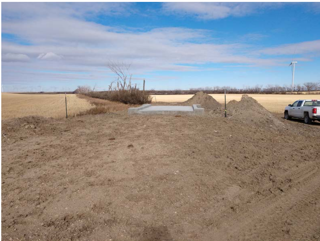
Photo 10. Photo of high-pressure gas line crossing near Turbine B4 (facing northeast).
