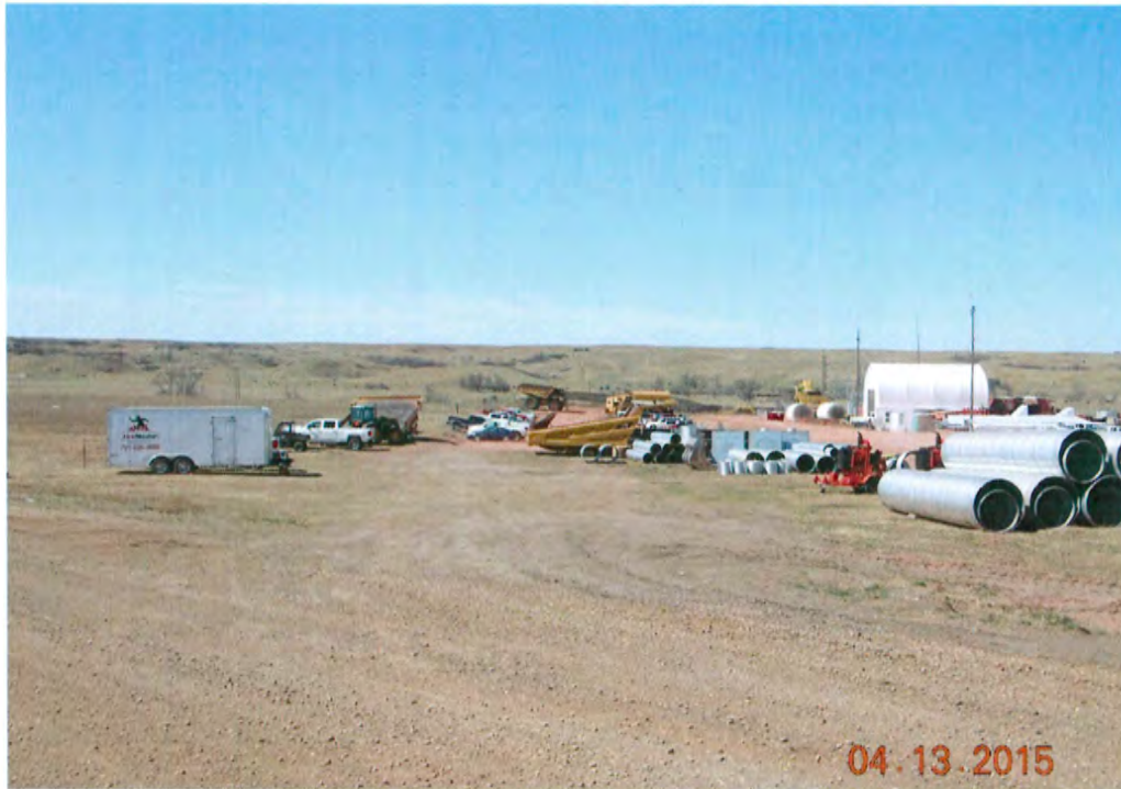
Figure 1. Area in the NE \frac{1}{4} NE \frac{1}{4} NE \frac{1}{4} of Section 31 in Permit NACC-1301 where SPGM had not been removed but is being used for contractor and equipment parking, and also for equipment and material storage - facing west with 65 \frac{1}{2} th AVE SW in foreground, and scoria capped parking in background - refer to Figure 5 for area location
