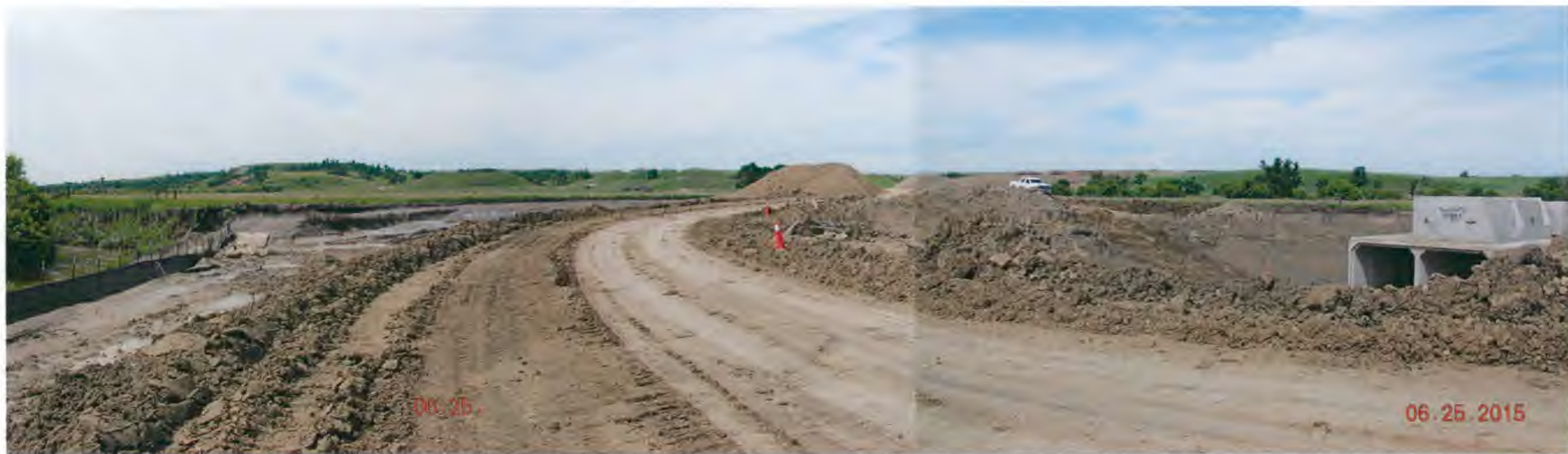
Figure 4. Box culverts on the right in relation to Coyote Creek across the Shop Access Road on the left - facing westerly.
