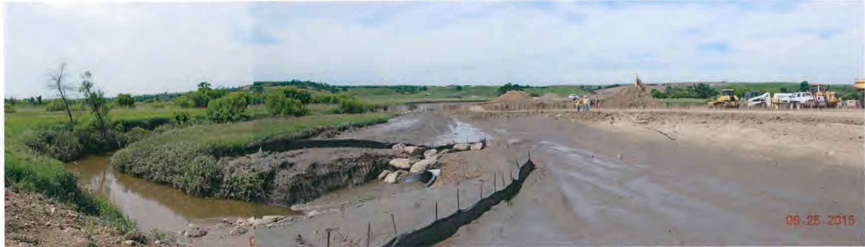
Figure 3. Coyote Creek flow into the low flow culvert - facing westerly with the Shop Access Road on the right.
