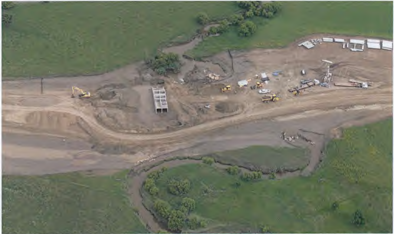
Figure 1- Coyote Creek at access road crossing site taken during June 25, 2015 flyover inspection
