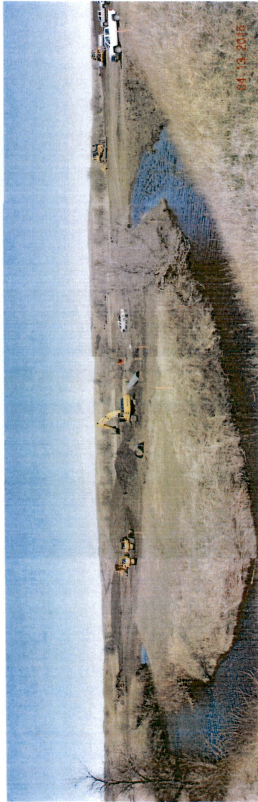
Figure 4. Panorama of 36 inch low flow steel culvert installation in Coyote Creek for the Shop Access Road Coyote Creek crossing - facing west on left and rotating to face north on right with temporary culvert in place on center-right for equipment crossing – refer to Figure 5 for culvert location – note temporary topsoil stockpile in left background and a temporary subsoil stockpile in middle background – also note that dozer was in motion when photographs were taken
