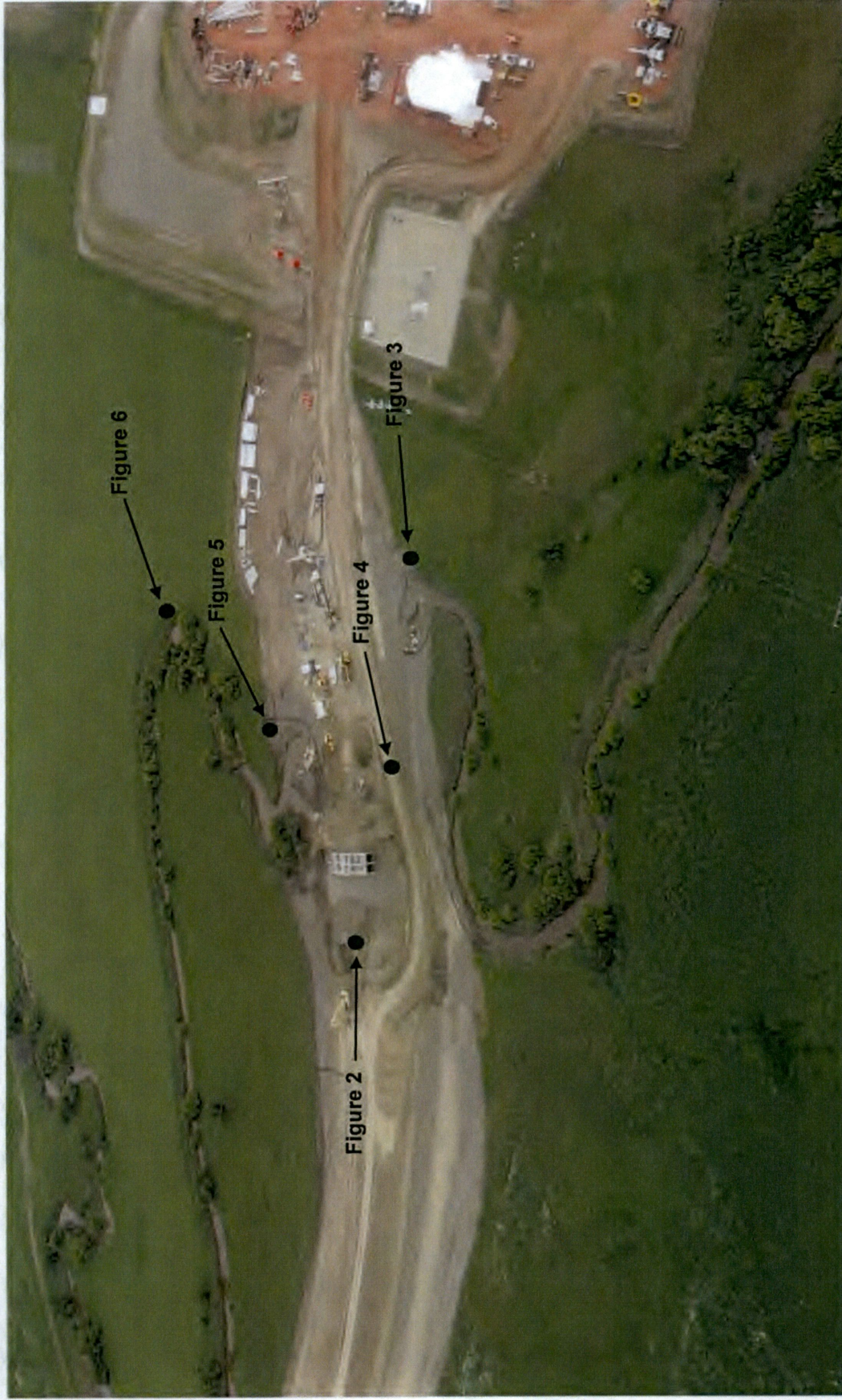
Figure 1. Ongoing box culvert installation for the Shop Access Road in Permit NACC-1302 at the Coyote Creek Mine on June 25, 2015 pictured on a 2015 mine flyover inspection aerial photograph. Points represent Figure 2 through Figure 6 photograph locations and arrows indicate general photograph direction.
