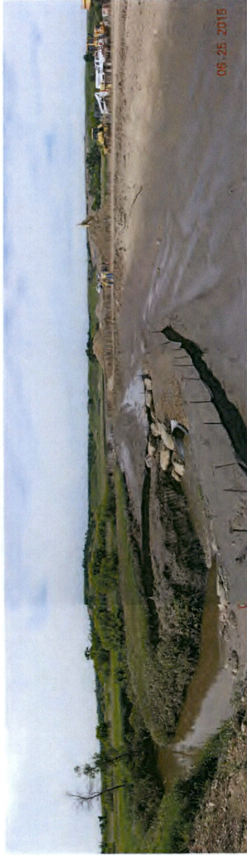
Figure 3. Coyote Creek flow into the low flow culvert - facing westerly with the Shop Access Road on the right.
