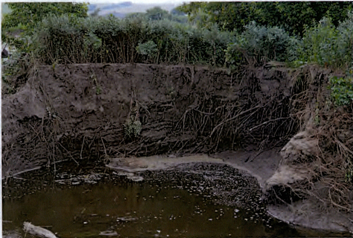
Figure 4- Closer view of bank erosion feature located across from the 60-inch culvert
