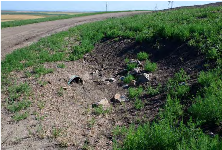
Photo 2: Between Tower 30 and 31 (facing North). Significant erosion, culvert filling with sediments (approximately 66% full)
