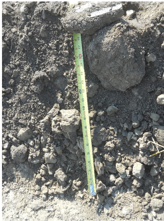
Photo 4: Located at station 108+00, photo showing depth of topsoil removal cut on Right of Way edge.
