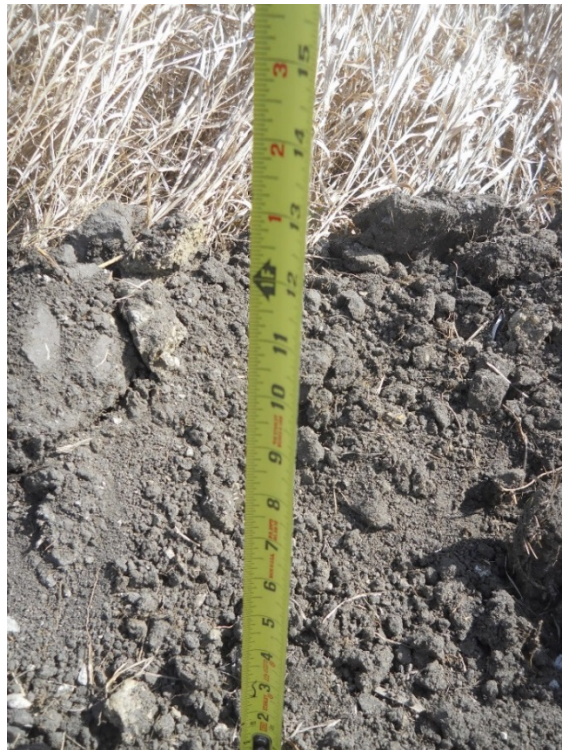
Photo 12: Located at station 48+00, photo showing depth of topsoil removal cut on Right of Way.
