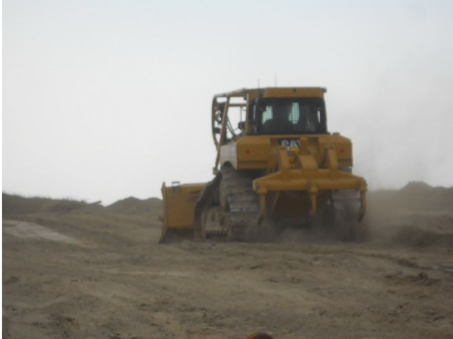
Photo 11: Located at station 40+00, looking west. Contractor ripping and stripping topsoil across Right of Way. Topsoil and subsoil are being placed at south side on Right of Way. Both topsoil and subsoil are placed far enough apart so no touching of soil types can occur.
