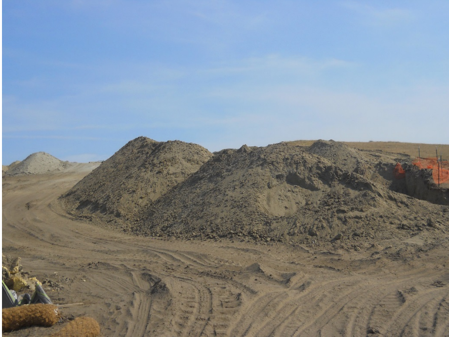
Photo 13: Located at station 52+00, looking north, showing Right of Way graded with topsoil and subsoil piles separated and placed along edges of Right of Way.
