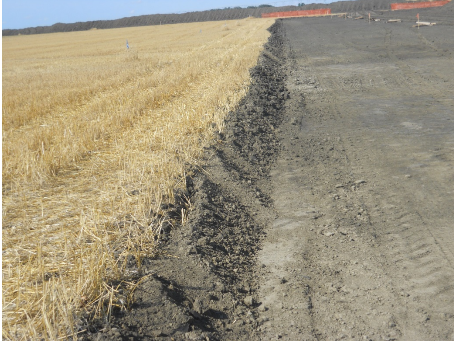
Photo 5: Located at station 110+00, looking south with graded Right of Way. Photo shows depth of topsoil cut at approximately 12 inches deep on left side along Right of Way. Topsoil pile shown on edge of Right of Way at top of photo.
