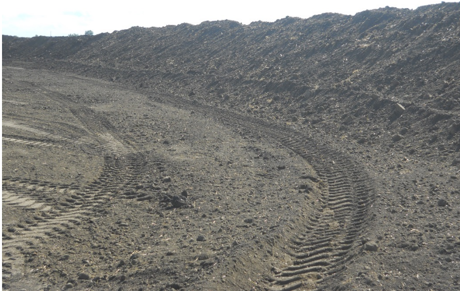
Photo 3: Located at station 105+00, looking south, photo showing Right of Way graded with topsoil pushed off on edge on Right of Way.
