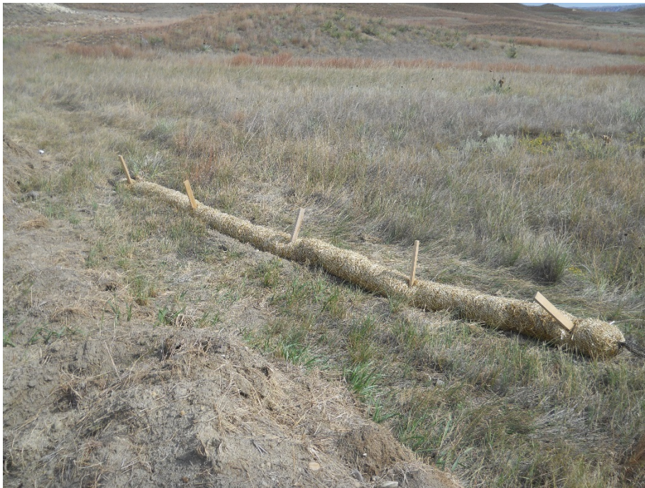
Photo 4: Located at station 18+00, showing BMP straw wattle placed along edge of Right of Way to prevent sediment runoff leaving Right of Way.
