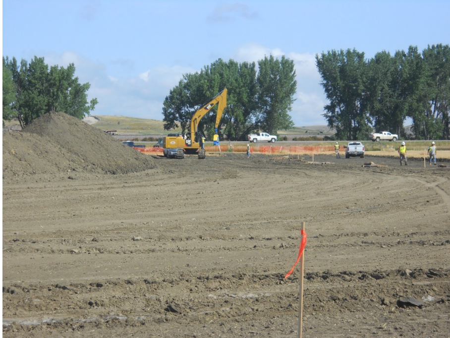
Photo 1: Located at station 98+00, looking north, photo showing workers grading Right of Way. Topsoil pile located on left side edge of Right of Way. Workers starting to bore Highway 1804 and railroad tracks, heading from south side Highway 1804.
