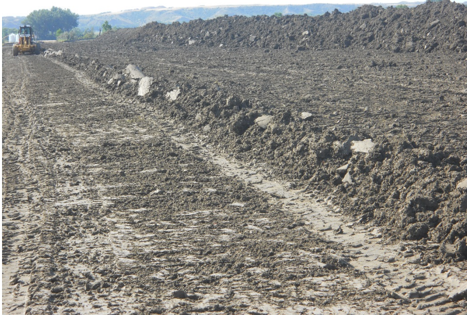
Photo 15: Located at station 91+00, showing contractor grading Right of Way looking south. Contractor pushing topsoil off Right of Way towards easement edge, located at right side of photo.
