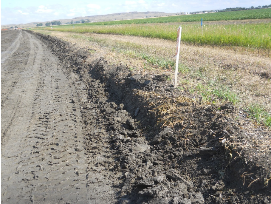
Photo 11: Located at station 127+00, looking north showing graded Right of Way with topsoil cut approximately 12 inches deep.
