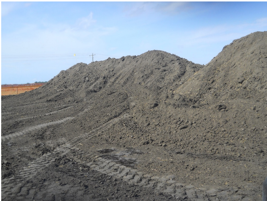
Photo 14: Located at station 72+00, photo showing graded Right of Way with topsoil pile pushed off Right of Way and piled along edge as shown.
