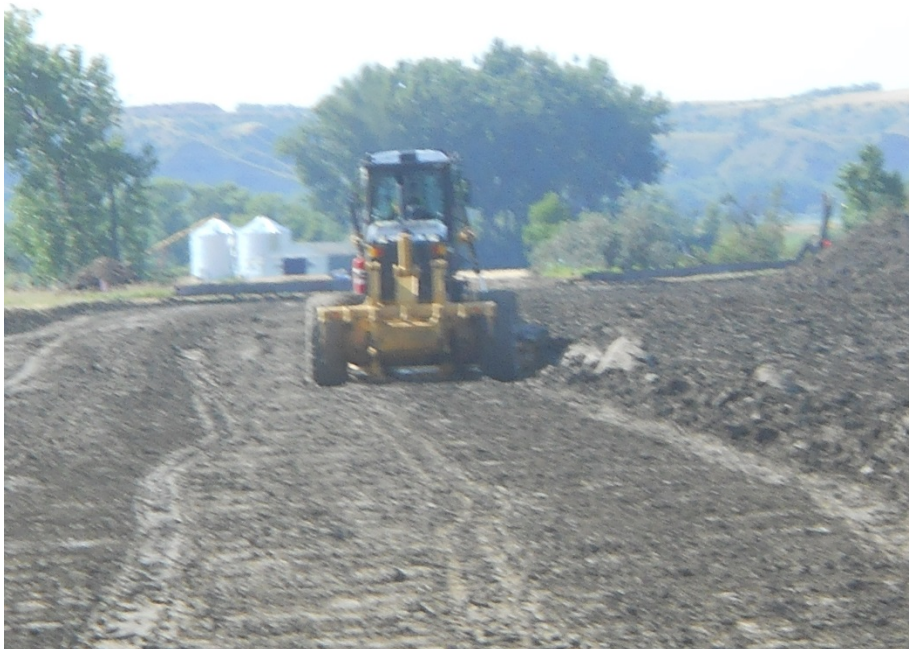
Photo 12: Located at station 130+00, looking south showing contractor grading Right of Way to PSC standards.
