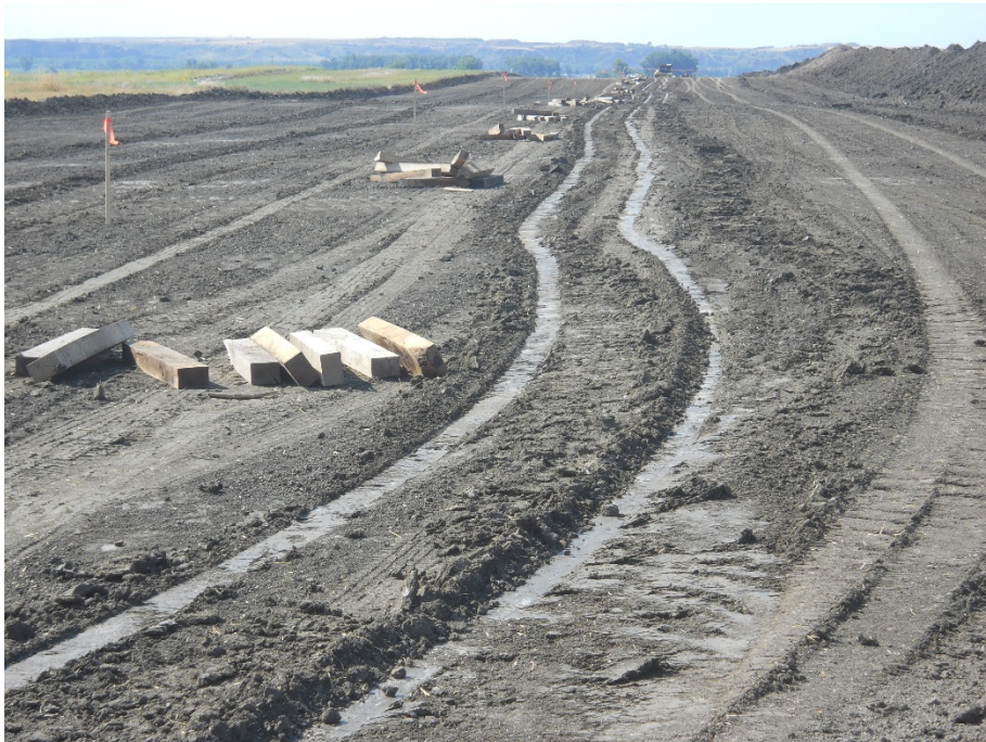
Photo 6: Located at station 113+00, looking south, showing Right of Way graded with topsoil pushed off on right side along Right of Way. Wooden skids placed on Right of Way ready for supporting piping.
