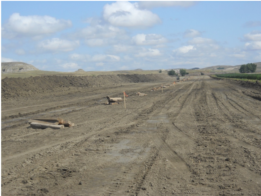
Photo 8: Located at station 30+00, photo showing graded Right of Way on north side of Highway 1804 showing depth of topsoil cut, at approximately 12 inches deep and topsoil pushed off on edge of Right of Way. Wood skids placed on Right of Way ready to string out piping.
