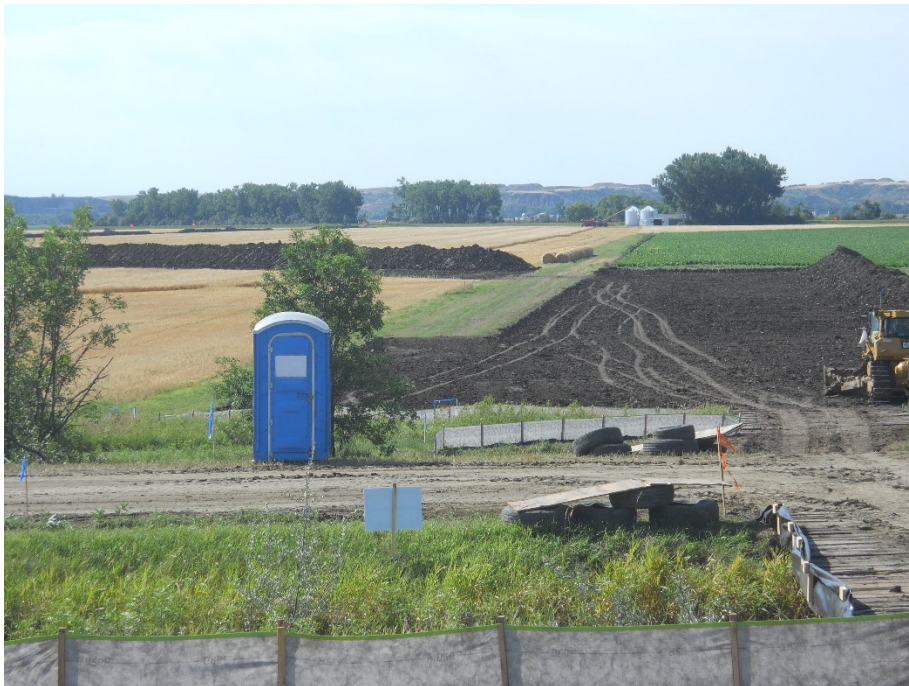
Photo 14: Located at station 140+00, showing graded Right of Way located at re-route south tie-in bench valve location. Right of Way is graded with topsoil push off on edge of Right of Way, as noted from photo. Silt fence BMP installed along Right of Way as required.
