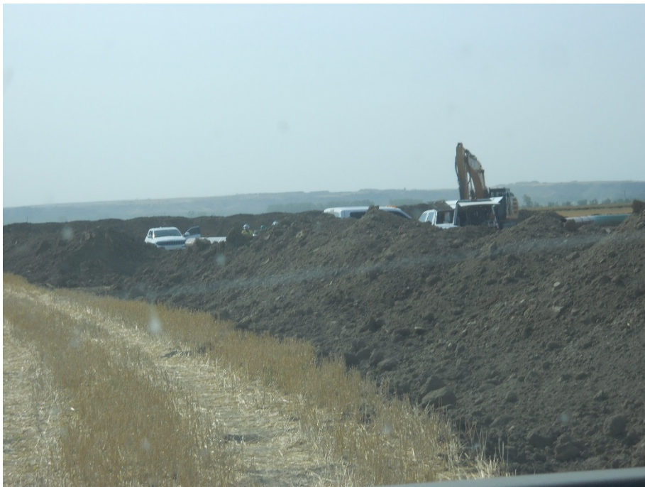
Photo 10: Located at station 36+00, photo looking south showing contractor grading Right of Way with topsoil placed along edge of Right of Way.
