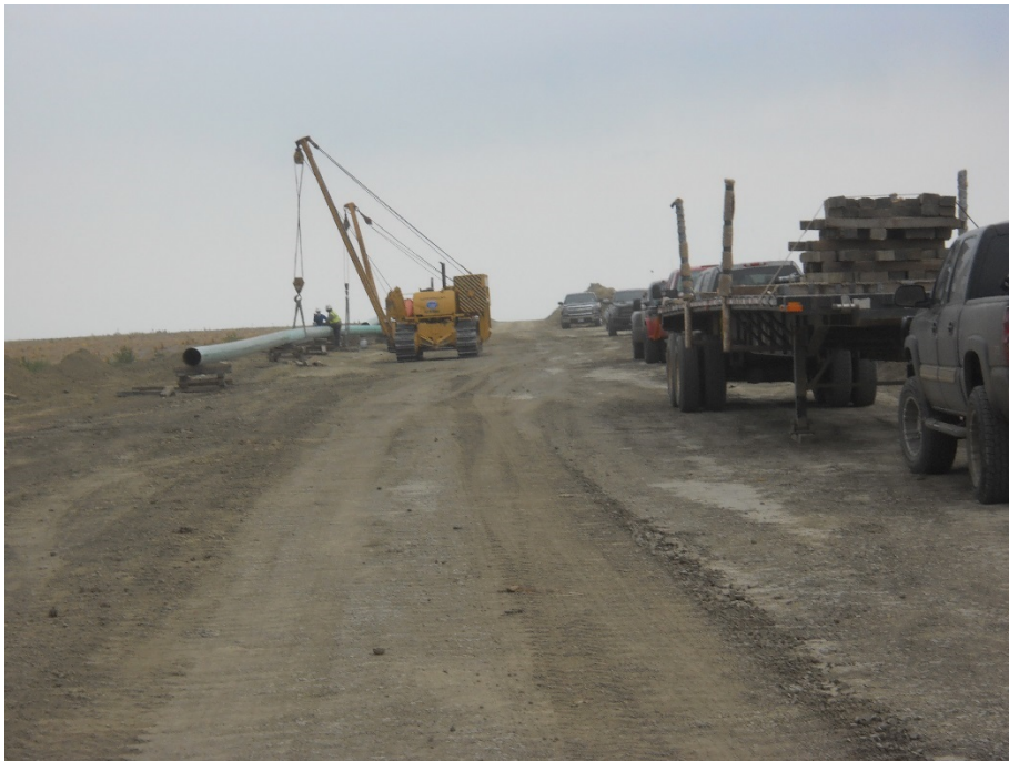
Photo 6: Located at station 24+00, looking west with topsoil stripped across Right of Way. Workers stringing pipe and welding pipe together.
