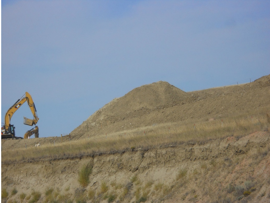
Photo 5: Located at station 21+00, photo showing Right of Way on north side of Highway 1804. Contractor working on Right of Way placing topsoil and subsoil piles along edge of Right of Way. Both soil types are separated and not touching.
