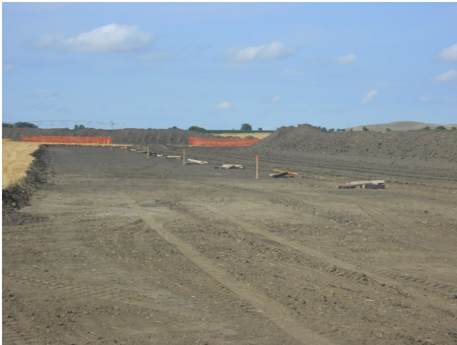
Photo 2: Located at station 102+00, looking south, photo showing graded Right of Way with topsoil pile placed on edge of Right of Way. Wood skids placed on Right of Way ready to support piping.
