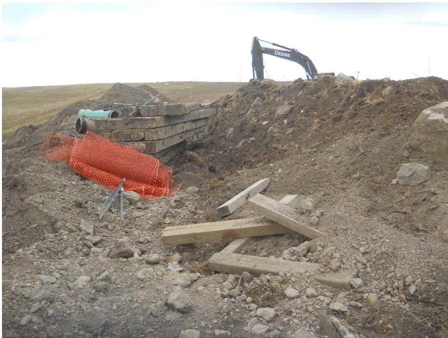
Photo 10: Located at station 126+00, looking south of graded Right of Way. Photo showing matts placed over Right of Way for access along easement. Topsoil pile has been pushed off edge of Right of Way as noted.
