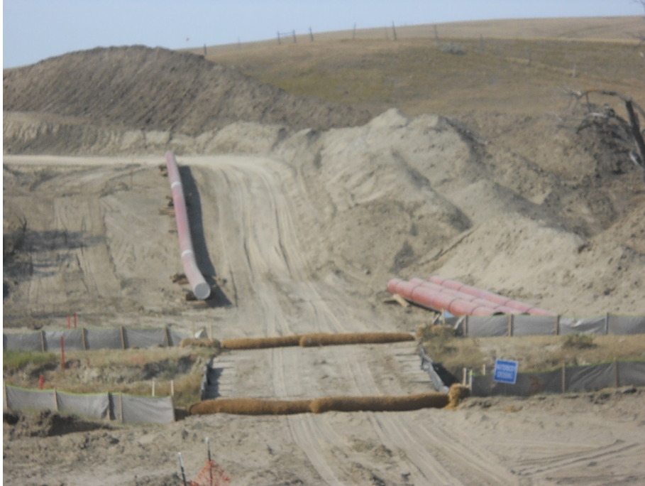
Photo 3: Located at station 15+00, photo looking west at Right of Way located on north side of Highway 1804. Right of Way has been graded with topsoil and subsoil piles separated and not touching along Right of Way edge. Photo shows BMP's, silt fences and straw wattles across Right of Way creek bed so sediment is contained on Right of Way.
