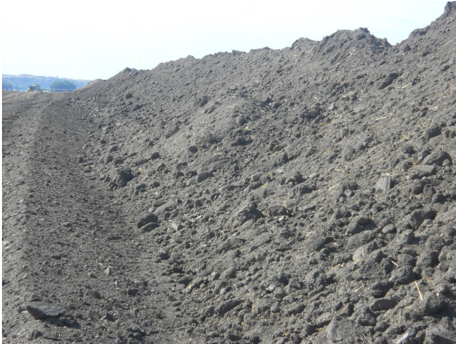
Photo 7: Located at station 115+00, photo showing graded Right of Way with topsoil pile pushed off edge of Right of Way, located on right side.
