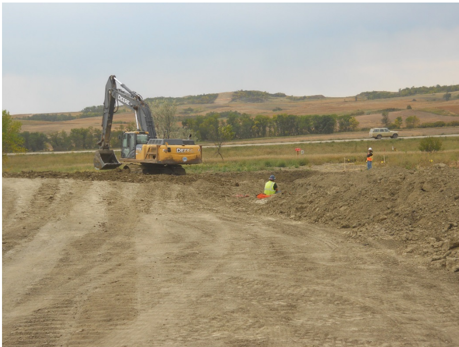
Photo 2: Located at station 6+00, Photo looking west showing Right of Way graded with topsoil pushed off on edge of Right of Way. Construction workers working on pit for Block Valve tie-in valve.
