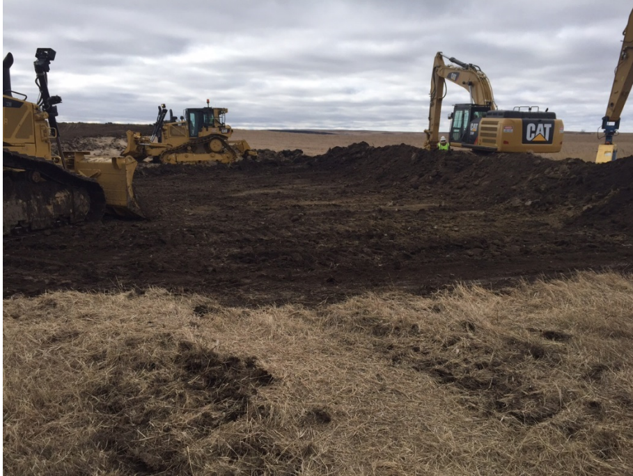
Photo 7: Located at station 27+00, photo looking west showing contractor starting to clear topsoil across Right of Way.
