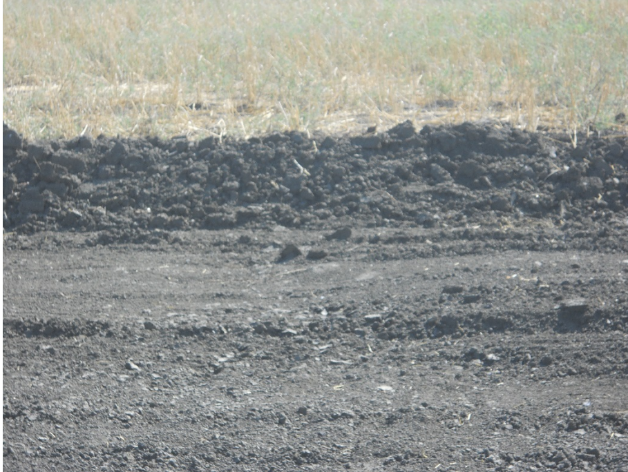
Photo 9: Located at station 122+00, photo looking south showing graded Right of Way topsoil cut approximately 12 inches deep.
