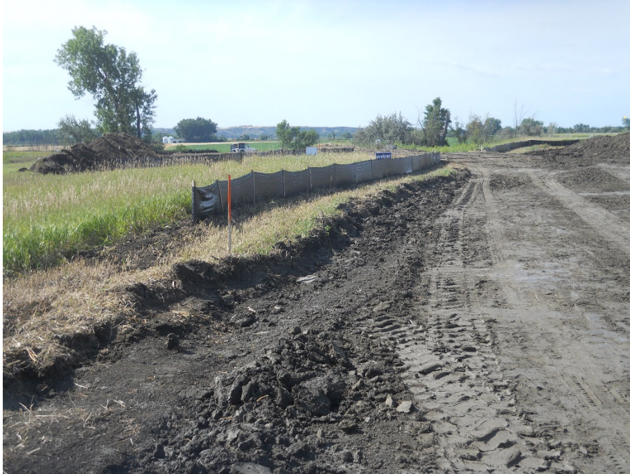
Photo 13: Located at station 134+00, photo looking west showing graded Right of Way and approximately 12" deep topsoil cut along left edge Right of Way. Topsoil placed along right side edge of Right of Way. Silt fence BMP in place along Right of Way.
