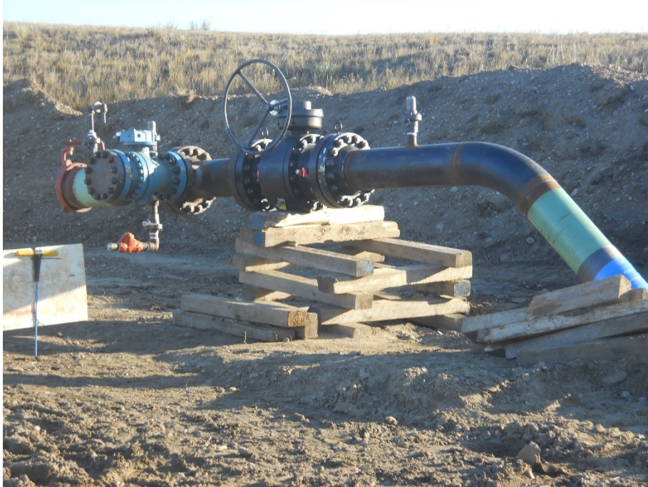
Photo 1: Located at station 0+00, showing Side Hill Junction Block Valve tie-in at end of line for Highway 1804 Re-Route North Right of Way Pipeline Project.
