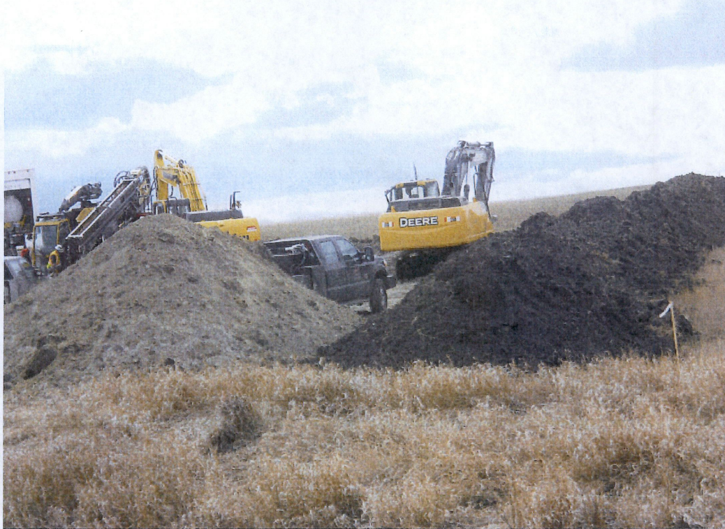
Above: Photo 33- Photo taken at bore exit 158+72.8 located on west side of county road 77 th Ave. NEW. Bore contractor on site working. Bore site was stripped of top soil and placed on west edge of site. Subsoil dug out for bell pits was deposited and mixed with top soil. Top soil should have been moved further from subsoil deposit.
