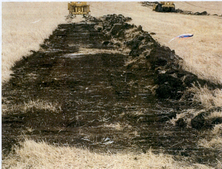
Below: Photo 6- located at bore exit 111+42.20. South side of Highway 2 looking south. Start of ripping and top soil removal on right of way.
