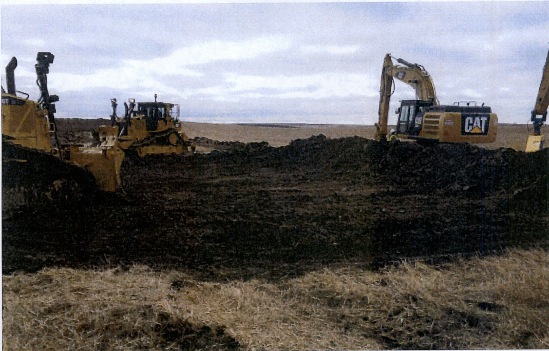
Above: Photo 7- Located at bore exit 111+42.20.South side of Highway 2 looking west. Start of ripping and top soil removal on right of way.
