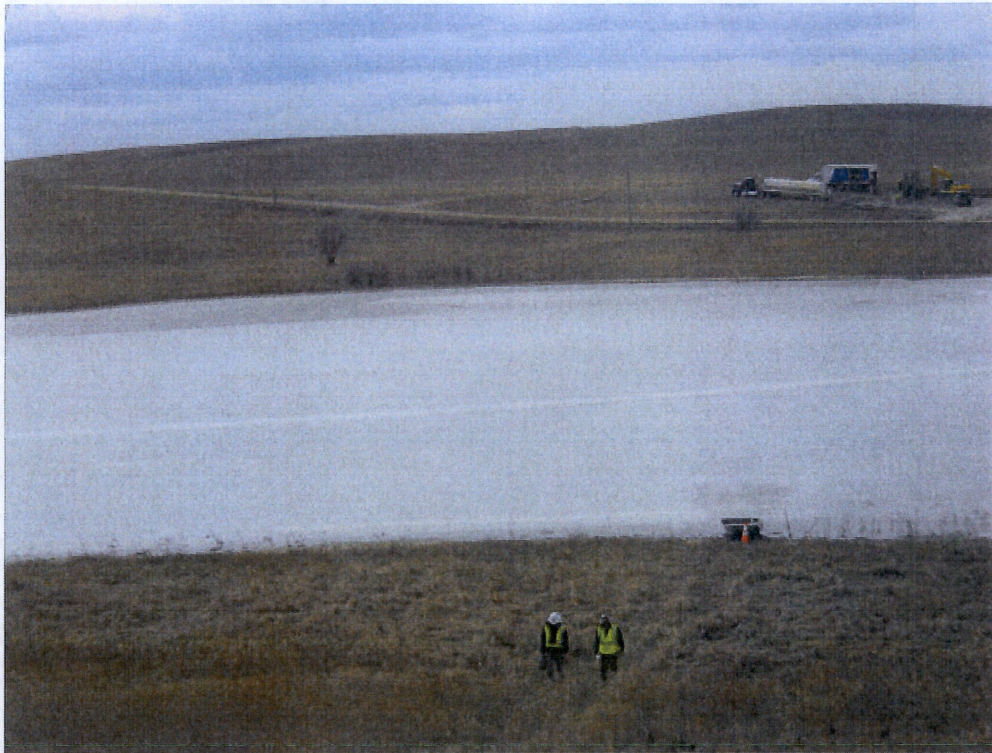
Above: Photo 31- Standing on west hillside at bore entry station 142+57.7 looking across waterway slough to be bored due to nesting habitat. Bore contractor on site working.
