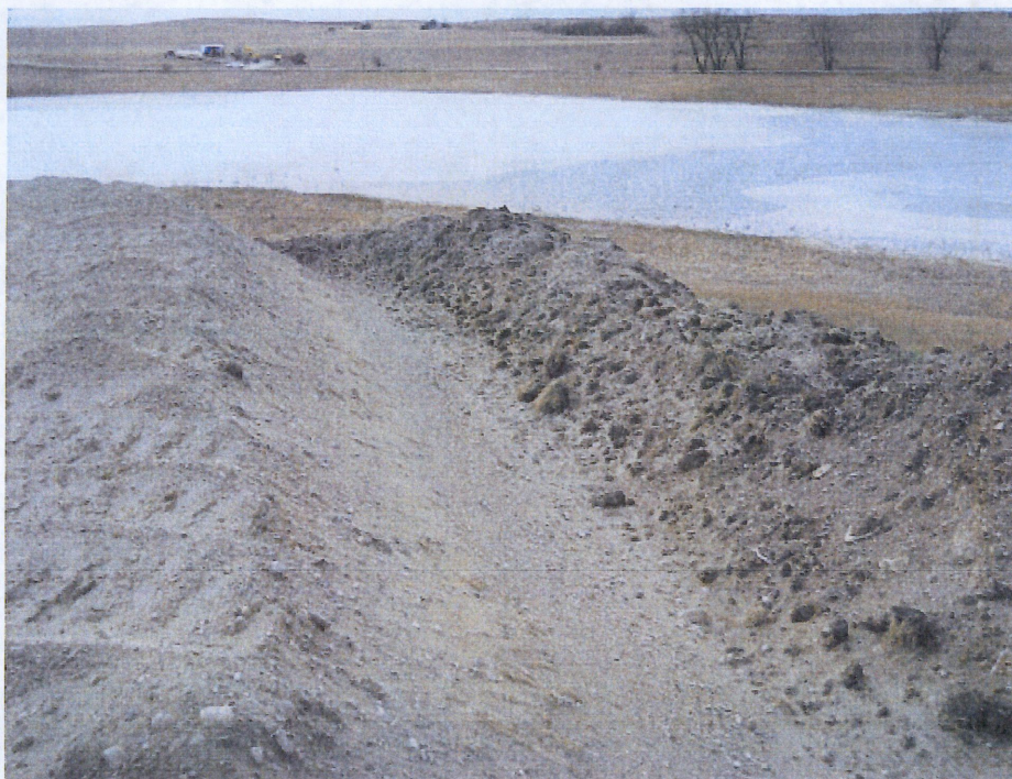
Below: Photo 30- Looking west for bore entry station 142+57.7 looking across water way slough. Top soil is placed at north side of right of way to left side of photo with subsoil ridge at left side of photo. Both subsoil and top soil appear to be mixed together. Bore contractor is shown beyond at bore exit station 156+72.8 across county road 77 th Ave. NW.
