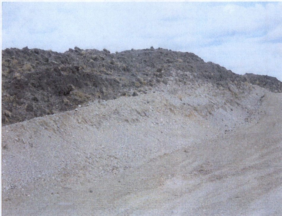
Below: Photo 28- Looking at north side of right of way at station 145+00. Photo shows graded right of way with top soil shown at top of photo. Lighter subsoil is deposited up against top soil, mixing both together.
