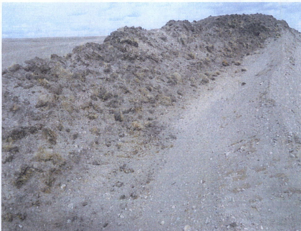
Above: Photo 29- Showing topsoil deposited at north side of right of way west end, looking back east. Subsoil ridge is shown placed up against top soil mixing both together.
