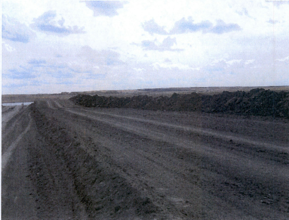
Above: Photo 15- Looking south at stopped right of way through hillside showing subsoil location lower left side of photo. Top soil placed at edge of right of way on west side easement. Station location 126+00.
