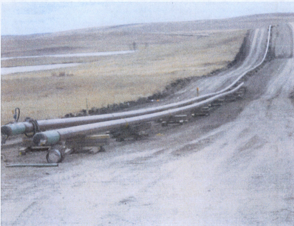
Below: Photo 22- Looking west from east end at graded right of way. Right of way has top soil depth of 12". Top soil is pushed off right of way located at right hand side of photo. Top soil not shown on photo. 12" bore piping shown on skids being hydro tested. Station location 130+00.
