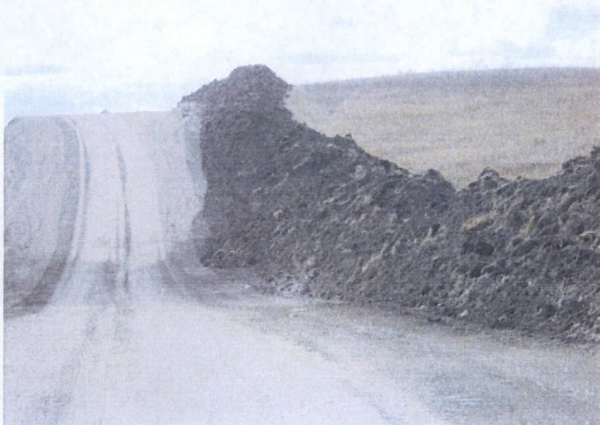
Below: Photo 24- Photo taken from east end of right of way facing west, heading uphill at station 134+00. Right of way graded with top soil pushed to north edge of right of way easement. No BMP's have been installed along entire length of right of way for erosion control.
