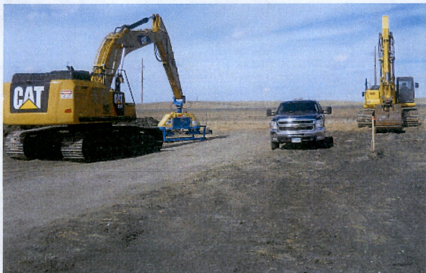
Below: Photo 2- Station 111+42.20 bore exit on south side of Highway 2 showing stripped right of way extending south with construction equipment on the side.
