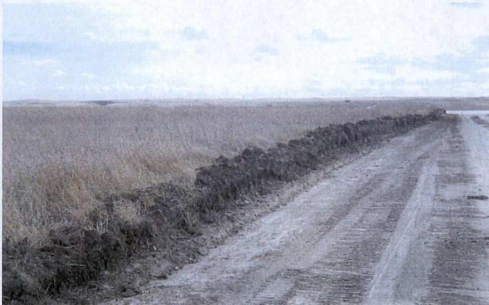
Below: Photo 10- Looking south at station 118+00 showing stripped right of way at approximate top soil depth of 12'. Photo is showing east side of right of way. Upper right hand side of photo is location of water resting habitat to be bored.
