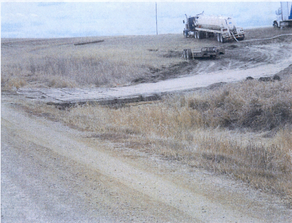
Below: Photo 32- Photo taken from county road 77 th Ave. NW. shown bridge mats in road ditch for contractor at bore exit 158+72.8.
