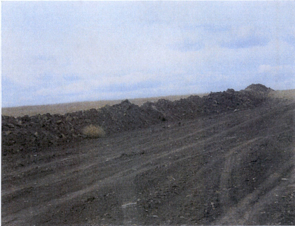
Above: Photo 21- Photo taken from east end right of way heading west towards left side of photo at station 132+00. Right of way graded with top soil pushed to north edge of right of way easement.
