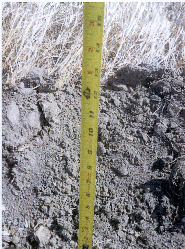
Above: Photo 7- Photo showing depth of approximately 12" top soil after right of way has been stripped. Station location is 114+00.
