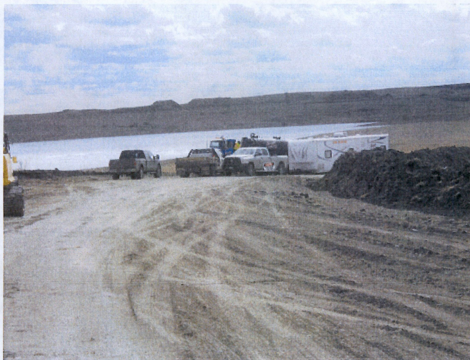
Below: Photo 20- Looking south at PI station 128+43.8 where right of way turns right and heads west. Photo shows contractor on site hydro testing bore piping. Pipe not showing in this photo.
