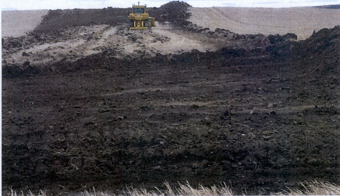
Above: Photo 9- Located at station 122+00 looking south. Top soil being ripped and stripped. Top soil being placed at west side on right of way.
