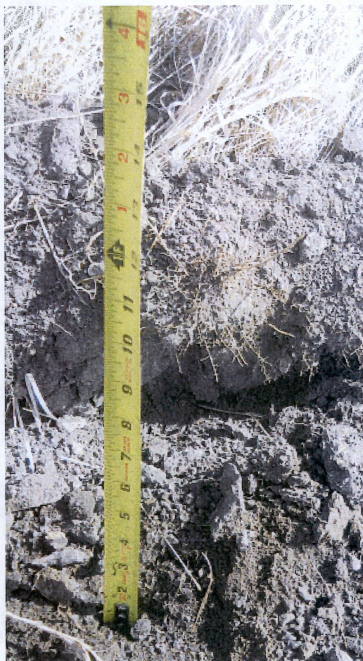
Above: Photo 11- Photo showing depth of approximately 12" top soil after right of way has been stripped. Station location is 118+00.
