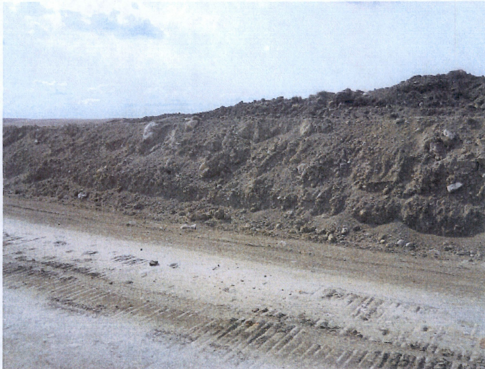
Above: Photo 13- Looking at west side of deep cut through hill at station 124+00. Right of way is stripped showing subsoil at left. Top soil is placed on east edge of right of way beyond subsoil location.
