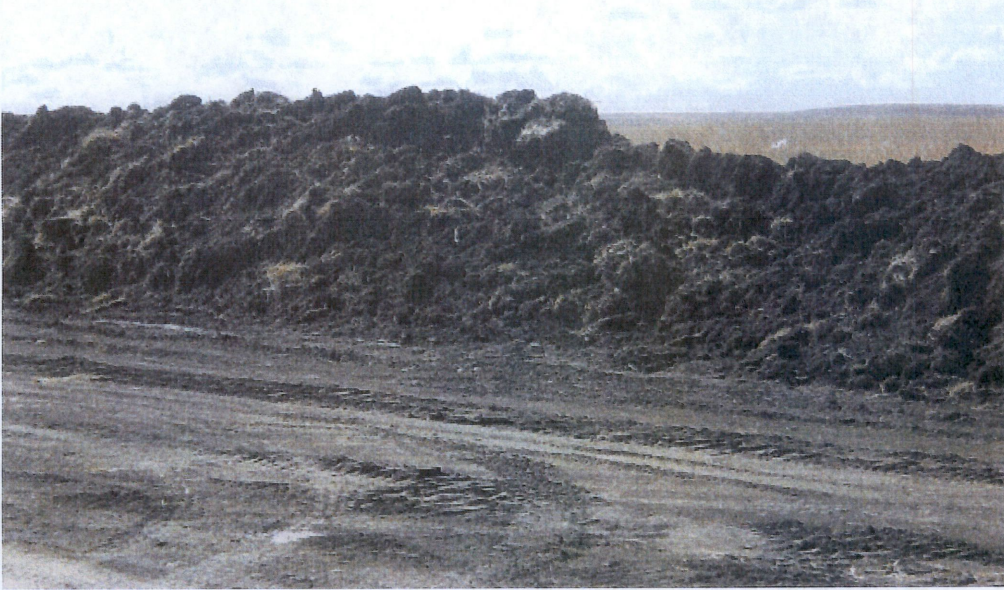
Above: Photo 5- Looking at top soil pushed off right of way located at west side of easement. Photo showing right of way stripped at station 114+00.
