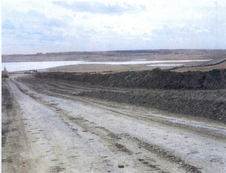
Above: Photo 19- Looking south from graded right of way at station 128+00. Subsoil shown in middle of photo with top soil pushed off right of way at edge of easement at west location. Photo also shows right of way turning west with water slough nesting area beyond. Contractor is shown beyond hydro testing bore piping.
