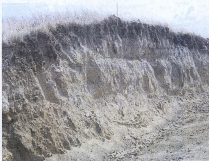
Below: Photo 12- Looking at east side of right of way cut through hillside at station 124+00. Photo showing approximately 12" top soil with subsoil located below.
