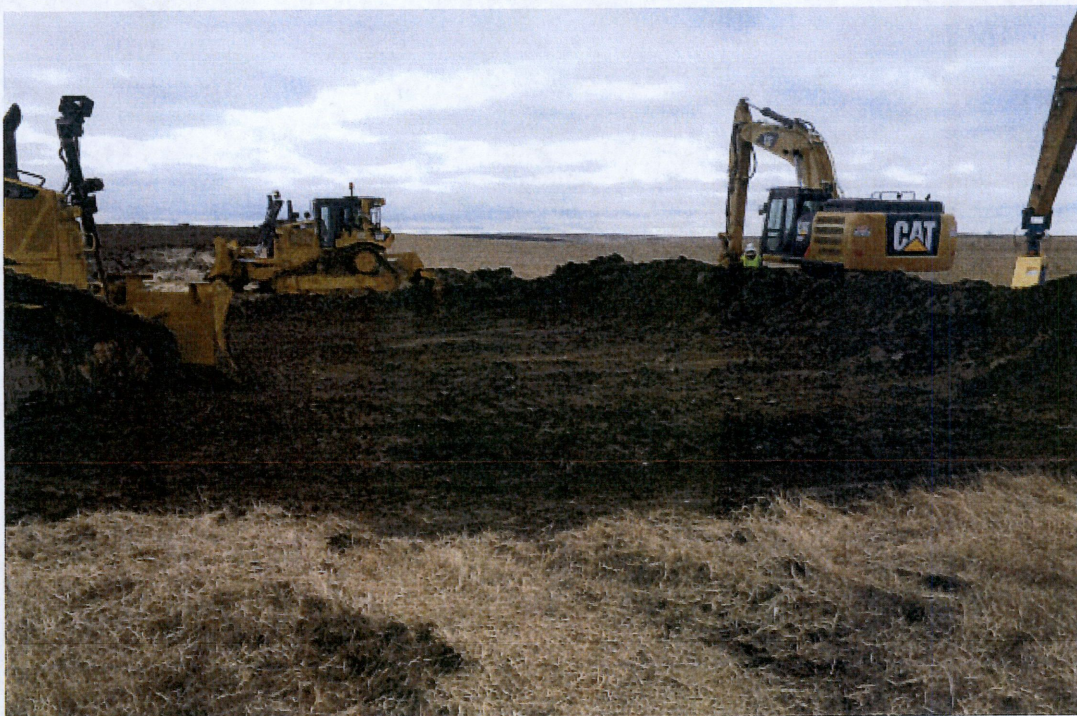
Below: Photo 8- Located at bore exit 111+42.20.South side of Highway 2 looking west. Top soil being stripped and being pushed to opposite side on right of way.
