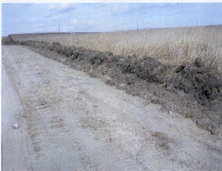
Below: Photo 8- Looking south at station 116+00 showing right of way being stripped with depth of top soil approximately 12". Photo taken at west side of right of way.
