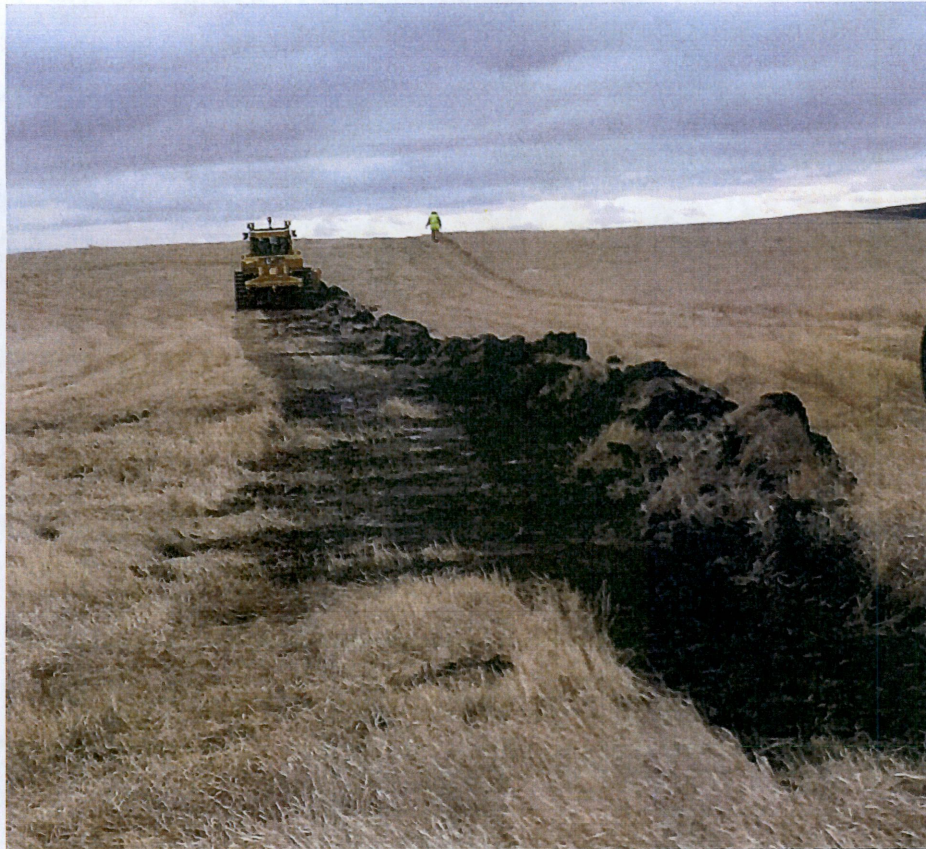
Above: Photo 5- Located at station 118+00. Direction looking south. Right of way extending up hill. Start of top soil stripping on right of way.
