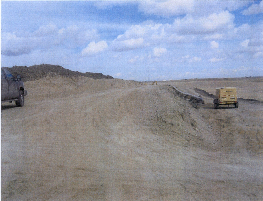
Above: Photo 25- Photo taken from west side of right of way facing east at bore stationing entry 142+52.8 Photo shows graded right of way with top soil shown at upper portion of photo. It appears that top soil is mixed together with subsoil deposit.
