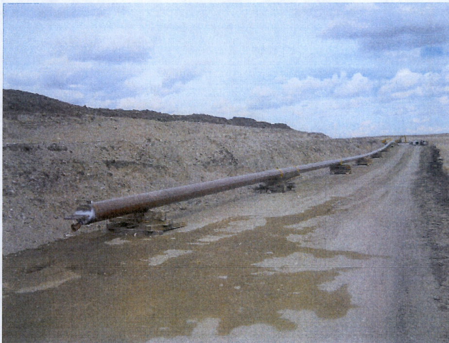
Below: Photo 26- Looking at west side of bore piping placed on skids at bore station 142+52.8. Photo showing right of way graded with top soil shown at top of photo. It appears that top soil is mixed together with subsoil deposits.
