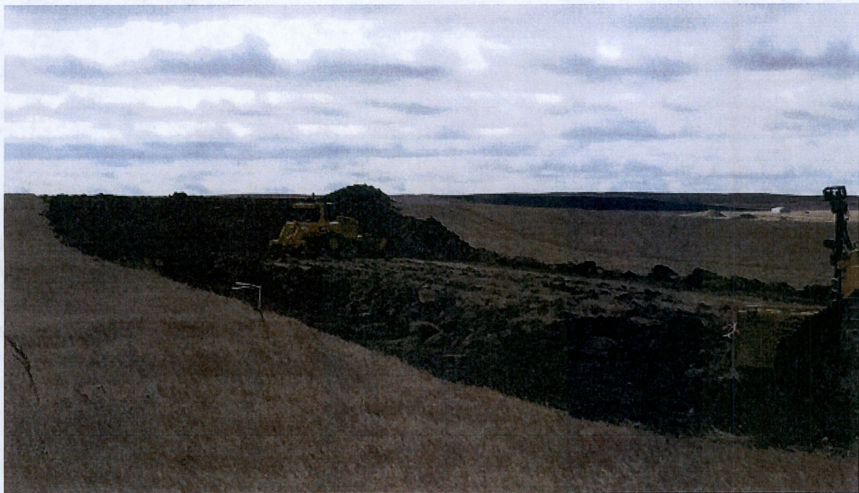
Below: Photo 10- Located at station 116+00 looking south/southwest. Top soil being stripped and pushed to west side on edge of right of way easement.
