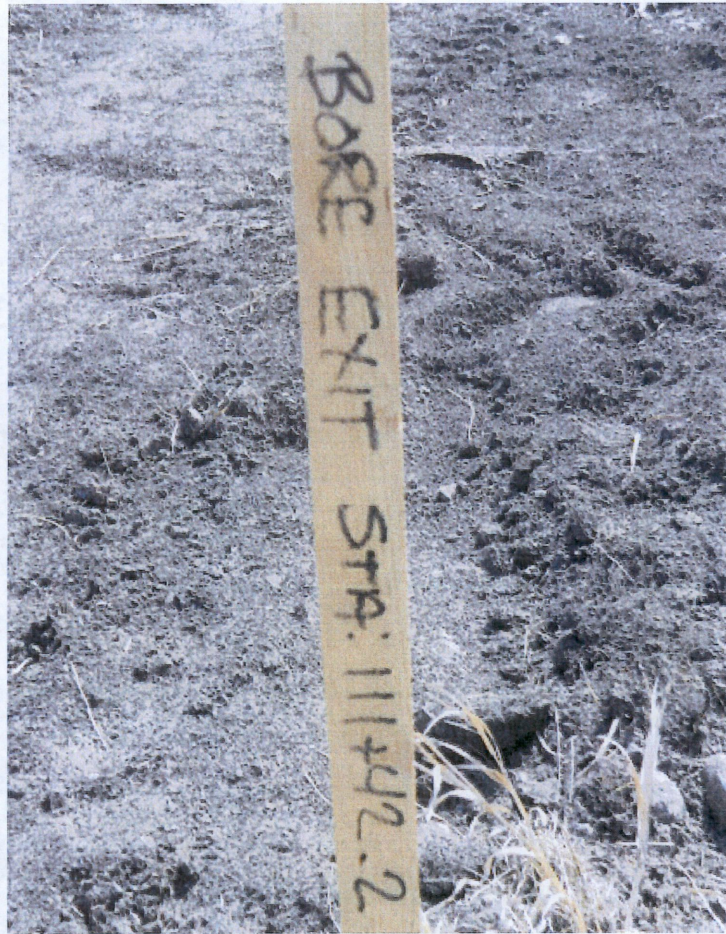
Above: Photo 1- Start of right of way inspection at bore exit stationing 111+42.2 located on south side of Highway 2. Photo shows start of top soil stripping.
