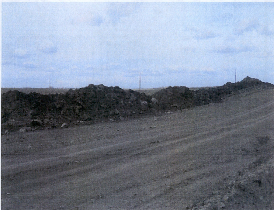
Below: Photo 16- Looking at west side of right of way with easement heading south. Photo location approximately 126+00. Work done from photo shows right of way graded with op soil placed on west side of right of way. Large rocks pushed off right of way into top soil location. Rocks need to be removed off right of way.
