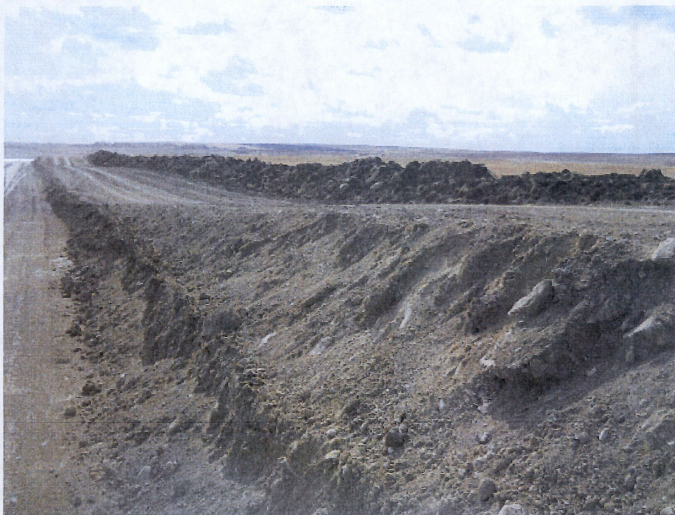
Below: Photo 14- Looking south at stripped right of way through hillside showing subsoil location with top soil placed at edge of right of way on west side of easement.
