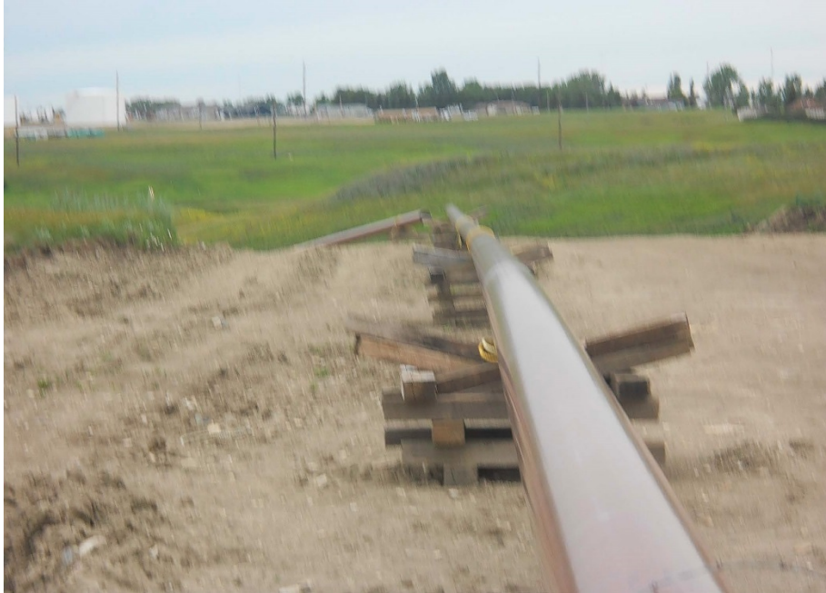
Photo 33 - Located at station 414+00, photo looking south west, showing pipe sitting on skids ready to be bored under wetland across from Enbridge tanks.
