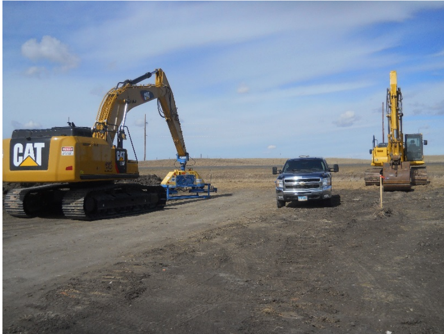
Photo 13 - Located at station 111+42.20, looking north across Highway 2. Bore exit on south side of Highway. Construction equipment on excavation getting ready to start bore pits.
