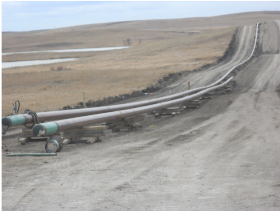
Photo 17 - Located at station 130+00, looking west showing graded Right of Way with bore pipe sitting on skids and under hydro test. Bore piping to be pulled under site slough when hydro test completed. Contractor was onsite at time of inspection.
