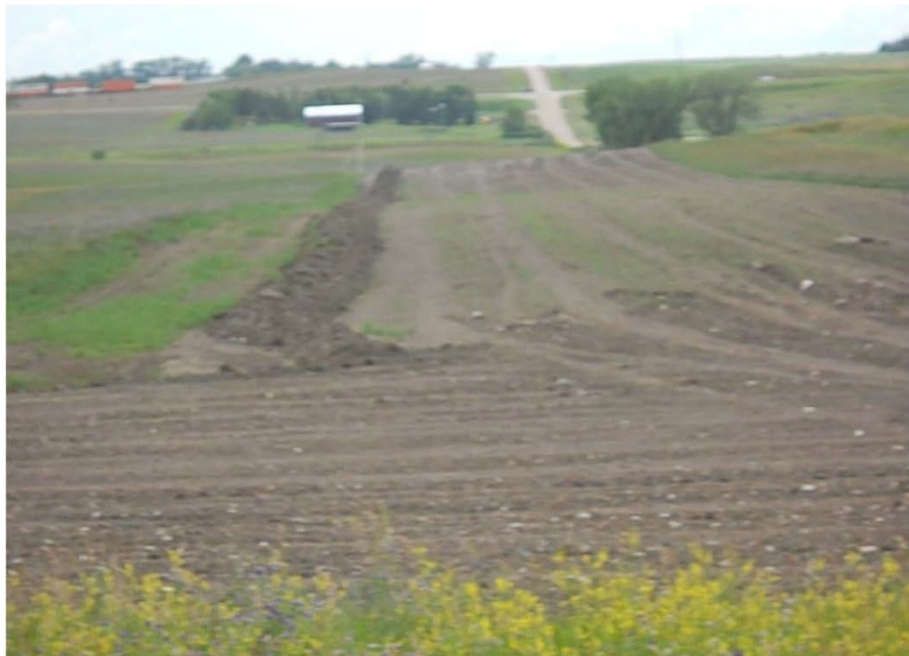
Photo 22 - Located at station 174+00, photo looking south at graded Right of Way, ready to string out pipe. Right of Way extends left towards west.
