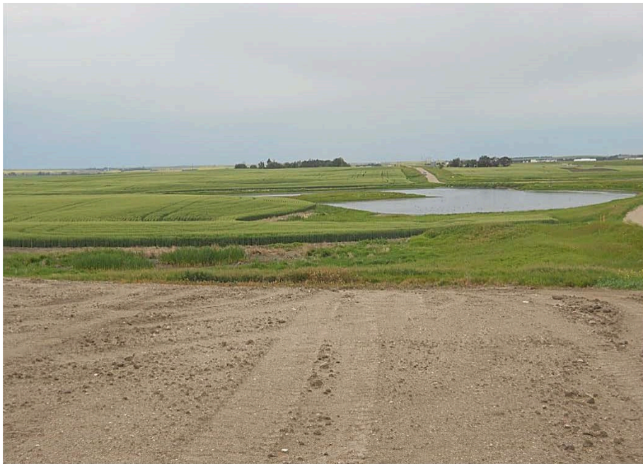
Photo 30 - Located at station 347+70.3, photo looking west at bore entry at wetland. No bore work has started yet. Right of Way is graded.
