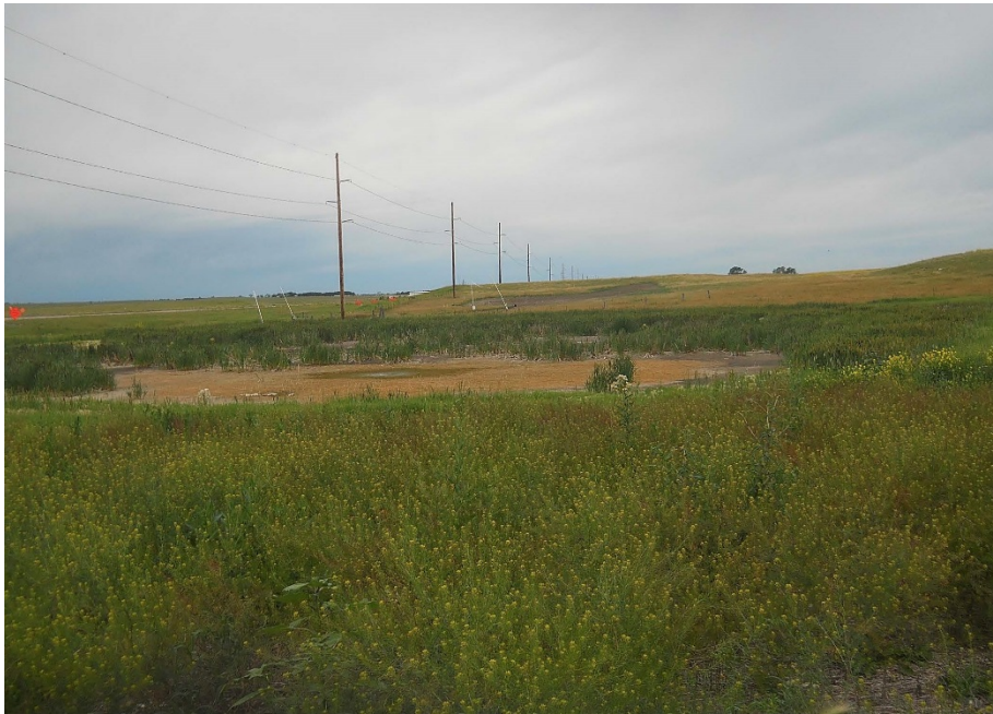
Photo 12: Located at station 98+00, looking southwest at wetland to be bored. At time of inspection, contractor had not gotten to location. Highway 2 is just to the south (left).
