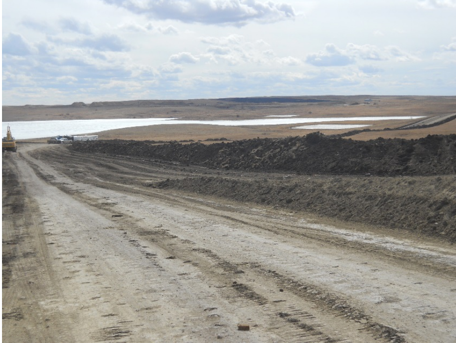
Photo 15 - Located at station 128+00, looking south showing graded Right of Way ready to string out piping and start trenching. Photo also shows Right of Way turning west with water slough nesting area beyond.
