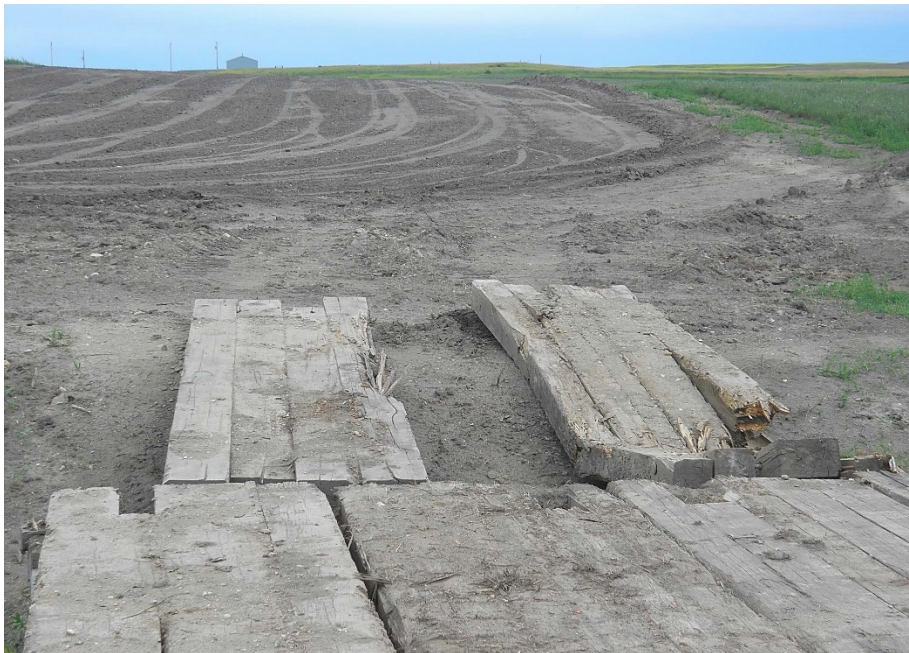
Photo 4: Located at station 24+00, looking west at graded Right of Way, ready for string out pipe. Bridge mats and overhead power markers are installed beyond towards wetland.
