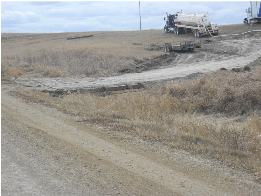
Photo 20 - Located at station 156+00, photo taken from county road 77 th Ave NW, shown bridge mats in road ditch for access point to have contractor perform bore work at station 158+72.8.
