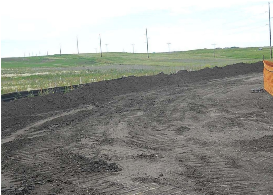
Photo 2: Located at station 8+00, looking south west at graded Right of Way ready for string out pipe. Right of Way has BMP's installed ready to stop any erosion sediment runoff if it should occur.
