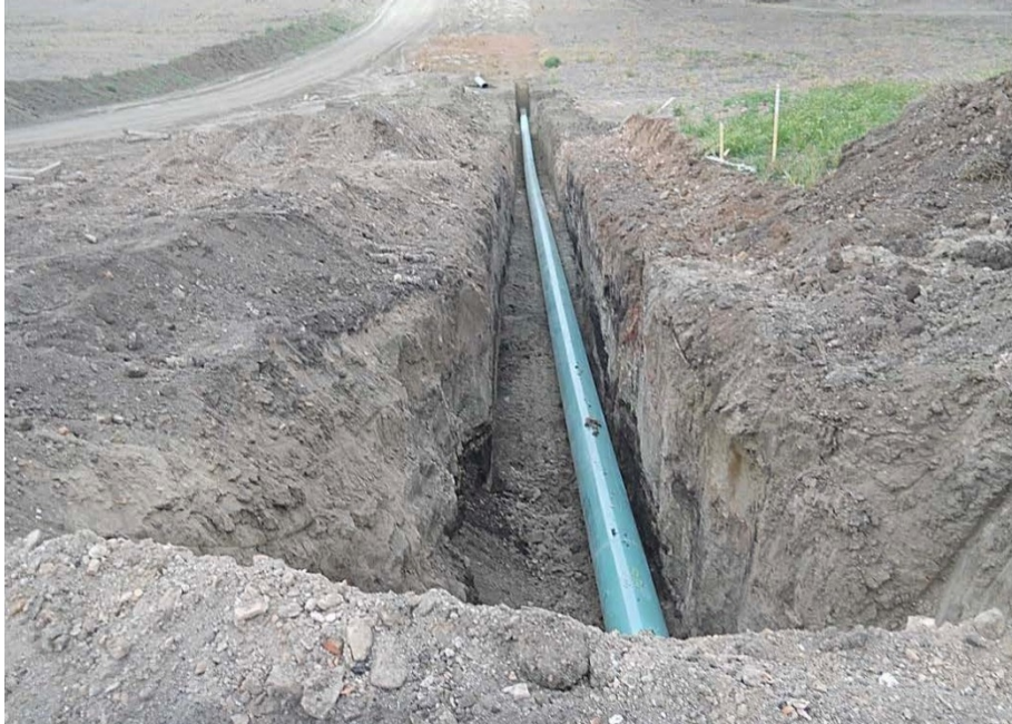
Photo 9: Located at station 70+00, looking west at pipe located in trench. Depth of trench was measured and found to have 4'0" of cover from the top of pipe.
