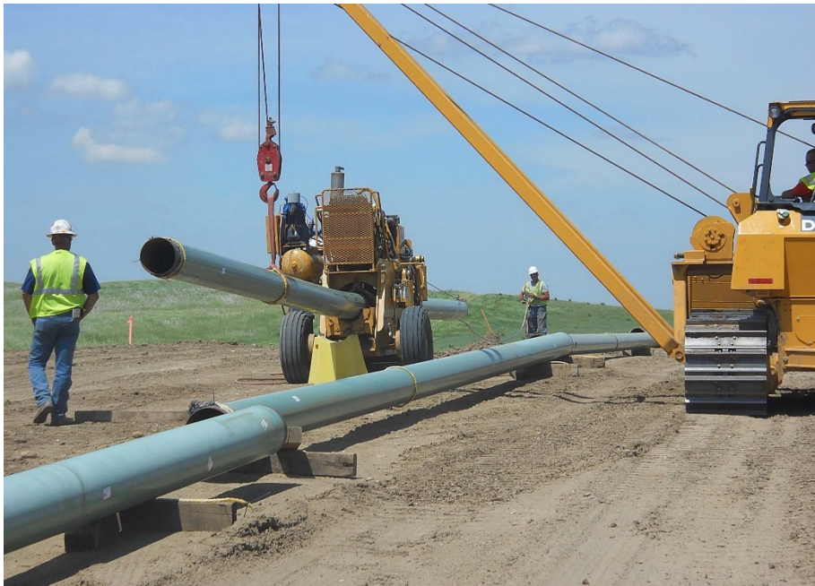
Photo 26 - Located at station 246+00, photo looking south with contractor bending pipe as required for installation. Pipe is strung out on graded Right of Way ready for welding and trenching.
