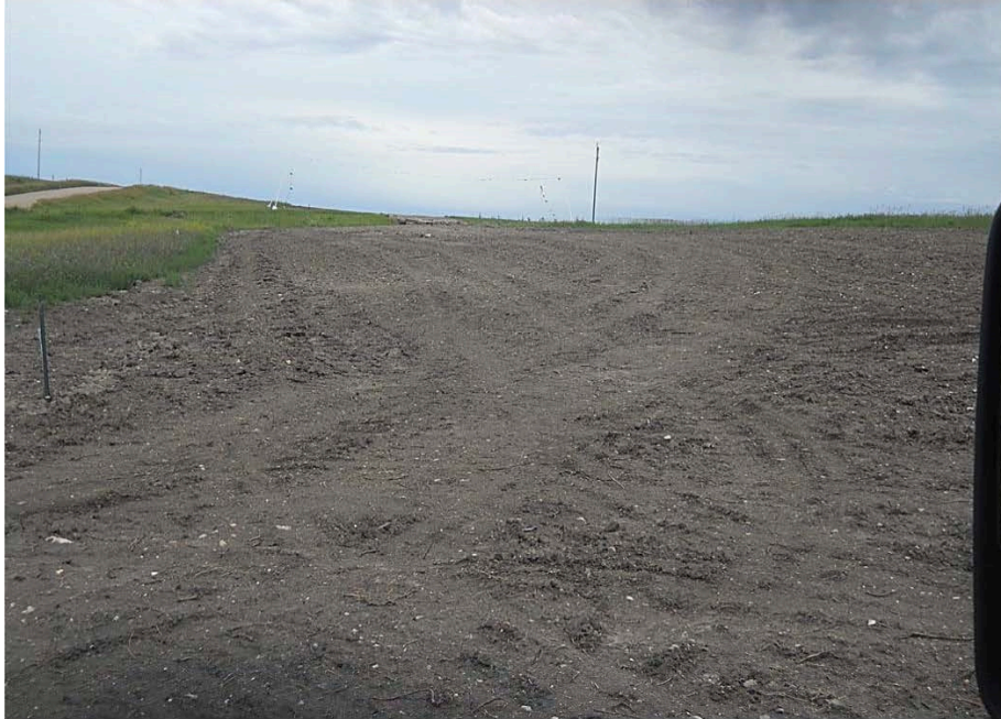
Photo 3: Located at station 14+00, looking west at graded Right of Way, ready for string out pipe. Bridge mats and overhead power markers are installed beyond towards wetland.
