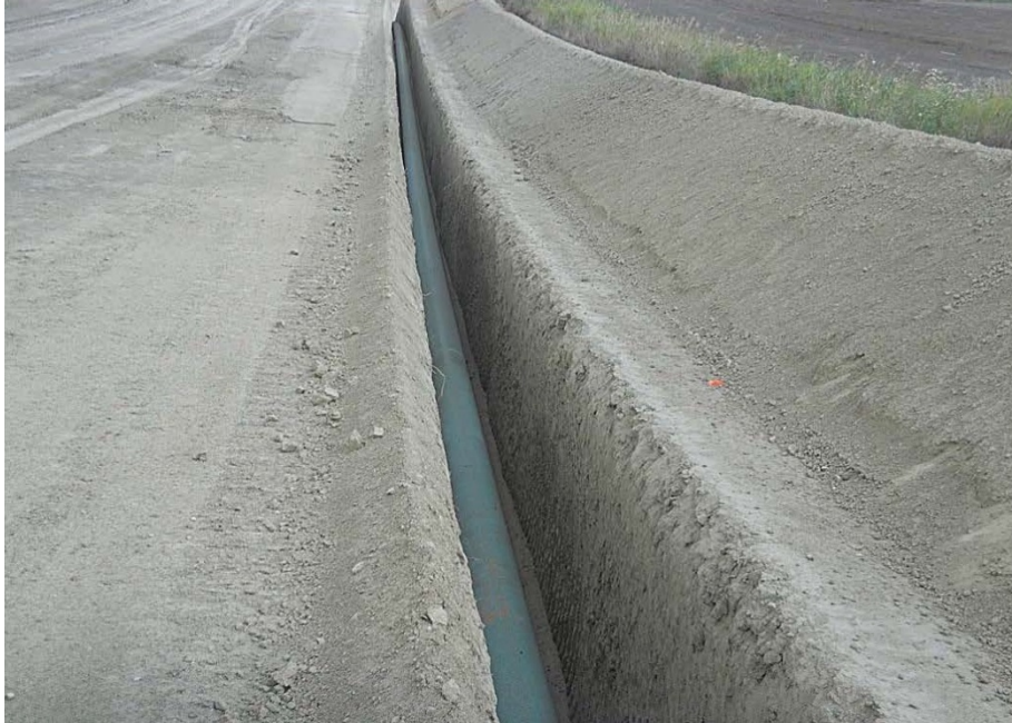
Photo 31 - Located at station 368+00, photo looking west showing piping installed in trench. Depth of trench was measured and was found to have top of pipe 4'0" to top of Right of Way trench opening. Trench was ready to be backfilled.
