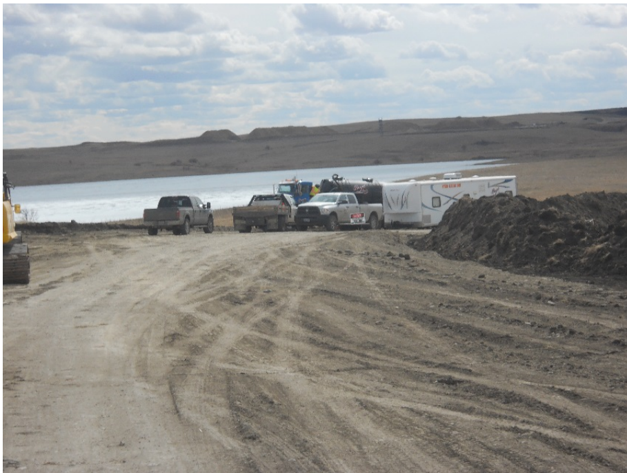
Photo 16 - Located at station PI 128+43.8, looking south where Right of Way turns right and heads west. Photo shows contractor on site hydro testing welded bore piping.
