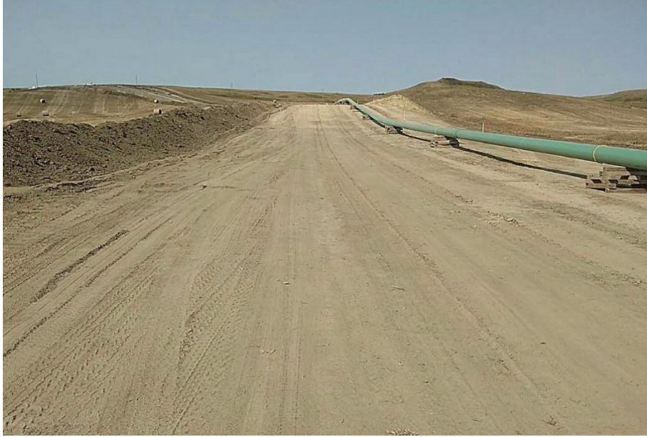
Photo 27 - Located at station 250+00, photo looking south at graded Right of Way with welded piping sitting on skids ready for trenching.
