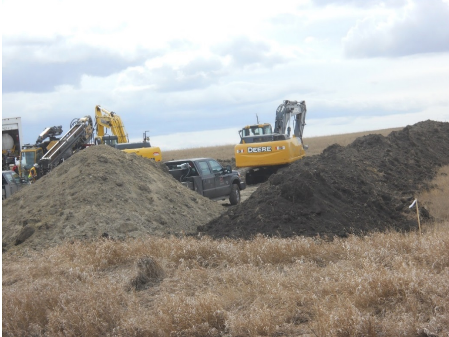
Photo 21 - Located at station 158+72.8, photo taken at bore pit exit station, located on west side of County Road 77 th Ave NW, at time of inspection contractor on site doing bore work.
