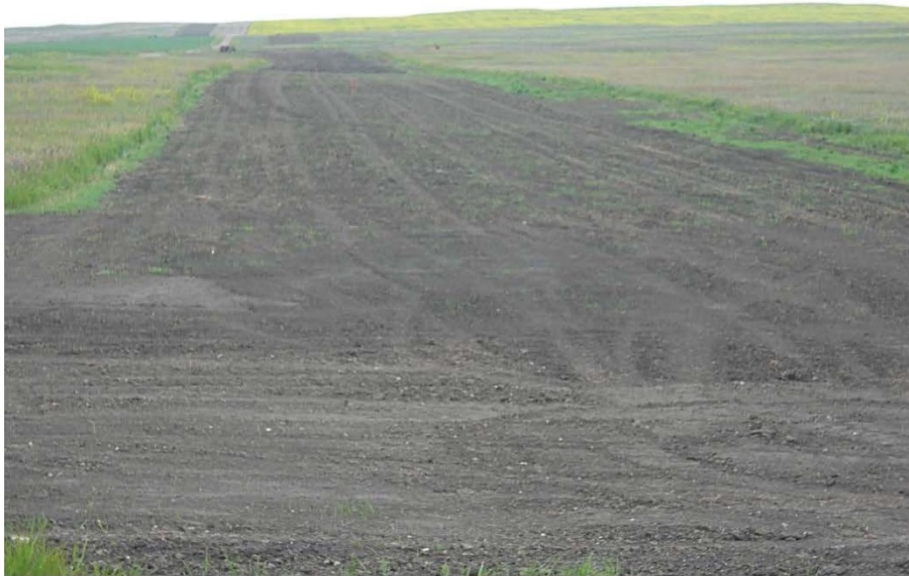
Photo 24 - Located at station 220+00, photo looking north west at graded Right of Way ready to string out pipe.
