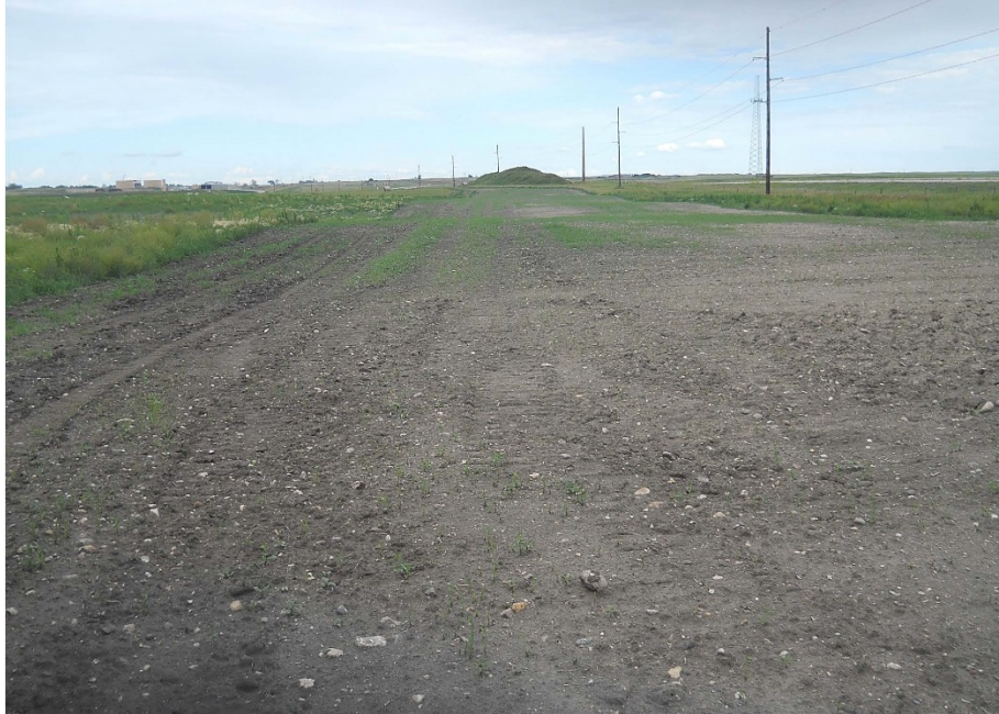
Photo 11: Located at station 84+00, looking south east at graded Right of Way, ready to string out piping. Right of Way is located on north side of Highway 2.
