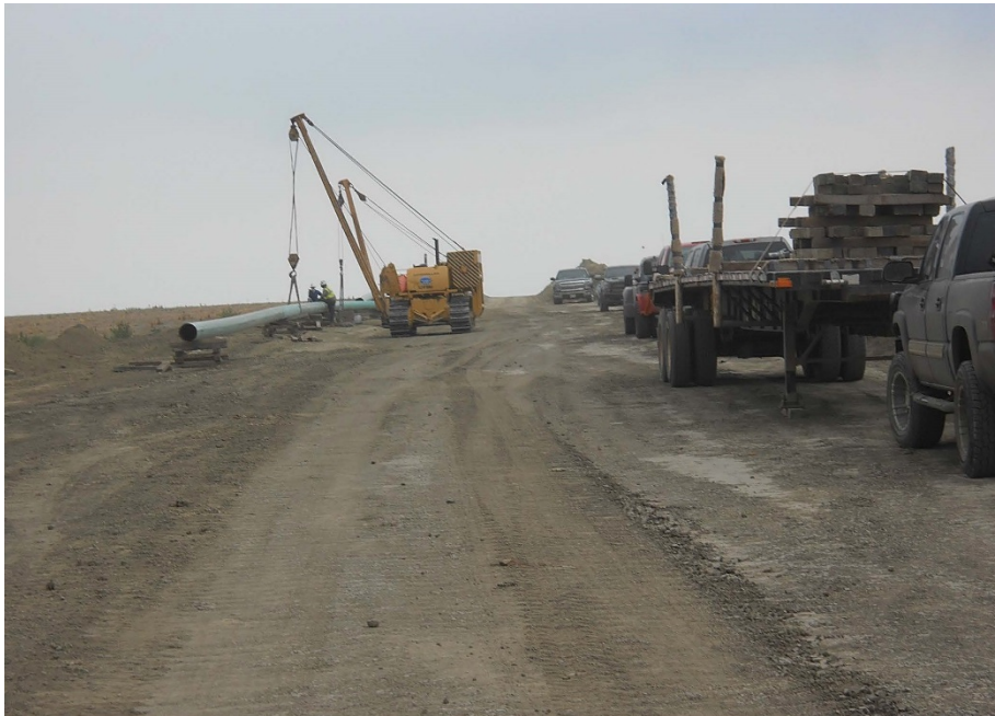
Photo 28 - Located at station 310+00, photo looking west showing contractor working on installing welded piping into trench.
