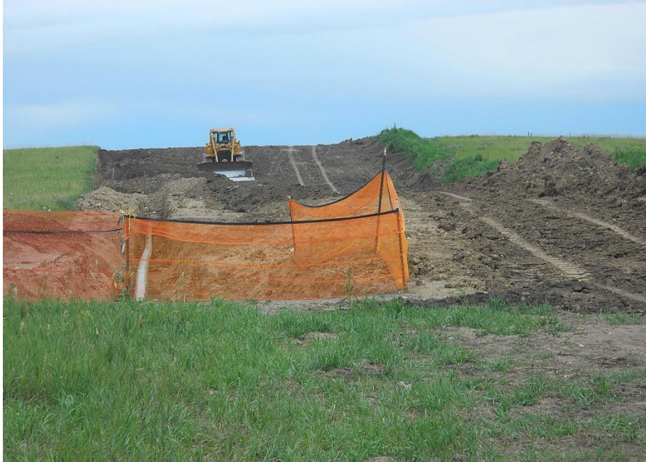
Photo 23 - Located at station 199+76.6, photo looking south at bore entry station, with bore exit station 203+57.3 beyond. Right of Way graded and ready to string pipe. Bore pit was rated during inspection to have installed fence barricade for safety.
