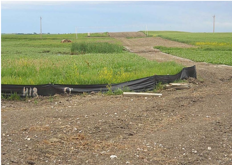
Photo 6: Located at station 34+00, looking west showing Right of Way with BMP's installed with bridge matting laid across wetland for Right of Way access. Overhead power connection lines beyond.
