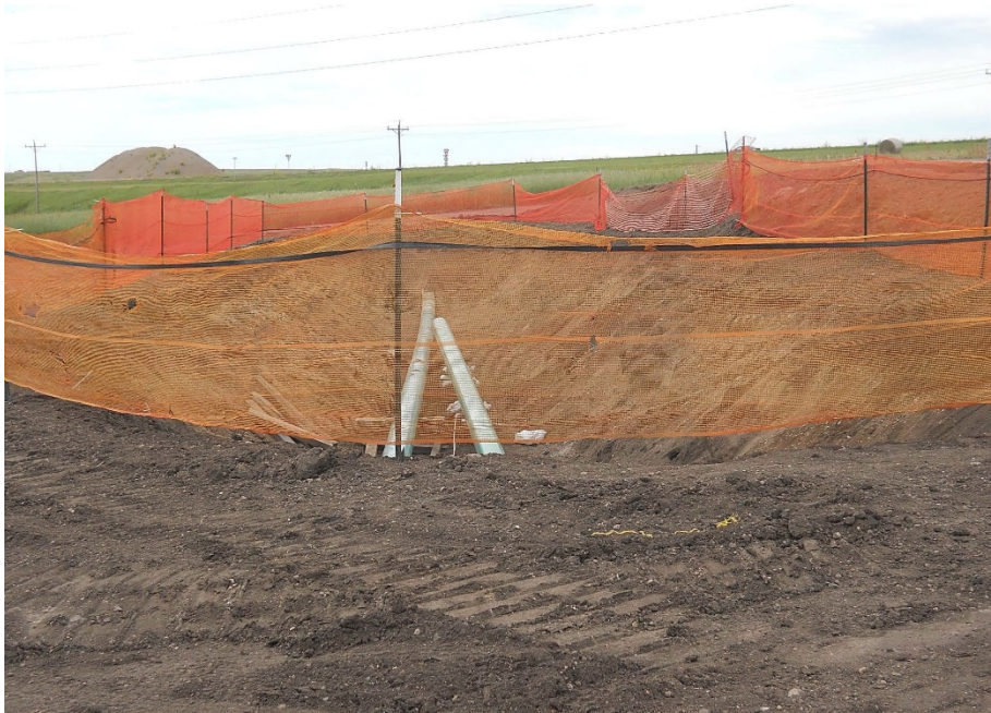
Photo 10: Looking west at bore pit entry Station PI 24+75.81 and exit bore pit beyond station PI 76+47.7, to cross under oil well access road. Piping has been pulled into bore pits and ready for connection.
