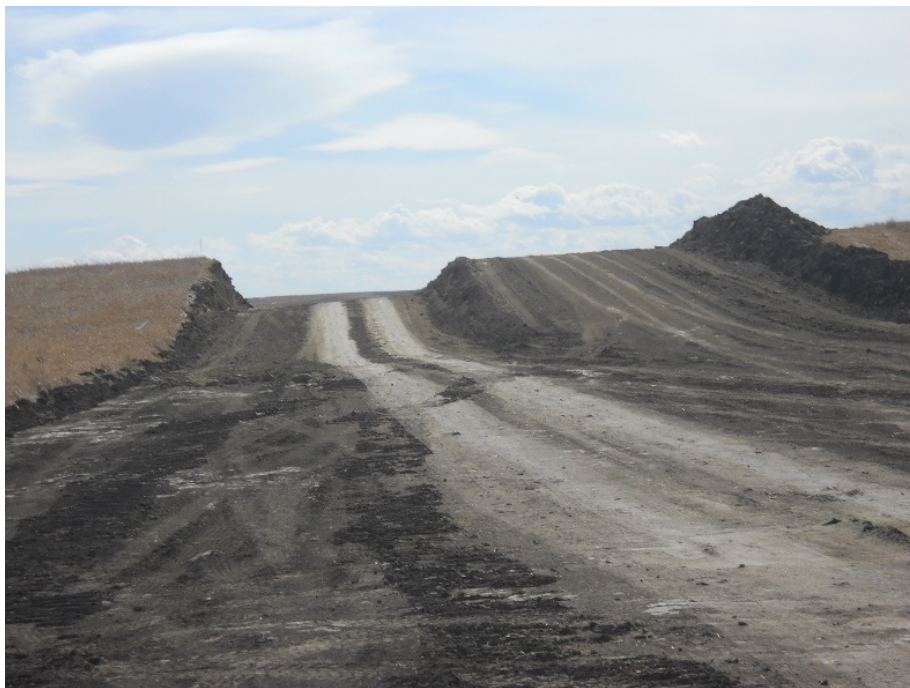
Photo 14 - Located at station 120+00, looking south showing graded Right of Way ready for pipe installation and trenching.
