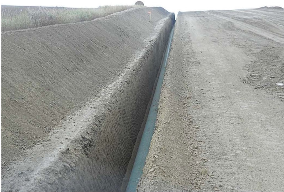
Photo 29 - Located at station 316+00, photo looking west showing piping installed in trench. Depth of trench was measured and was found to have top of pipe 4'-0" to top of Right of Way trench opening. Trench appeared to be ready to be backfilled.
