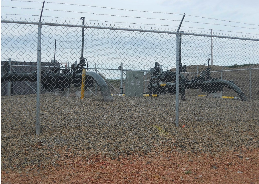
Photo 1: Located at station 2+00, looking north east at Palermo tie-in locations, for Beginning of Pipe (BOP) start.
