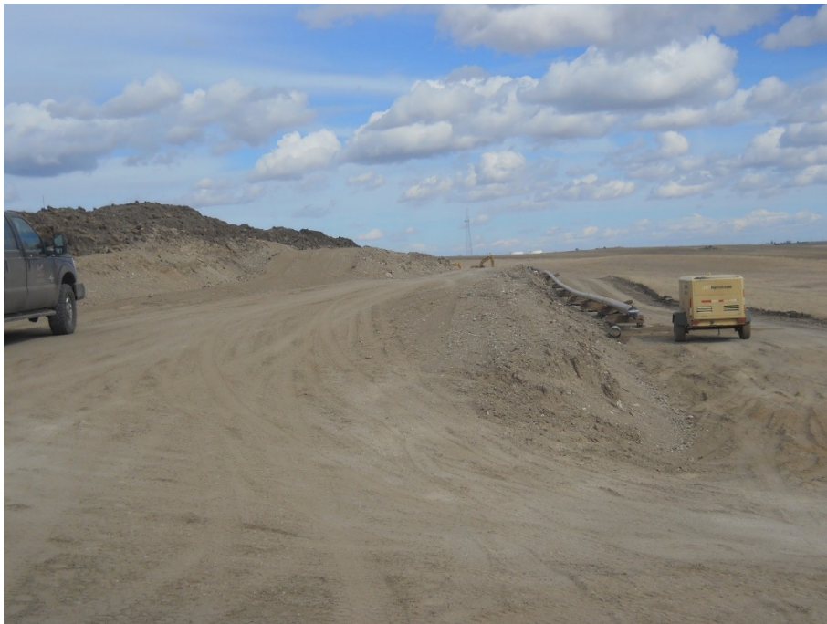
Photo 18 - Located at station 142+52.8, photo taken from west end of Right of Way facing east at bore entry. Bore piping being hydro tested at time of inspection.
