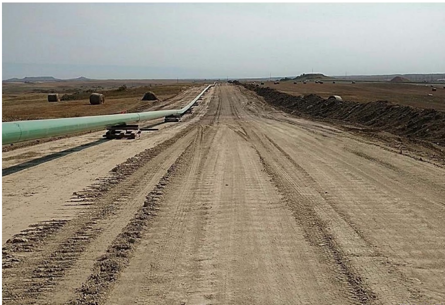
Photo 8: Located at station 62+00, looking east showing piping welded and sitting on skids ready for excavation. Piping is located on graded Right of Way.
