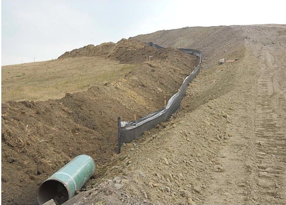
Photo 25 - Located at station 232+00, photo looking north west showing graded Right of Way with BMP silt fence installed to separate top and subsoil types from touching. Right of Way turns and heads south.
