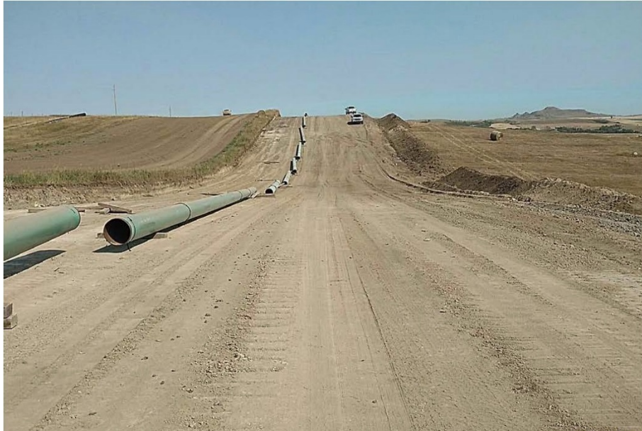
Photo 7: Located at station 54+00, looking east showing piping strung out on Right of Way, ready for welding.
