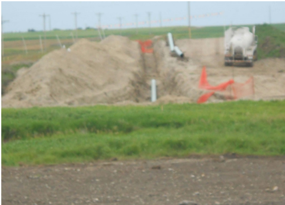
Photo 32 - Located at station 412+75.9, photo looking east at bore pit. Piping has been bored under wetland, with pipe pulled through trench. Fenced barricade has been installed around bore pit.
