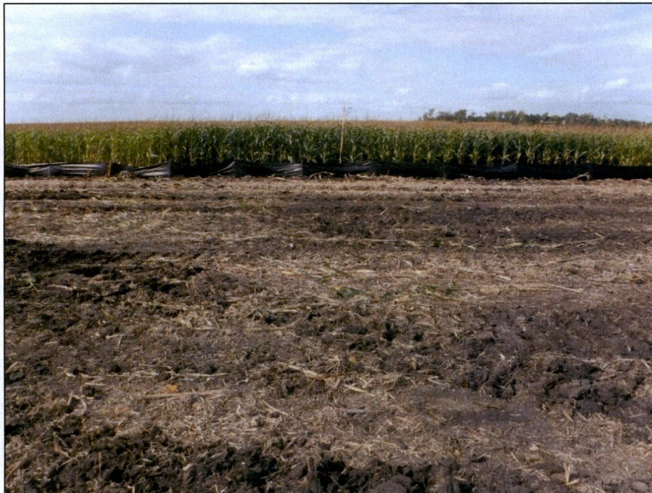
Figure 10. Outfall 005, silt fence installed on the south side of the Maple River at Station 098+00, looking north.
