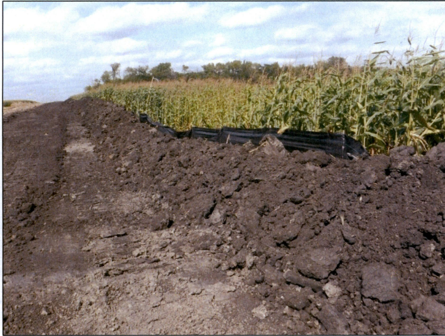
Figure 9. Outfall 004, silt fence on the east side of the ROW at Station 084+00 and Station 085+00.
