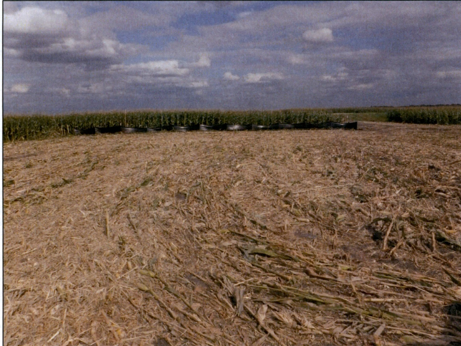
Figure 13. Outfall 006, silt fence installed on the west side of 165th Ave. SE. between Station 194+00 and Station 196+00, looking northwest.
