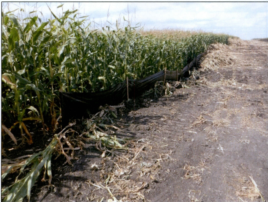
Figure 8. Outfall 004, silt fence on the west side of the ROW at Station 084+00 and Station 085+00.
