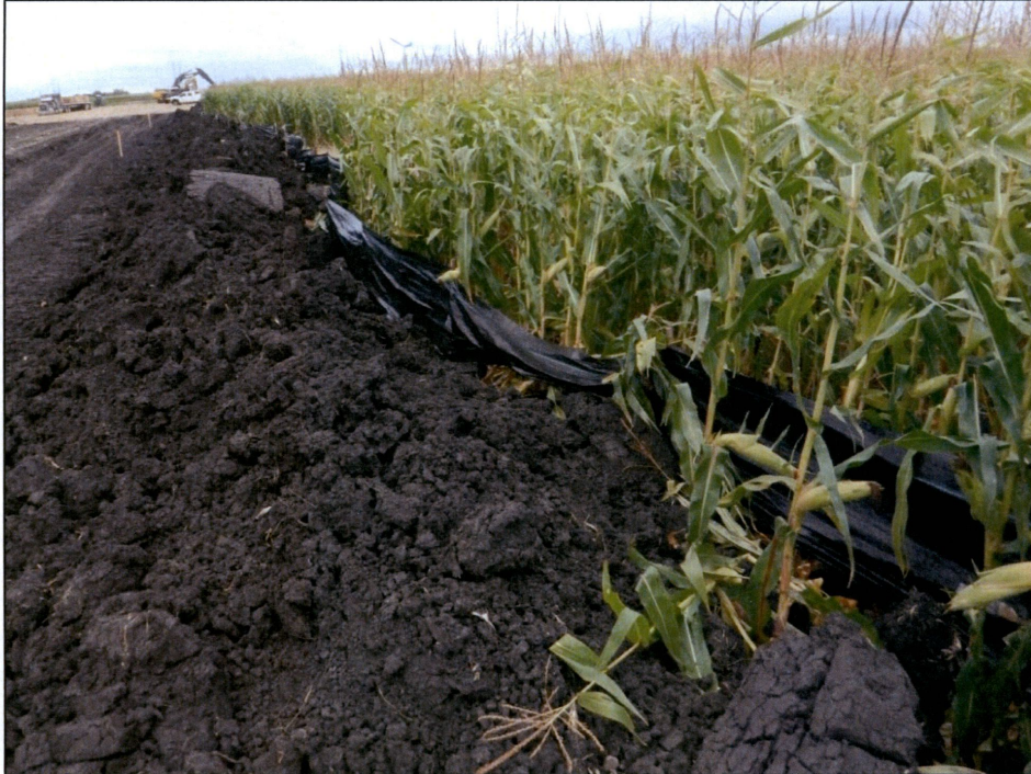
Figure 1. Outfall 001– Silt fence installed on the north side of the ROW at Station 002+40 to Station 004+40, looking northwest.
