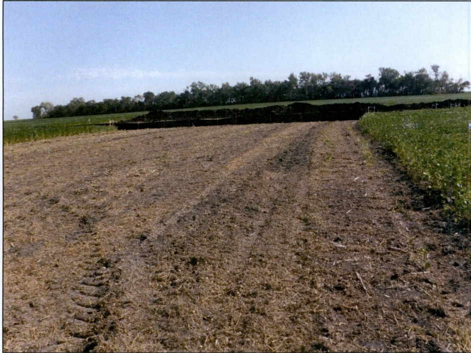
Figure 7. Outfall 003, silt fence on the north side of County Road 20, looking south.
