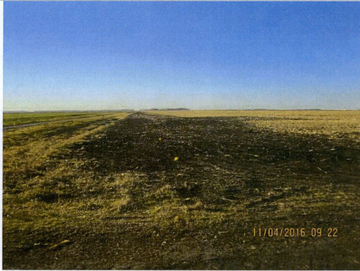
Photo 16: South side of open trench, south side of Maple River (looking south).
