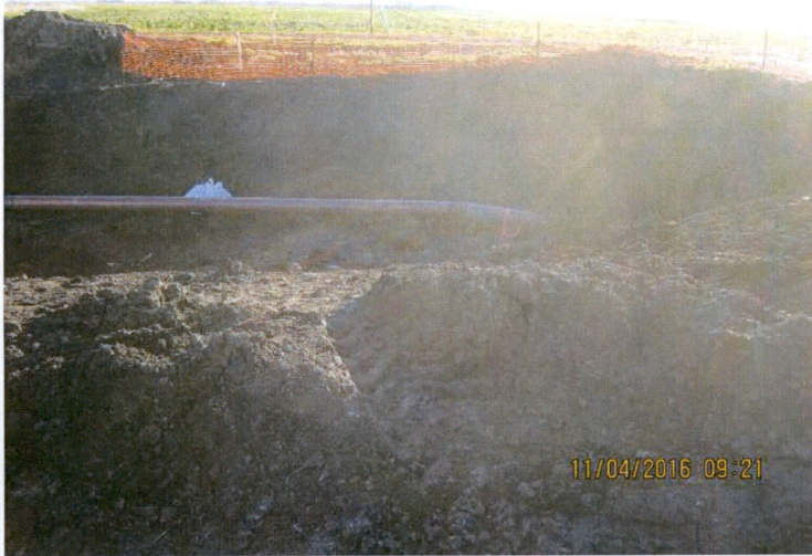
Photo 3: View of pipe depth installed on south side of Maple River (northern portion of alignment).
