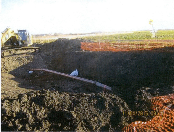
Photo 1: View of pipe depth installed on south side of Maple River (northern portion of alignment).
