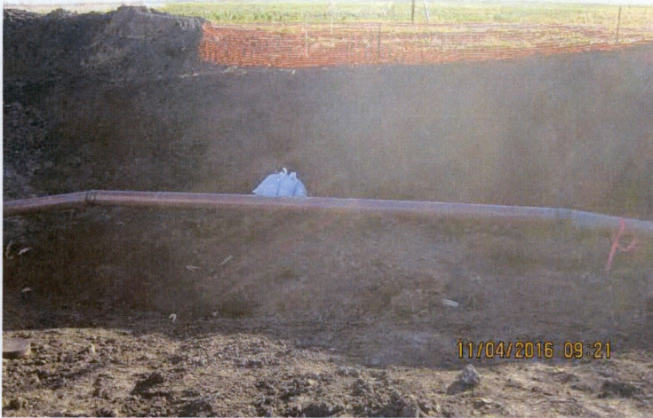
Photo 2: View of pipe depth installed on south side of Maple River (northern portion of alignment).
