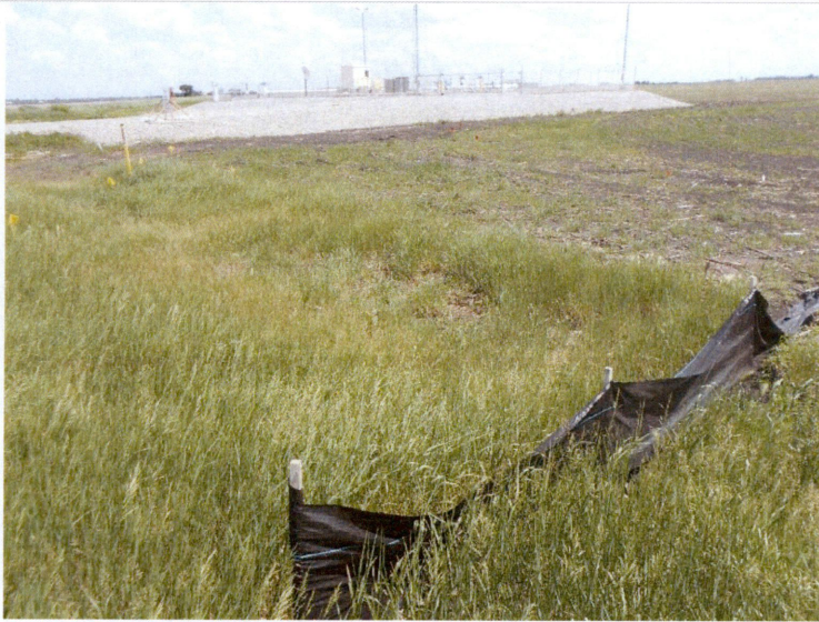
Photo 16: Fargo Terminal silt fencing.
