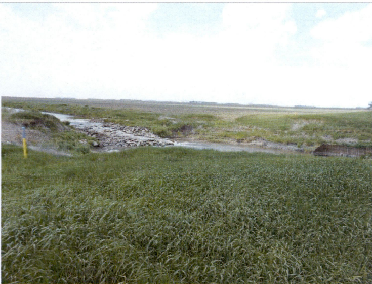
Photo 22 / 23: Project Corridor at Maple River crossing. Horizontal Directional Drilling was used to span the river.
