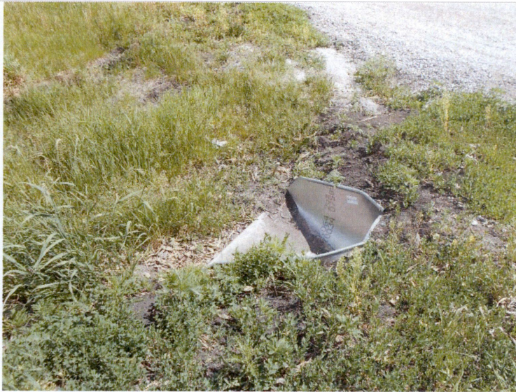
Photo 14: Culvert at Fargo Terminal. No erosion / sedimentation issues, or bare ground observed.
