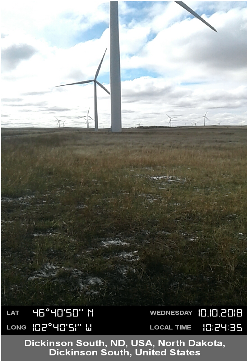
Report Photo #4: Overview of turbine construction block (T63) from North to South.
