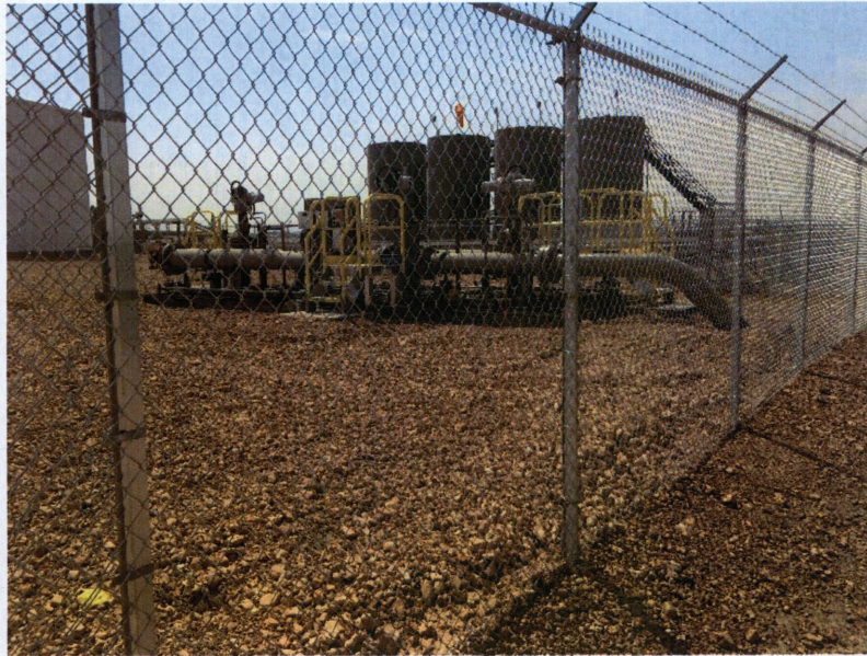
Photo No. 1 Tesoro Pipeline Station 0+00 Starting Point of Pipeline Project South of 40 th Street NW July 31, 2017
