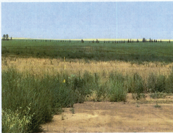
Photo No. 4 Tesoro Pipeline Station 4+20 to 7+81 PI #2 of Pipeline Project South of 40 th Street NW July 31, 2017
