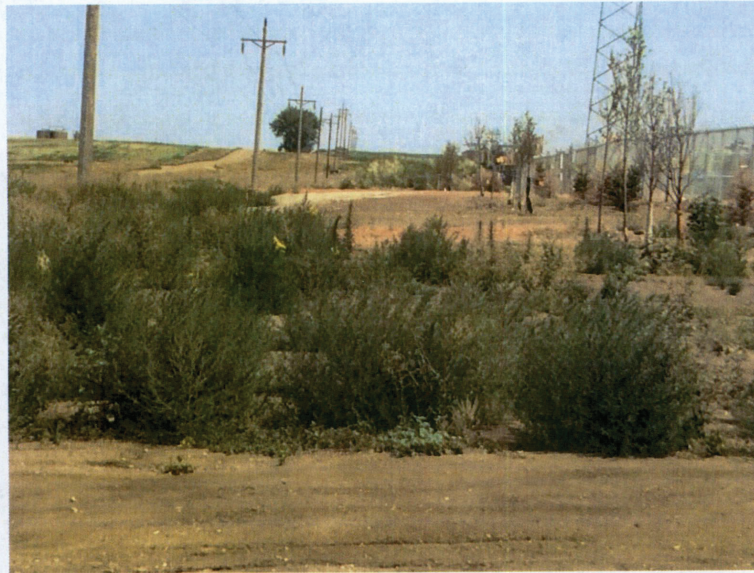
Photo No. 3 Tesoro Pipeline Station 4+00 to 0+57 PI #2 of Pipeline Project South of 40 th Street NW July 31, 2017
