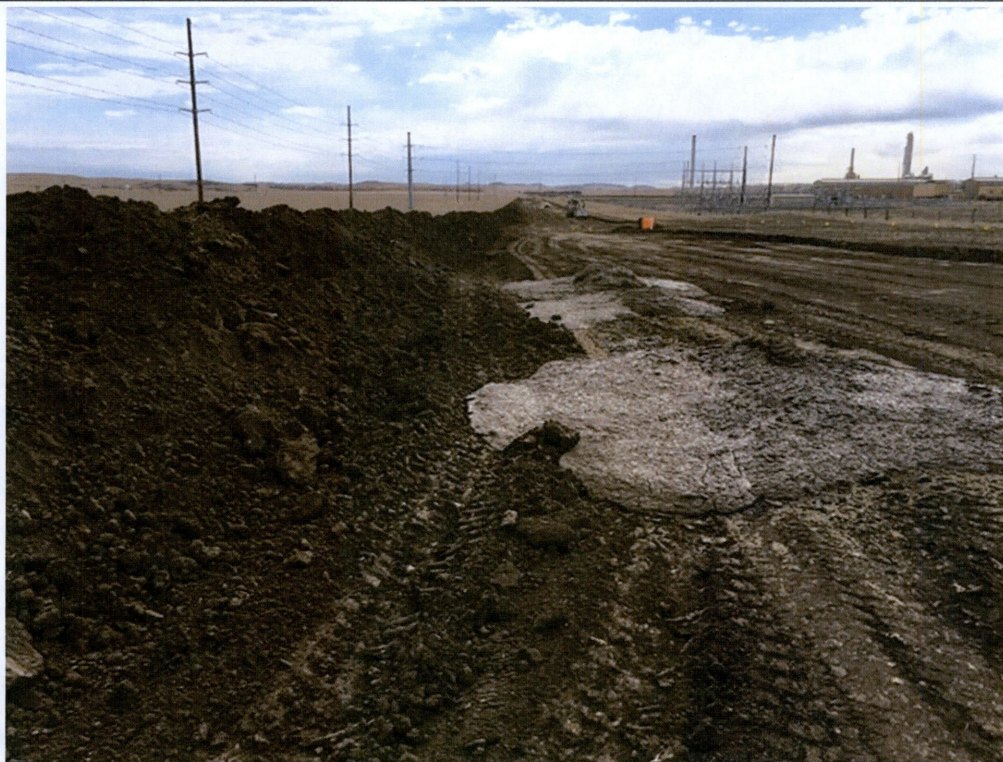
Photo 11 – Approx. Station 30+00. Hydro vac spoil encroaching on topsoil pile.
