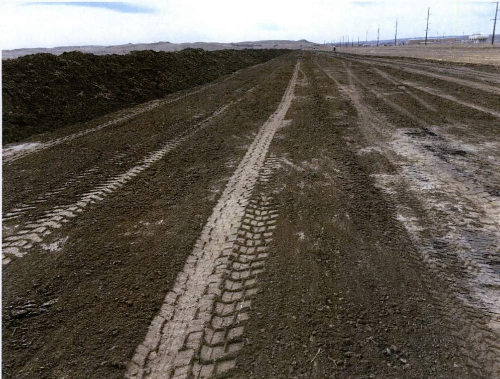
Photo 7 – Approx. Station 43+00. View of area with insufficient depth of removed topsoil.
