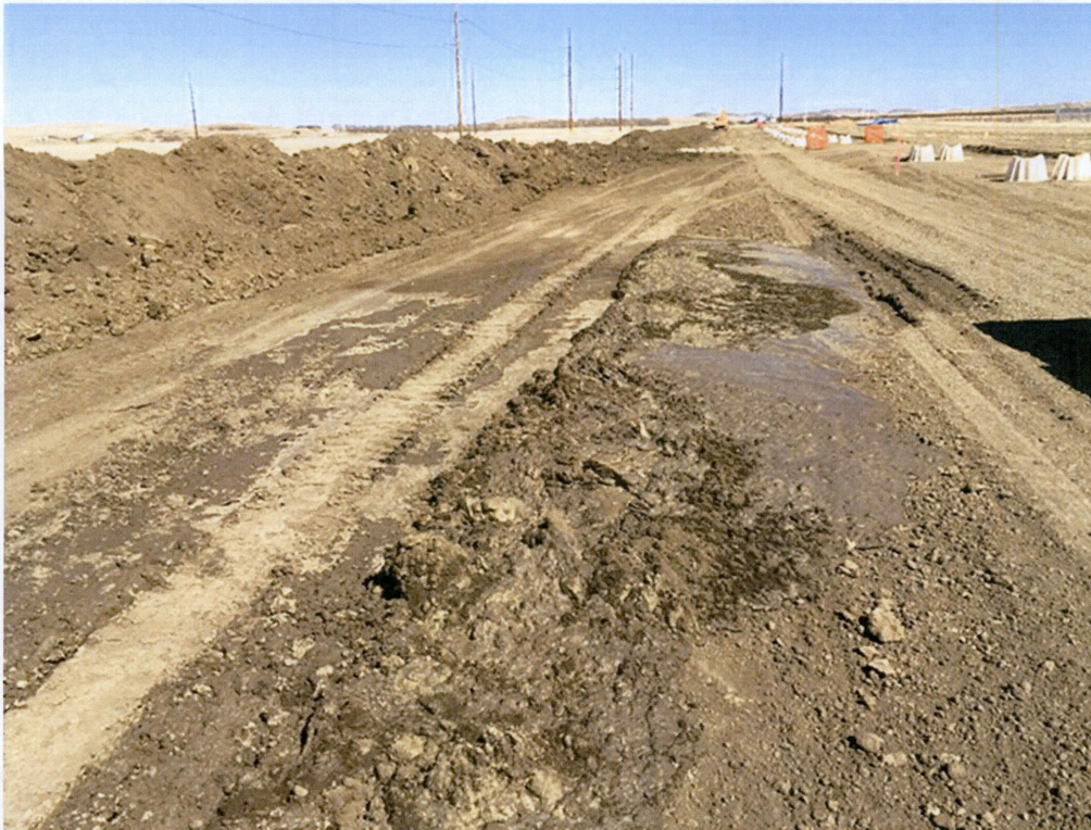
Photo 13 – Approx. Station 30+00. View of the hydro vac spoil separated from the topsoil pile.
