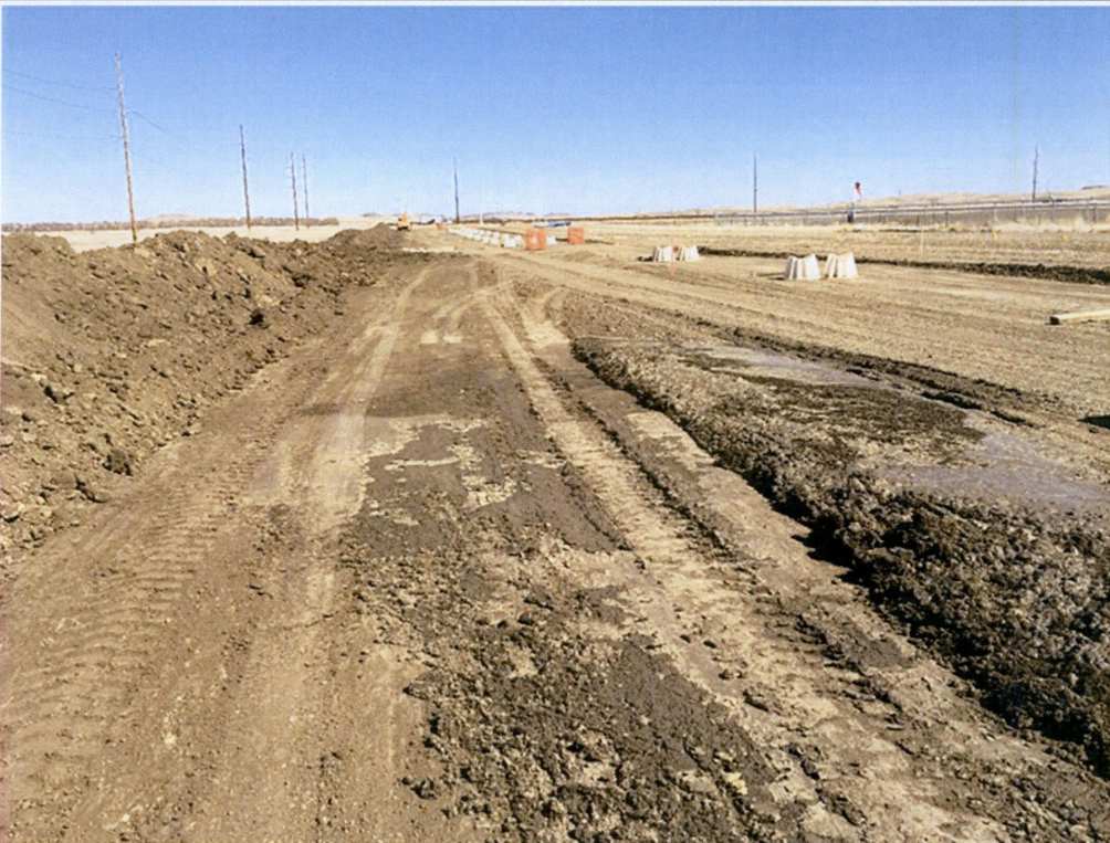
Photo 14 – Approx. Station 30+00. View of the hydro vac spoil separated from the topsoil pile.
