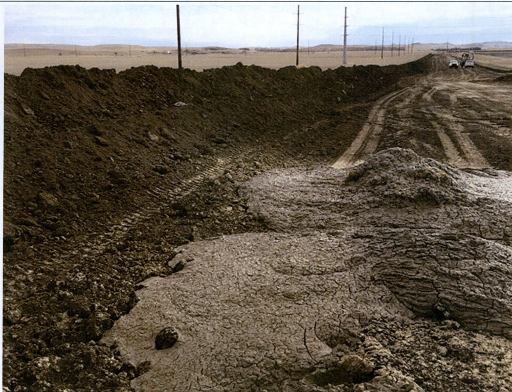
Photo 12 – Approx. Station 30+00. Hydro vac spoil encroaching on topsoil pile.
