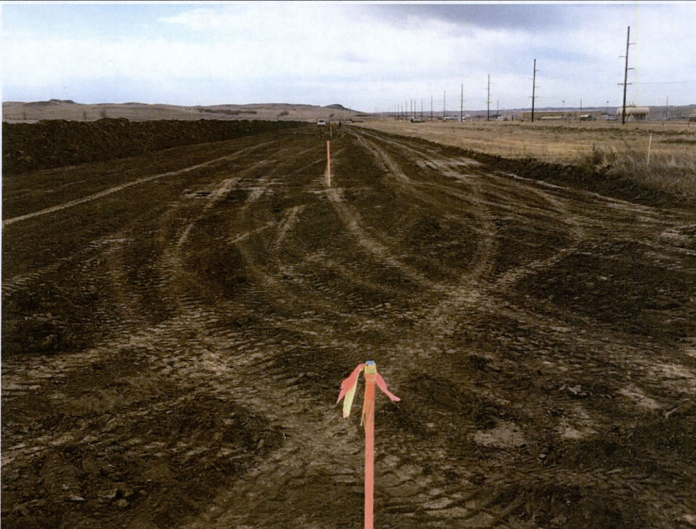
Photo 8 – Approx. Station 43+00. View of area with insufficient depth of removed topsoil.
