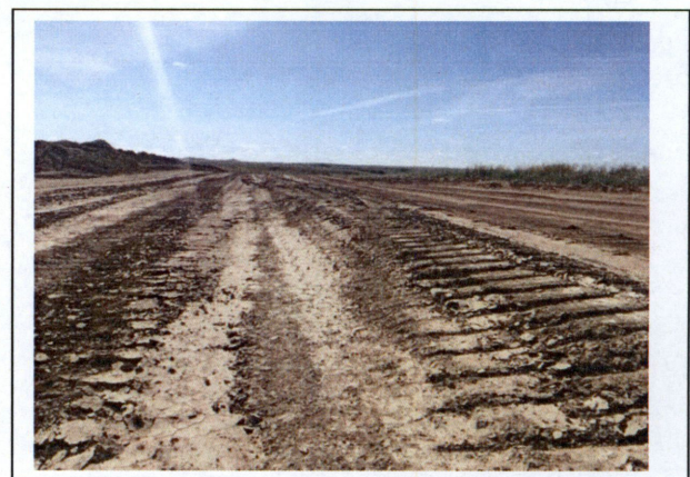
6. View E; St. 520; rough grade complete trench subsoil backfilled; topsoil remains separated
