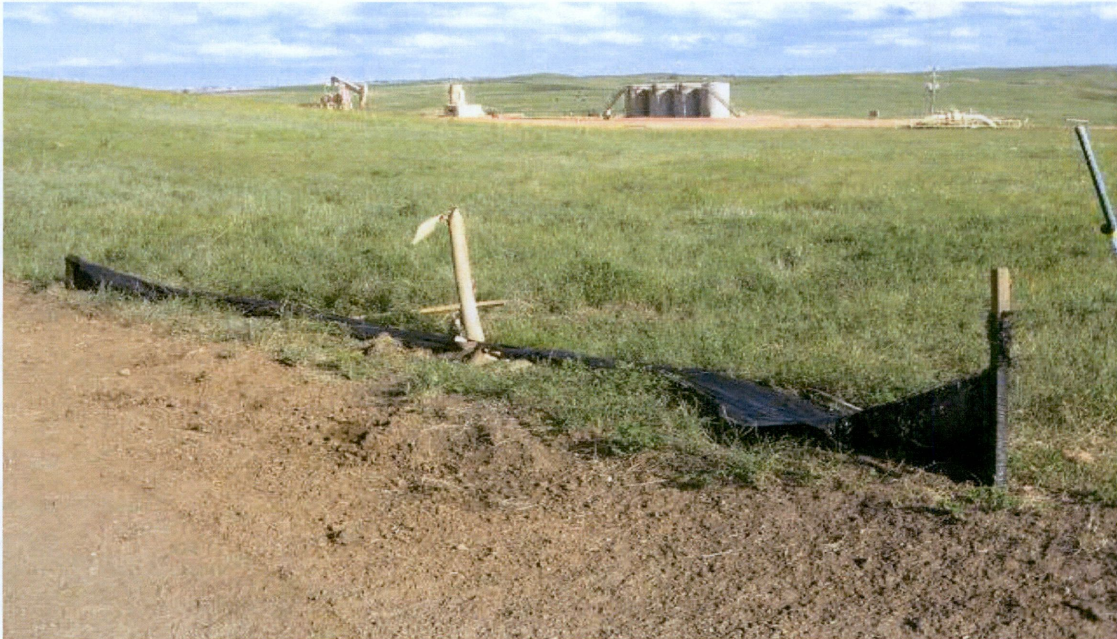
Photo 11 – Approx. Station 604+00. View of erosion control requiring repair.
