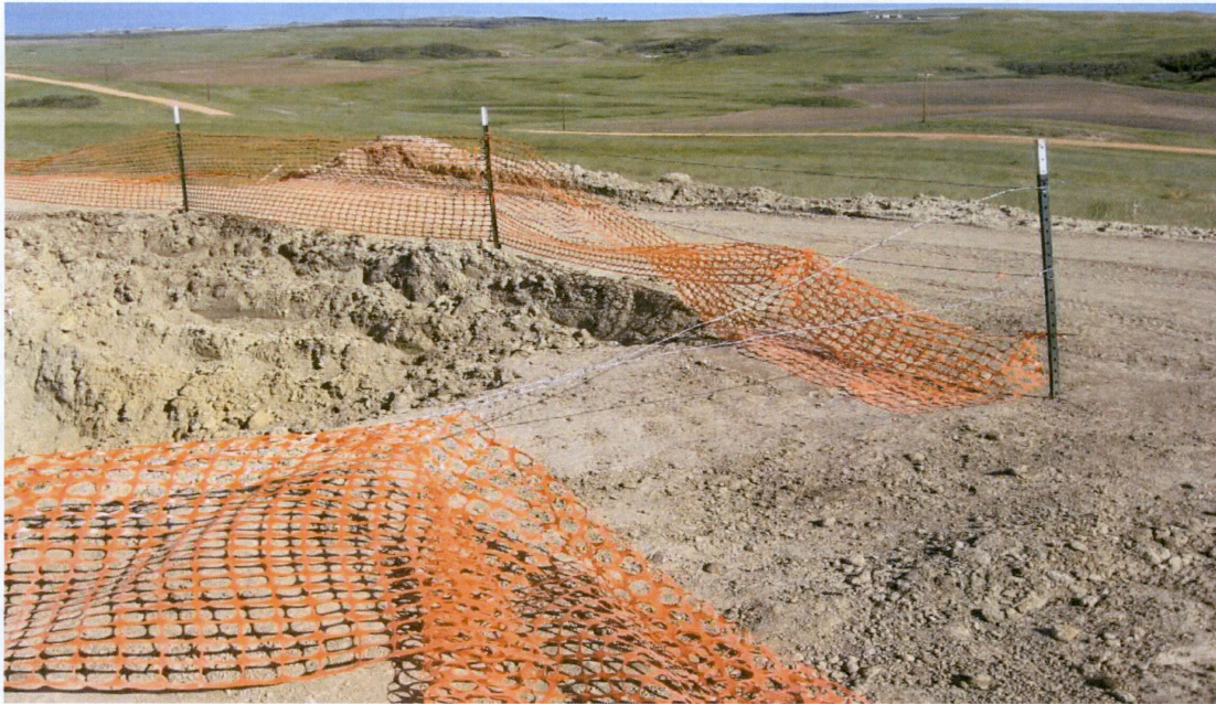
Photo 15 – Approx. Station 571+56. View of exclusion fence requiring repair.
