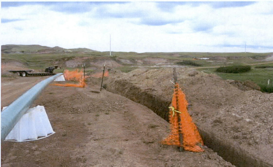
Photo 14 – Approx. Station 342+00. View of exclusion fence requiring repair.
