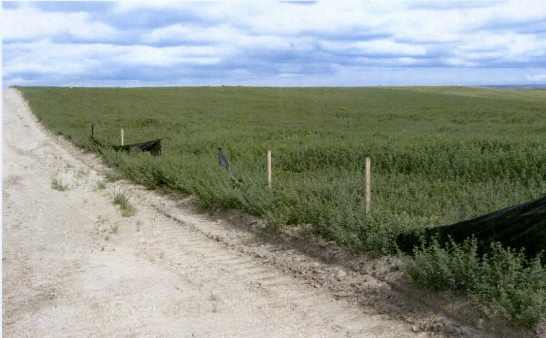
Photo 9 – Approx. Station 300+00. View of erosion control requiring repair.
