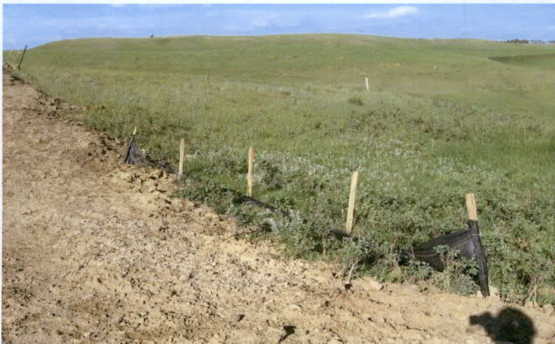
Photo 12 – Approx. Station 612+00. View of erosion control requiring repair.
