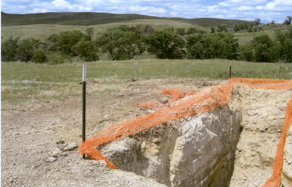
Photo 13 – Approx. Station 212+57. View of exclusion fence requiring repair.
