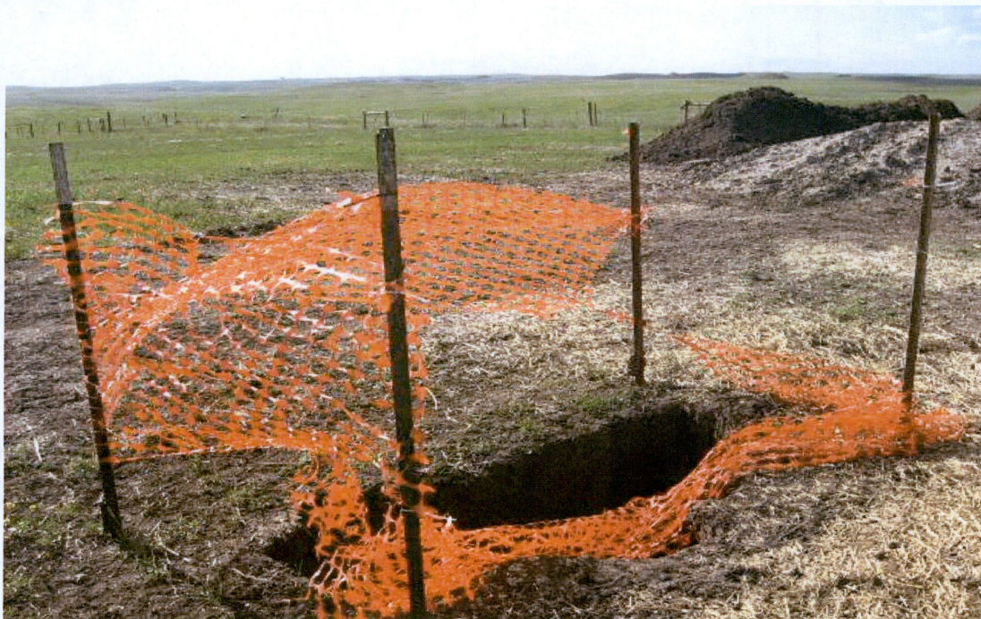
Photo 16 – Approx. Station 630+00. View of exclusion fence requiring repair.
