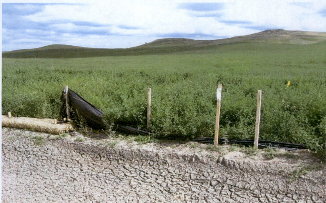
Photo 10 – Approx. Station 328+00. View of erosion control requiring repair.
