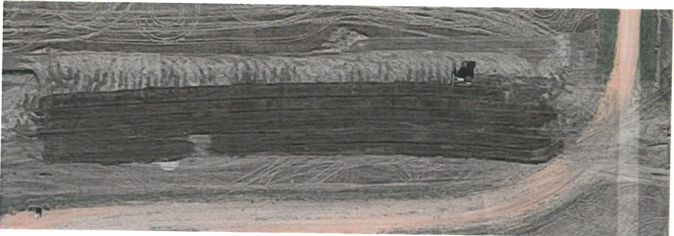
Approximate Sta. 53+00 Aerial Photo #5 of Top Soil Replacement over the Tesoro Pipe Line Trench Ready to turn south towards 40 th Street NW September 2016
