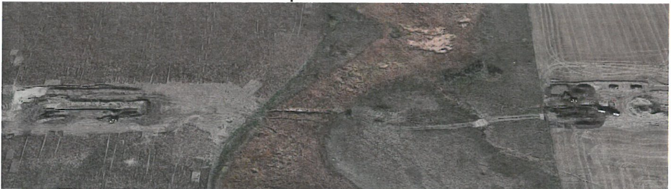
Sta. 16+20 to 21+60 Aerial Photo #3 Boring under Wetlands Stock Piling Top Soil for the Tesoro Pipe Line Trench East of Highway 1806 September 2016
