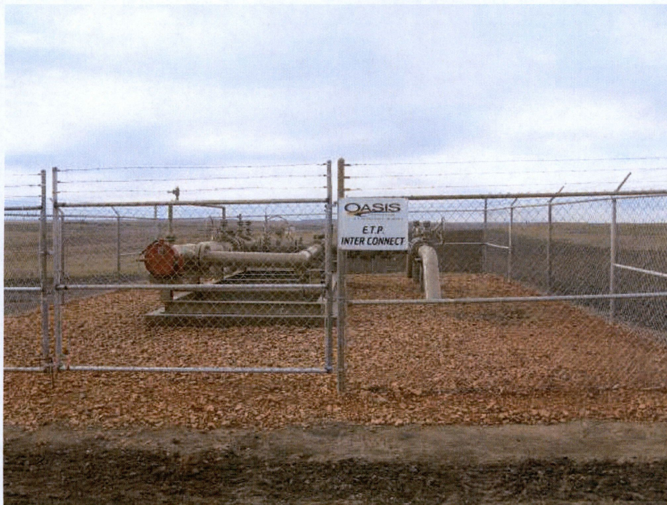
Photo 10 – Approx. Station 858+00. View of ETP interconnect valve.
