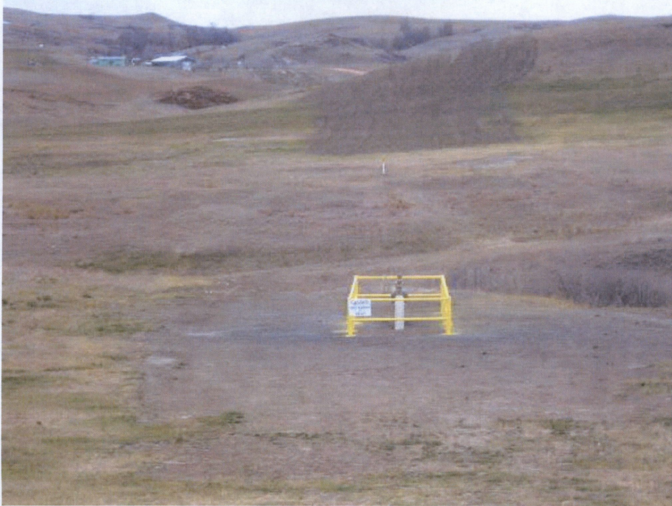
Photo 8 – Approx. Station 371+00. View of Main Line Valve.
