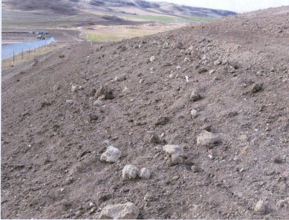
Photo 13 – Approx. Station 960+00. View of rocks from another project on Oasis right of way.
