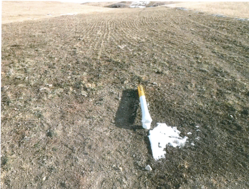
Photo 23 – Approx. Station 434+00. View of pipeline marker needing repair.
