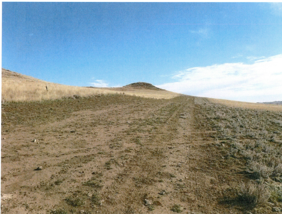
Photo 14 – Approx. Station 187+00. View of the right of way that requires additional seeding.
