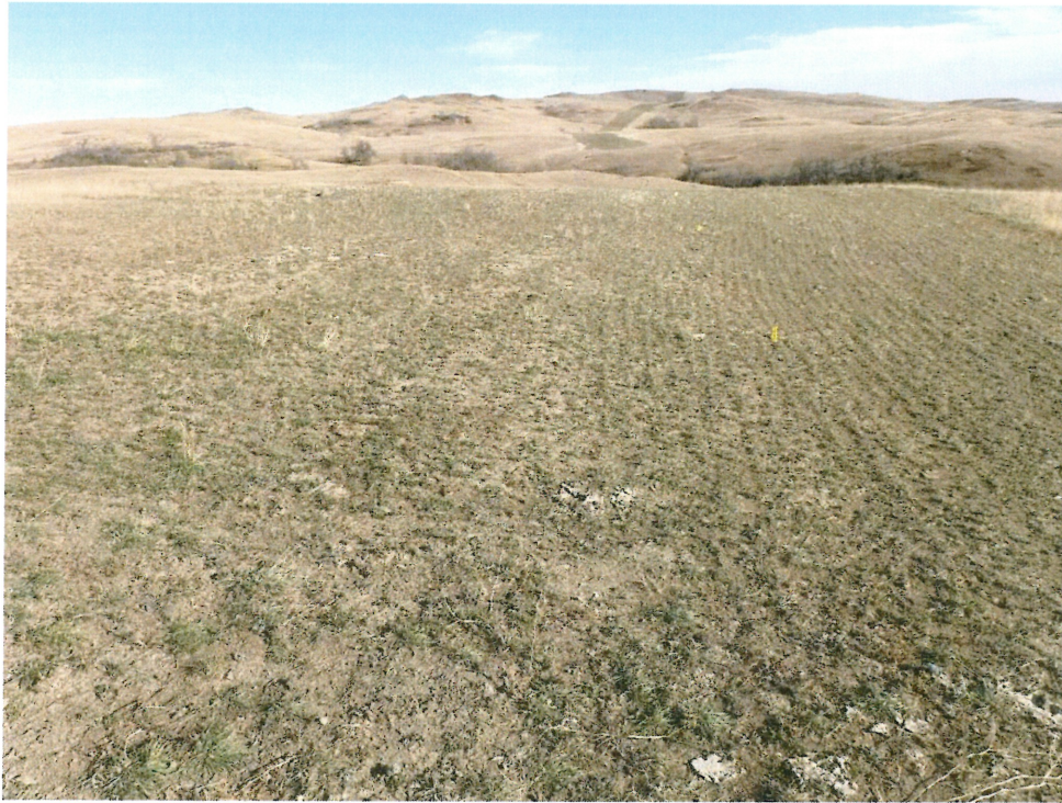
Photo 17 – Approx. Station 207+00. View of the right of way that requires additional seeding.
