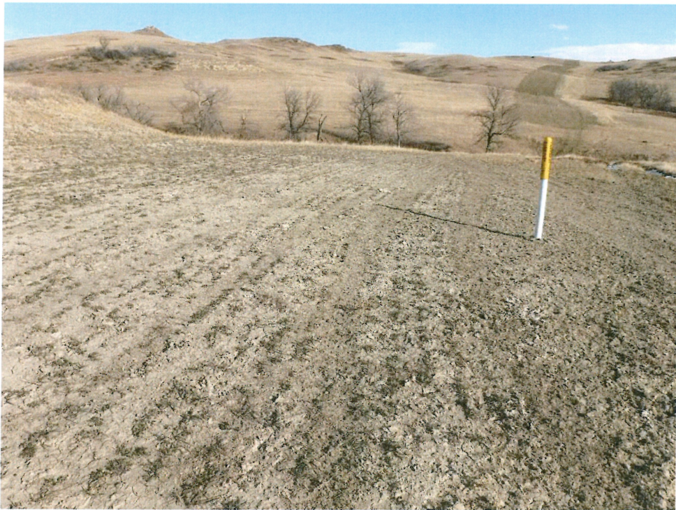
Photo 18 – Approx. Station 234+00. View of the right of way that requires additional seeding at HDD workspace.
