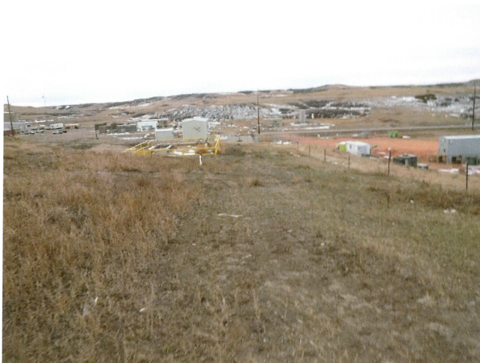
Photo 30 – Approx. Station 891+00. View of the right of way that requires additional seeding.
