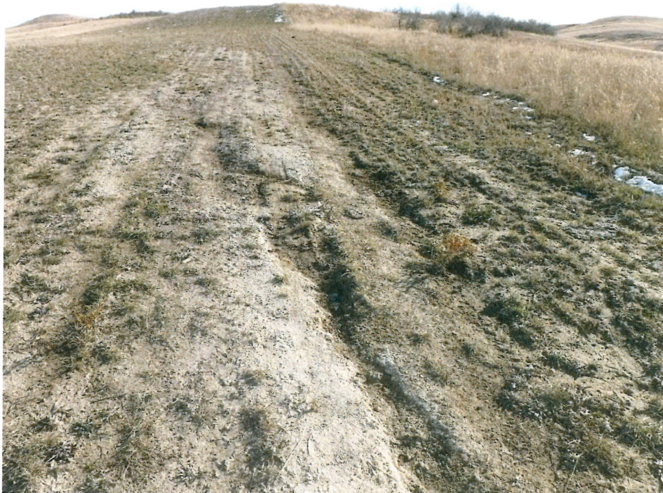
Photo 13 – Approx. Station 154+00. View of minor erosion.
