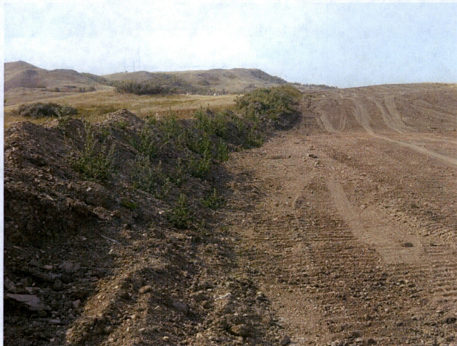
Photo 15: Located at station 354+00, looking north at graded Right of Way showing pipe installed in trench with subsoil backfilled and graded across Right of Way. Photo shows topsoil placed on edge of Right of Way ready to grade and level over Right of Way to original condition.
