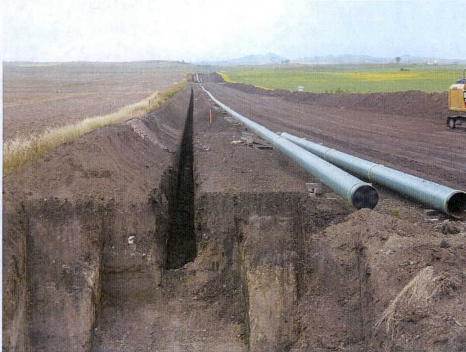
Photo 9: Located at station 126+00, showing grade Right of Way direction looking east with trench excavated. Pipe is welded and ready to place in trench. Photo shows subsoil placed on left side of Right of Way. Top soil placed along right side edge on Right of Way.
