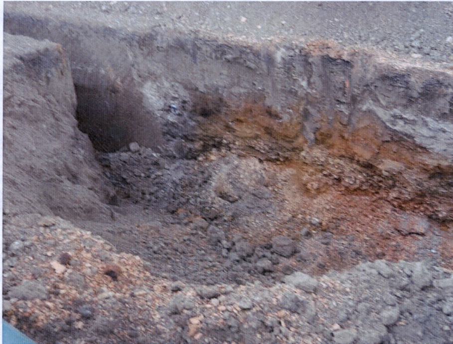
Photo 11: Located at station 141+00, photo showing open trench where existing line was hit while excavating trench. Hess line was not damaged and existing line location was not found or exposed.
