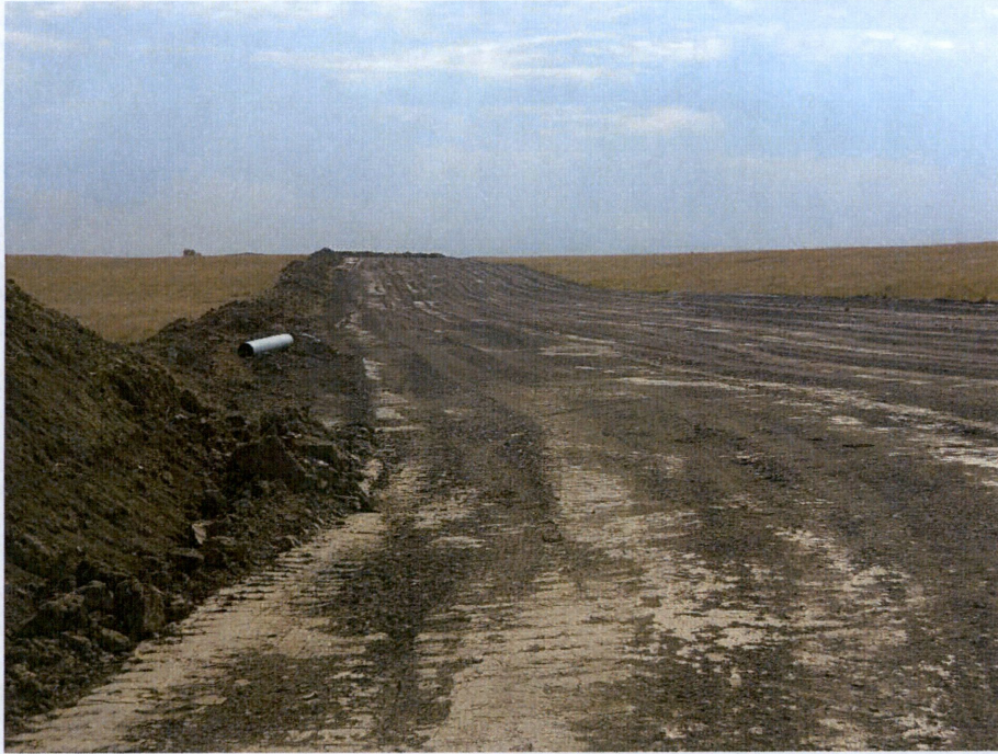
Photo 17: Located at station 420+00, looking west at graded Right of Way, showing pipe installed in trench with subsoil graded and leveled. Topsoil replacement and Right of Way cleanup still needs to be completed.
