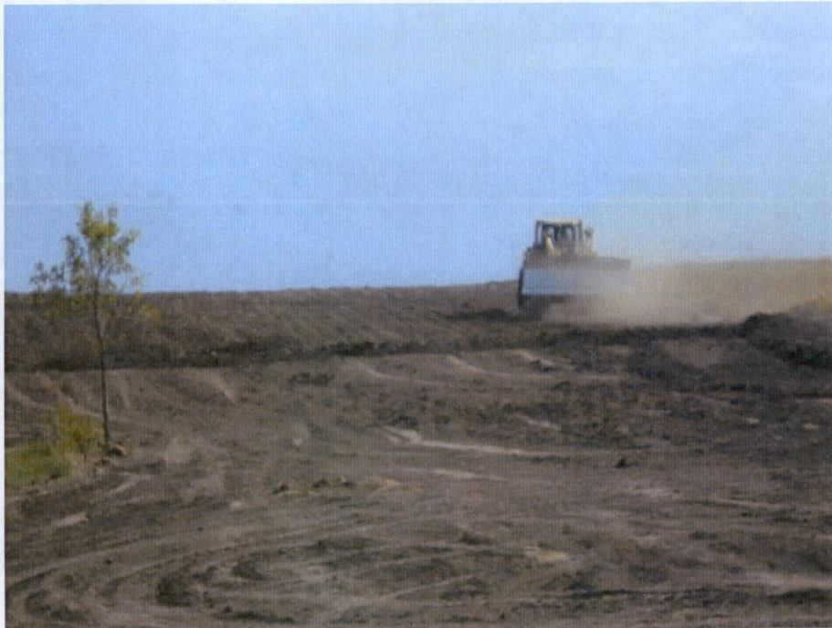
Photo 10: Located at station 288+00, looking south at Right of Way. Pipe installed in trench and backfilled. Contractor in process of installing and leveling Right of Way to original condition. Clean up in process.
