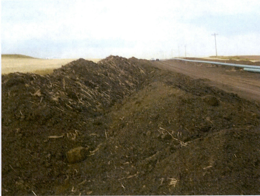
Photo 1: Located at station 6+00, showing Right of Way direction looking east with graded top soil placed on edge of Right of Way. Subsoil is pushed to left edge of topsoil, but is segregated and separated from each. Pipe is welded and sitting on skids ready for trenching.
