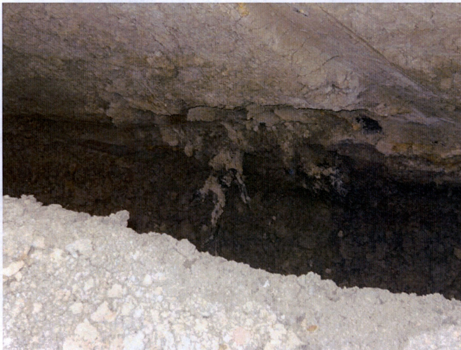
Photo 12: Located at station 141+00, looking inside trench where existing Hess pipeline was partially hit and disturbed during excavation of trench. Pipe was repaired by Hess and no liquid from pipe flowed into trench. Location of Hess pipe was mismarked during locating existing piping for trench work.
