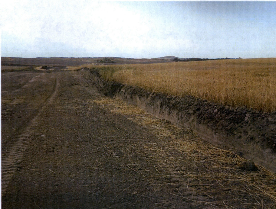
Photo 28: Located at station 570+00, showing graded Right of Way with 12 inches of topsoil removed. Grading showing subsoil below topsoil after grading completed.
