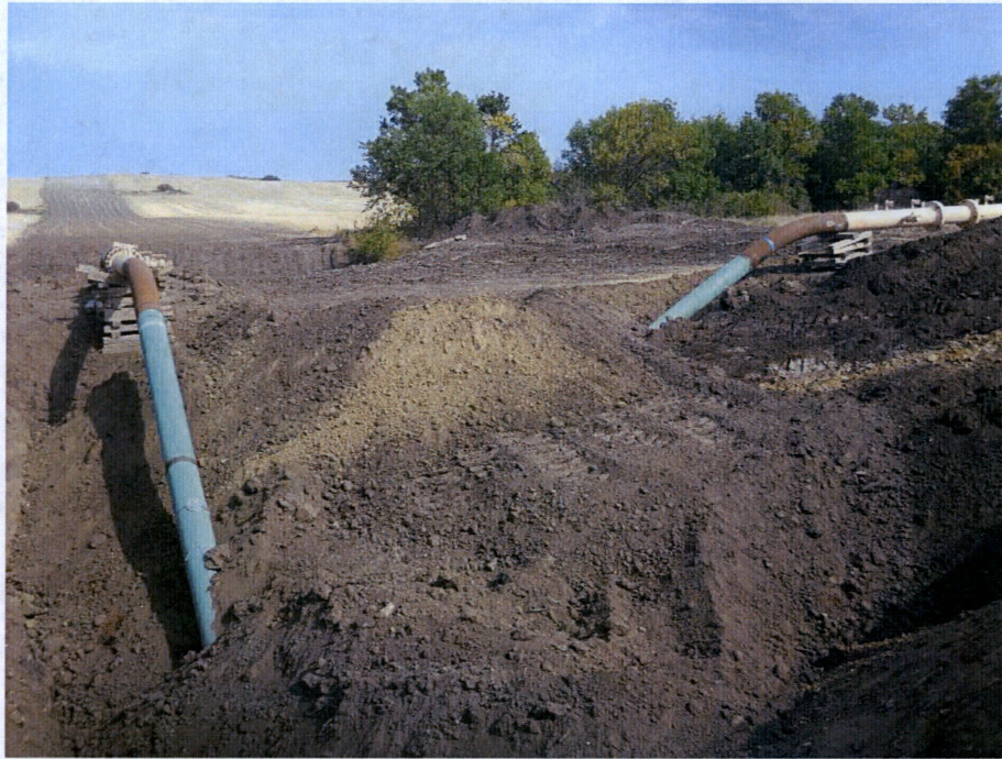
Photo 11: Located at station 319+52.27, looking at bore pit on east side of County Road 14. Photo showing piping and valve settings.
