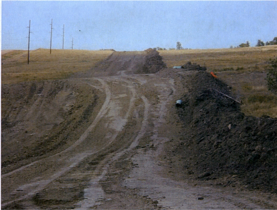
Photo 23: Located at station 474+00, looking north at Right of Way, showing piping installed in trench and backfilled. Subsoil has been regraded across Right of Way. Topsoil work has not started yet, shown on right side of photo. Clean up work across Right of Way is not completed.
