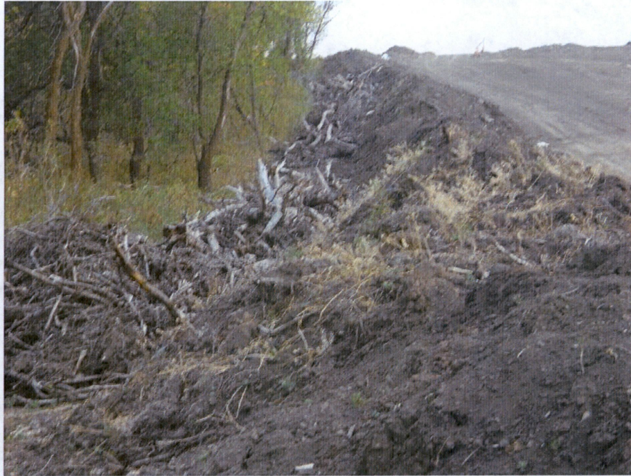
Photo 25: Located at station 492+00, photo showing Right of Way graded with piping in trench and backfilled. Topsoil shown on outside of Right of Way with a lot of dead timber located with topsoil, that needs to be cleaned up and removed.
