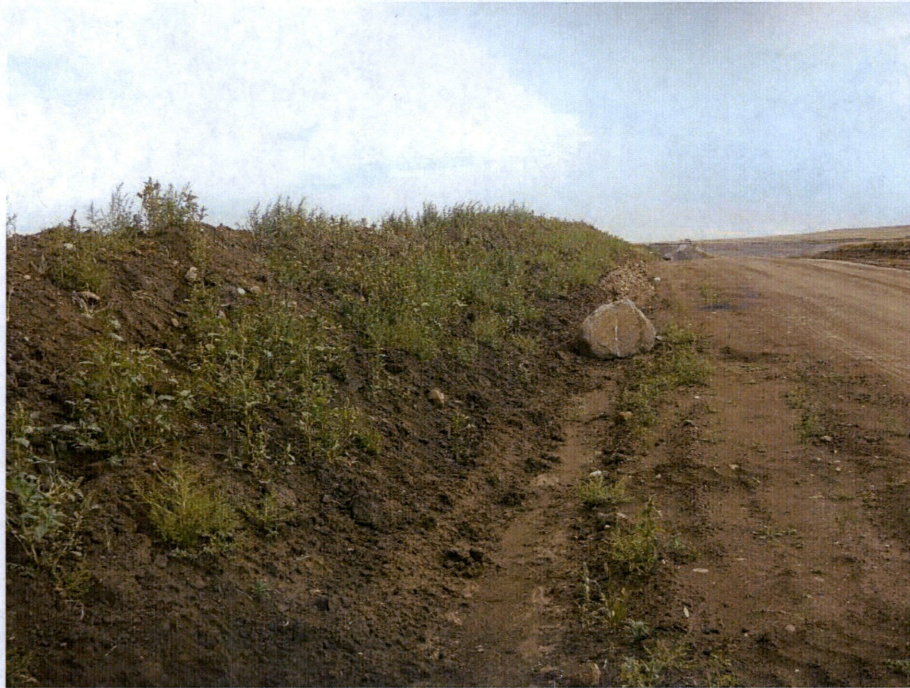
Photo 7: Located at station 248+00, Facing west, showing graded Right of Way with topsoil pushed off Right of Way edge on west side. Subsoil is pushed on Right of Way edge on left side. Rocks need to be removed from Right of Way when replacing topsoil.
