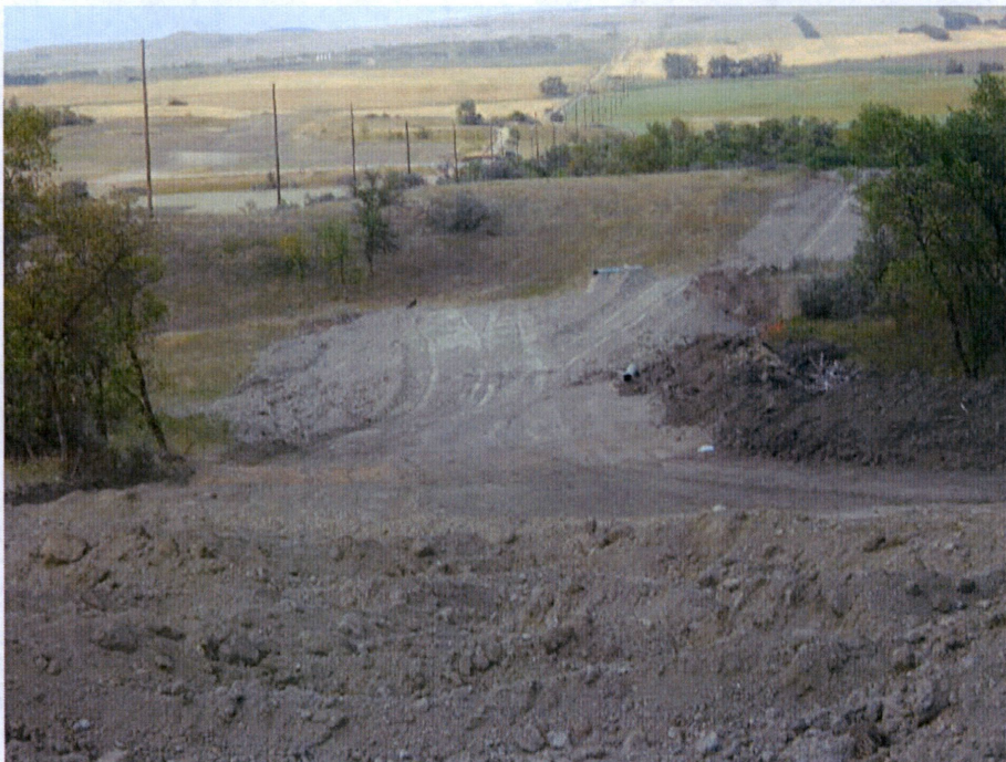
Photo 24: Located at station 483+00, looking north, showing subsoil grading started but not completed. Topsoil placed on edge of Right of Way, showing no work started. Clean up work across Right of Way not started.
