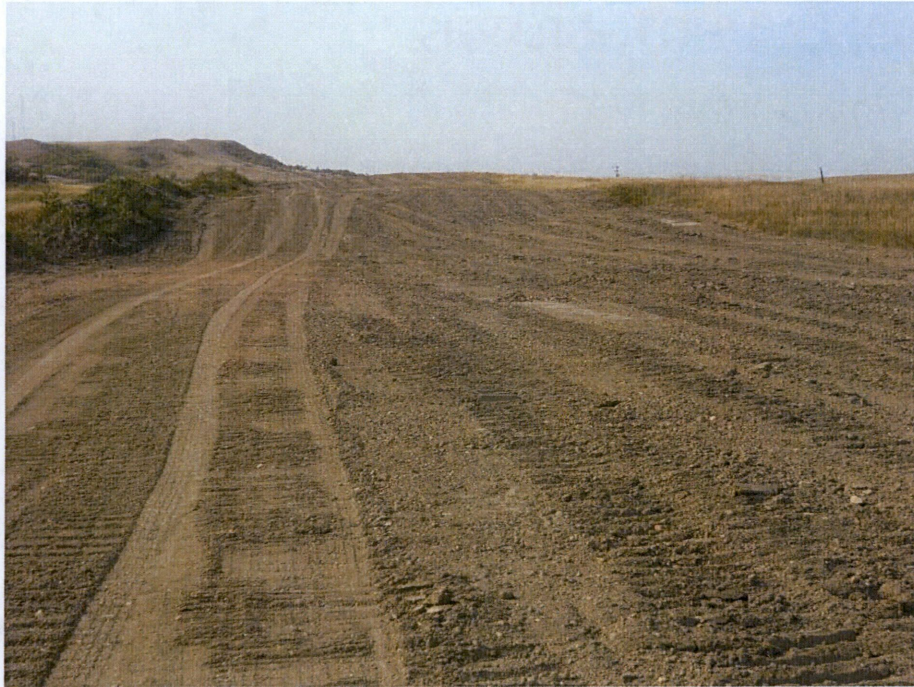
Photo 29: Located at station 600+00, looking north, showing graded subsoil across Right of Way levelled. Topsoil shown on left side of photo. Topsoil work not started yet.
