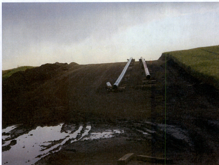
Photo 21: Located at station 204+00, showing Right of Way heading west. Station is at bore pit, location by County Road 14 that heads west. Right of Way has been stripped of topsoil which is located along left side (south edge) of Right of Way. Photo showing pipe welded and ready to be bored under County Road 14.
