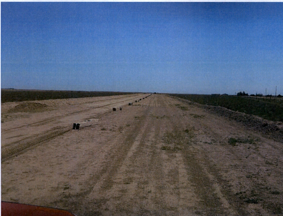
Photo 4: Located at station 27+00, showing Right of Way direction looking west graded with top soil pushed off Right of Way. Pipeline skids placed on Right of Way ready for piping.
