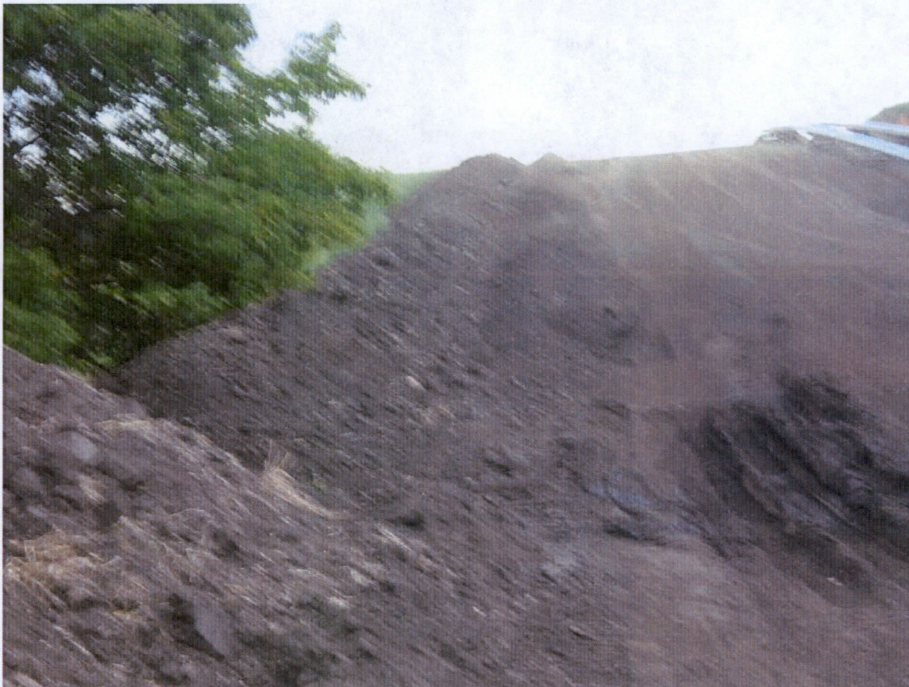
Photo 18: Located at station 198+00, showing Right of Way heading west. Station is at bore pit located at County Road 14 that heads east. Right of Way has been stripped with topsoil located at left side (south edge) on Right of Way. Topsoil depth stripped has been approximately 12 inches. Photo showing bore piping located on left side of photo.
