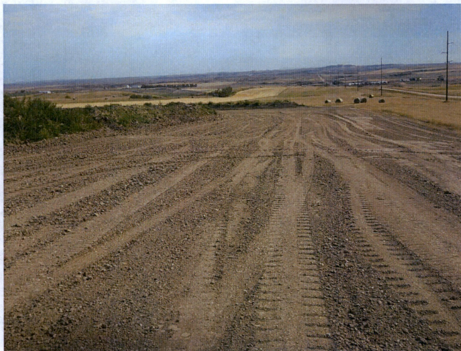
Photo 16: Located at station 435+00, looking south at graded Right of Way, showing pipe installed in trench with subsoil graded and leveled. Topsoil still shown placed on edge of Right of Way, needs to be regraded and returned to original condition.
