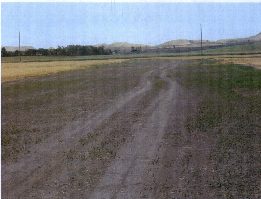
Photo 4: Located at station 222+00, Looking north of Right of Way with pipe in trench and Right of Way leveled and regraded to original condition. Right of Way has been cleaned and ready for seeding.
