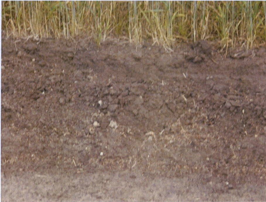
Photo 19: Located at station 203+00, showing stripped Right of Way with approximate topsoil depth of 12 inches. Photo is showing north side of Right of Way.
