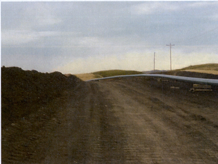
Photo 6: Located at station 66+00, showing graded Right of Way with welded pipe on skids ready for trenching. Topsoil is shown on edge of left side of Right of Way.
