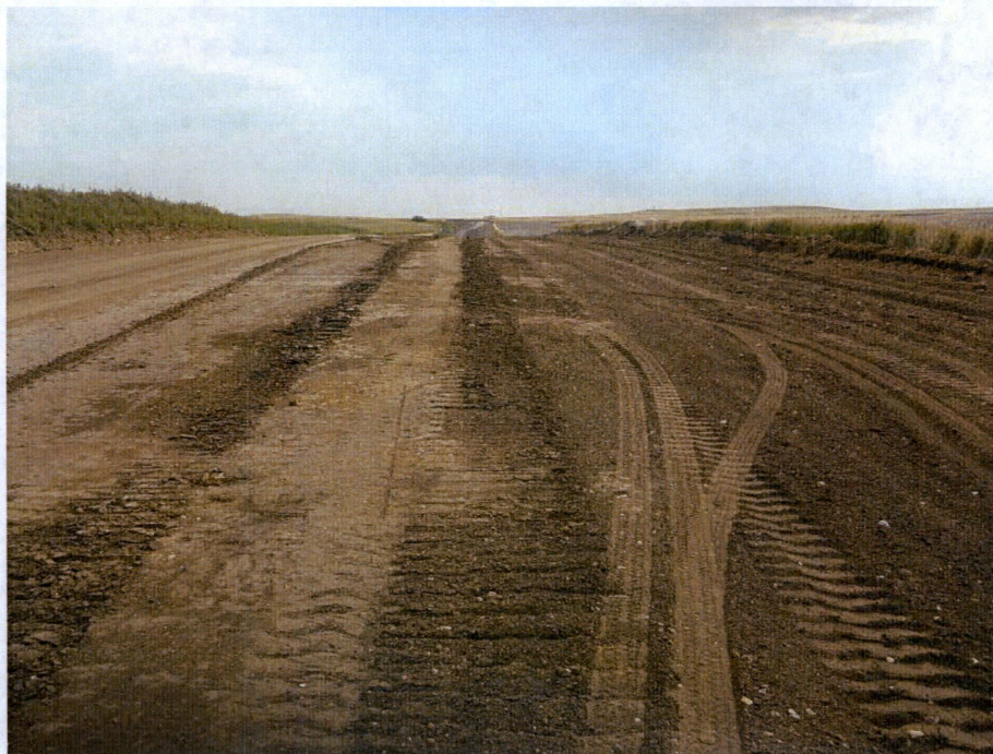
Photo 8: Located at station 264+00, looking west at graded Right of Way showing topsoil located on left side of Right of Way. Topsoil removal is approximately 12 inches deep.
