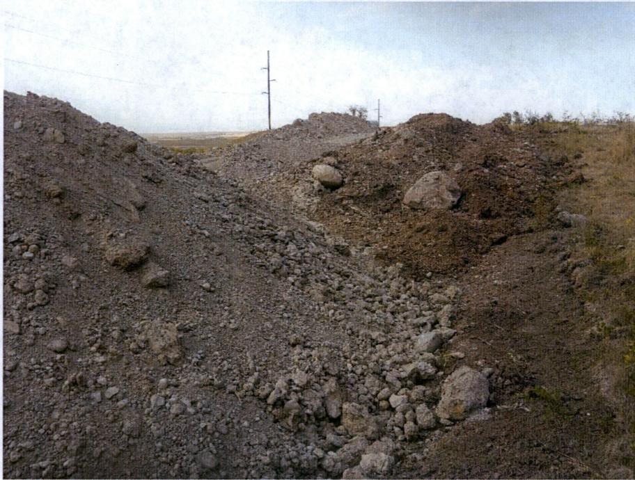
Photo 27: Located at station 519+00, showing Right of Way with segregated subsoil and topsoil along edge of Right of Way.
