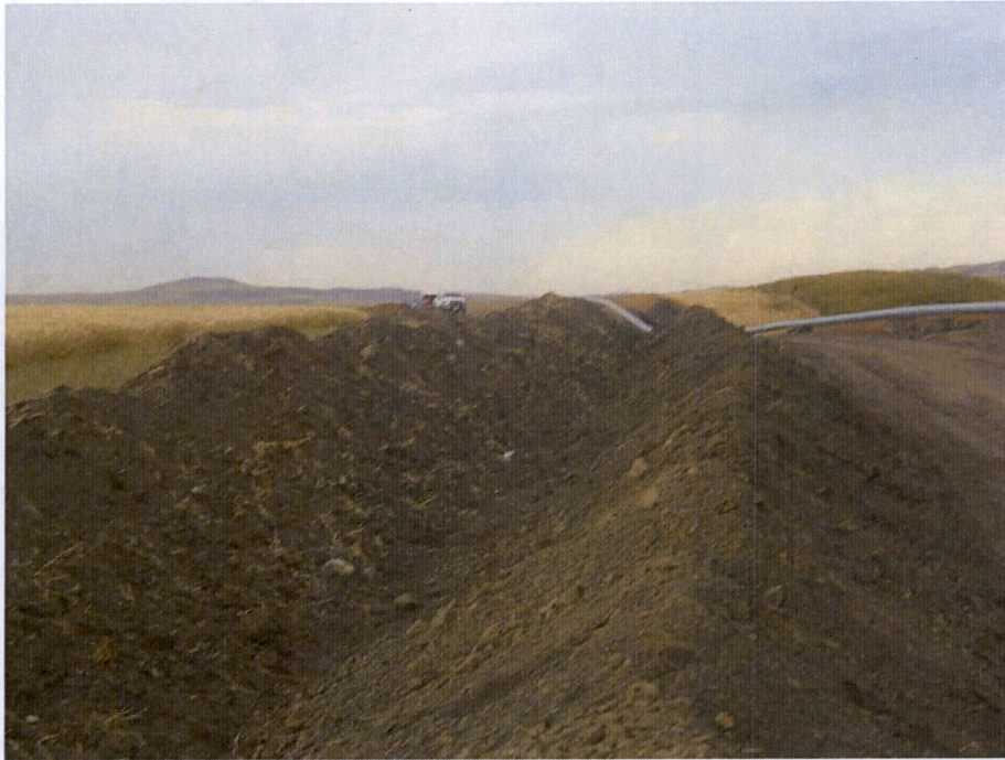
Photo 5: Located at station 48+00, showing graded Right of Way with subsoil located on left side on Right of Way and topsoil stockpiled on extreme left side of Right of Way. Both topsoil and subsoil have been kept segregated. Pipe has been welded and ready to install in trench.
