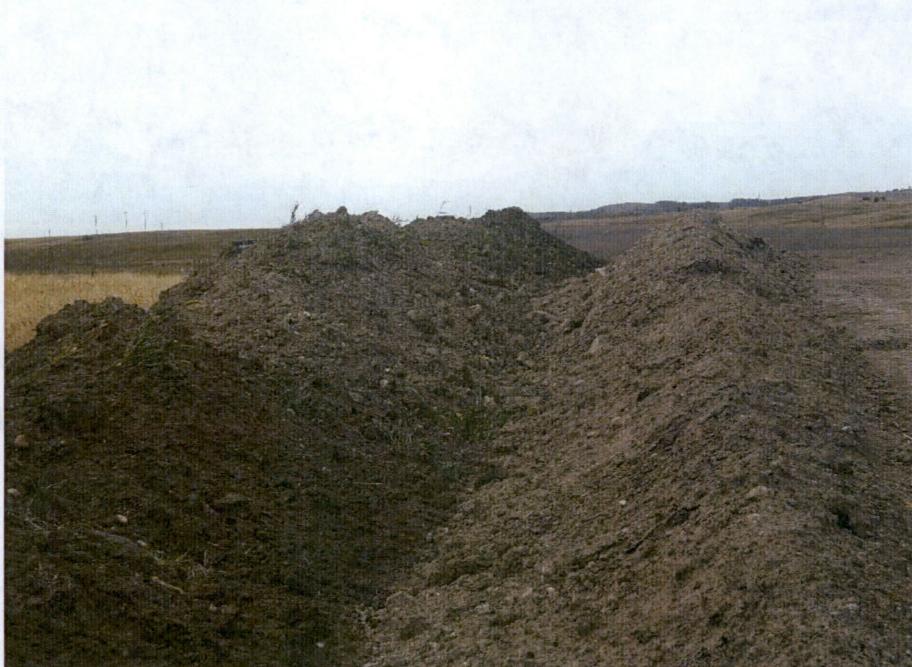
Photo 2: Located at station 207+00, showing Right of Way direction looking east. Right of Way has been stripped with subsoil on right side of photo and topsoil is located on the left side of photo and Right of Way. Both soil types are kept separated and segregated.
