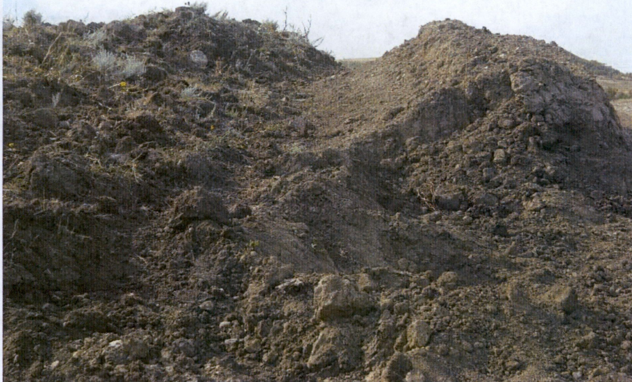
Photo 18: Located at station 450+00, looking north at Right of Way, showing subsoil and topsoil along the edge of Right of Way. Subsoil shown on right side of photo and topsoil on left side of photo. Both soil types are separated and segregated.
