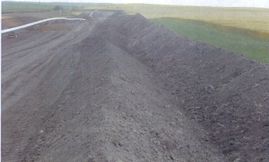
Photo 3: Located at station 21+00, showing Right of Way direction looking west graded with topsoil placed on the edge of Right of Way. Subsoil is pushed to the edge of topsoil, but is segregated and separated from each. Pipe is welded and setting on skids ready for trenching.
