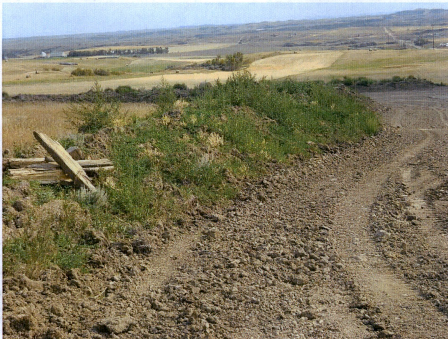
Photo 20: Located at station 438+00, looking south at Right of Way, then turning east, showing graded subsoil. Topsoil still placed on edge of Right of Way, needing to be regraded and levelled across Right of Way to original condition. Clean up work across Right of Way not completed.
