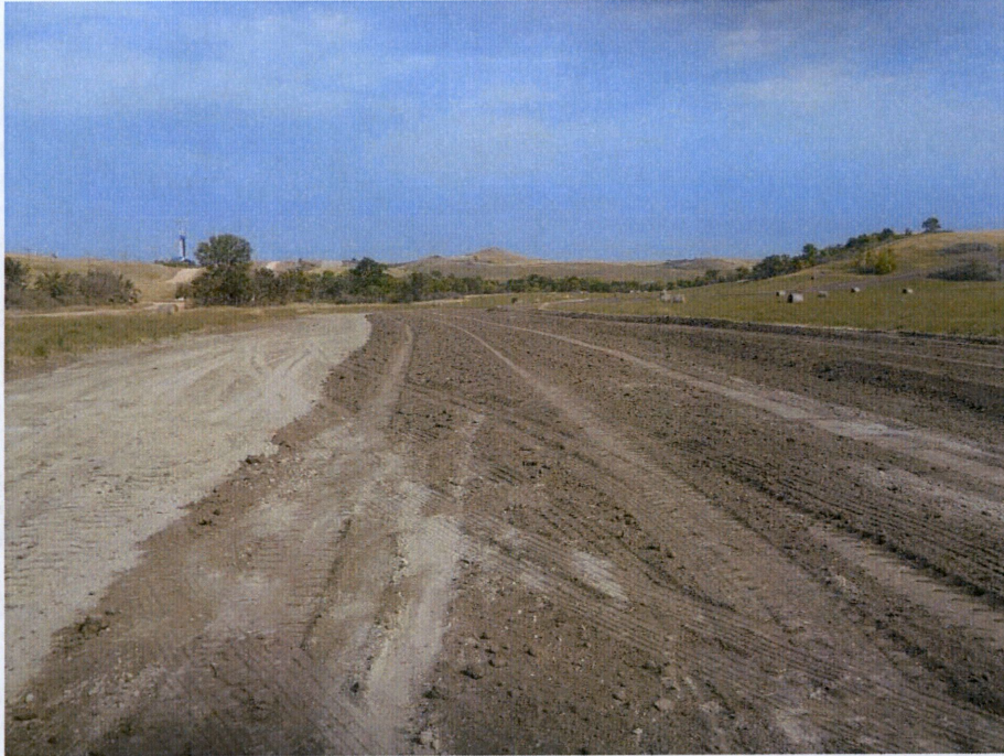
Photo 9: Located at station 297+00, looking east at graded Right of Way. Pipe installed in trench with subsoil replaced over Right of Way. Existing topsoil being regraded and leveled over Right of Way. Clean up in progress.
