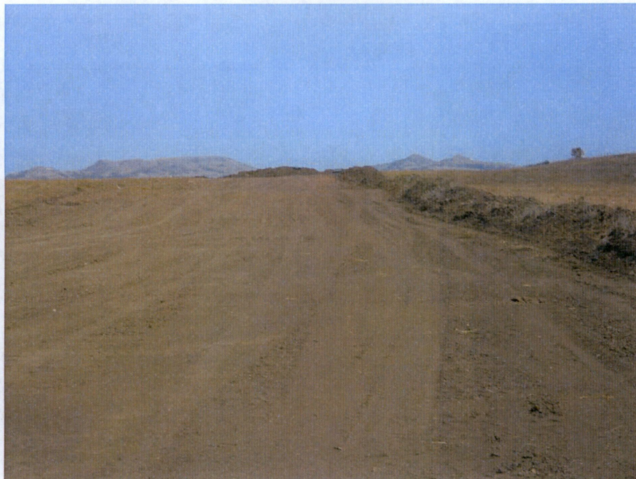
Photo 5: Located at station 225+00, taken from east end of Right of Way facing west, heading uphill. Right of way graded, with topsoil pushed to north edge of Right of Way easement. No BMP's have been installed along entire length of Right of Way for erosion control.
