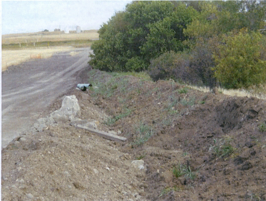
Photo 1: Showing Right of Way at station 198+00, Bore site located at County Road 14. Right of Way needs cleaning. Photo looking east, showing subsoil at lower left of photo with topsoil pushed off Right of Way on right side of photo. Both soil types are kept separated and segregated.
