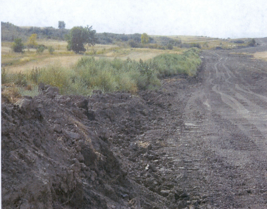
Photo 14: Located at station 345+00, looking north at graded Right of Way showing pipe installed in trench and backfilled. Topsoil still needs to be regraded and leveled out across Right of Way.
