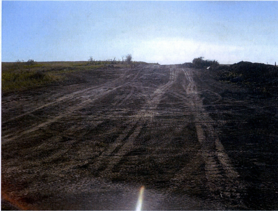
Photo 7: Located at station 78+00, showing Right of Way direction looking west with graded topsoil pushed to edge of Right of Way.
