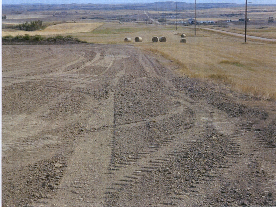
Photo 21: Located at station 444+00, looking south at Right of Way showing piping installed in trench and backfilled. Subsoil has been regraded and leveled across Right of Way. Topsoil has not been regraded and levelled out across Right of Way.
