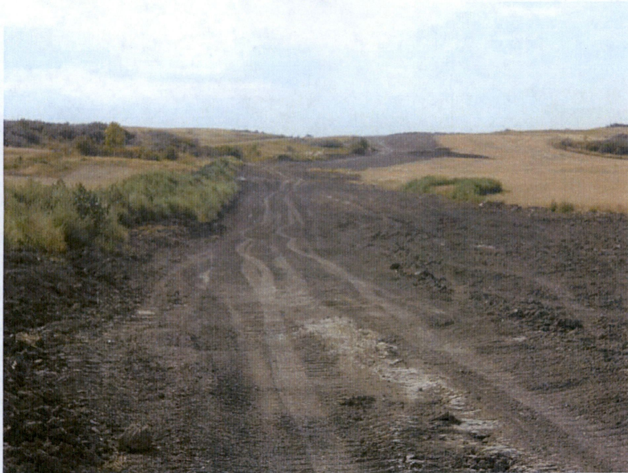
Photo 13: Located at station 342+00, looking north at graded Right of Way. Pipe installed in trench and regraded. Right of Way topsoil needs to have leveling finished and cleaned up to original condition.
