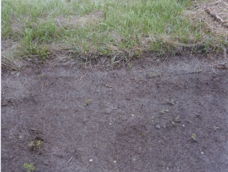
Photo 17: Located at station 165+00, photo showing stripped Right of Way with approximate topsoil depth exposed at 12 inches. Photo showing east side at edge of Right of Way.
