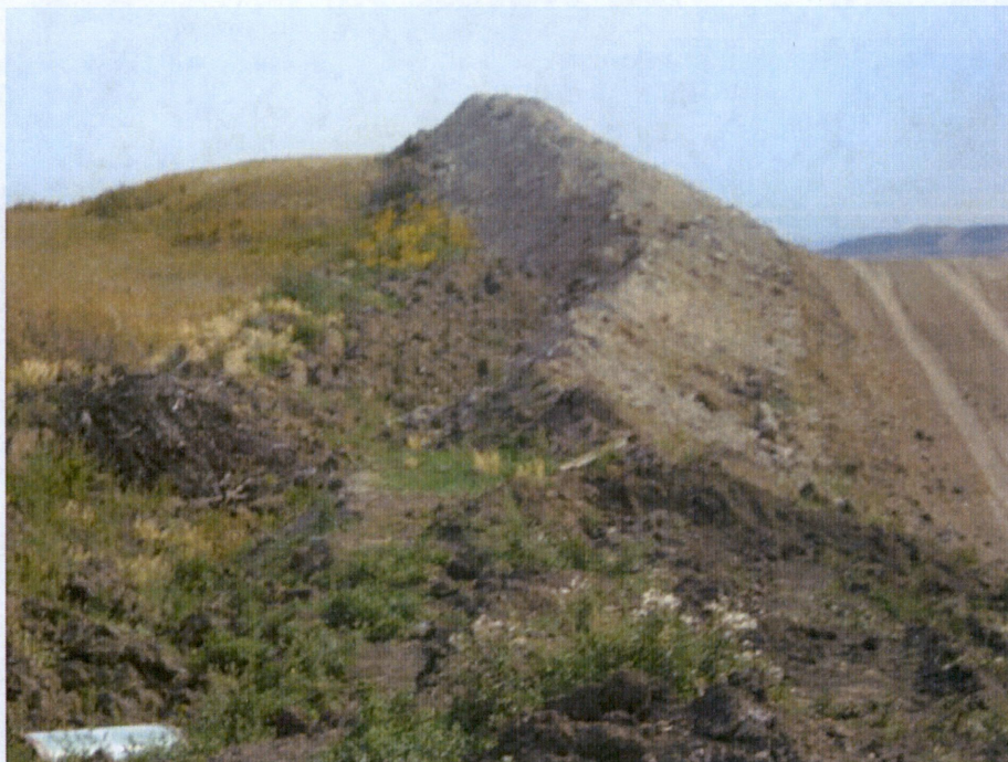
Photo 22: Located at station 459+00, looking south at topsoil placement along edge of Right of Way. Right of Way has been graded and ready to install topsoil over Right of Way to original condition.
