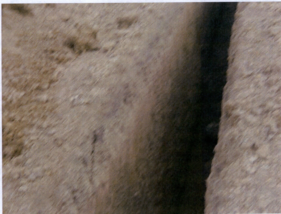
Photo 15: Located at station 148+00, showing trench work completed on Right of Way ready to place piping in trench.
