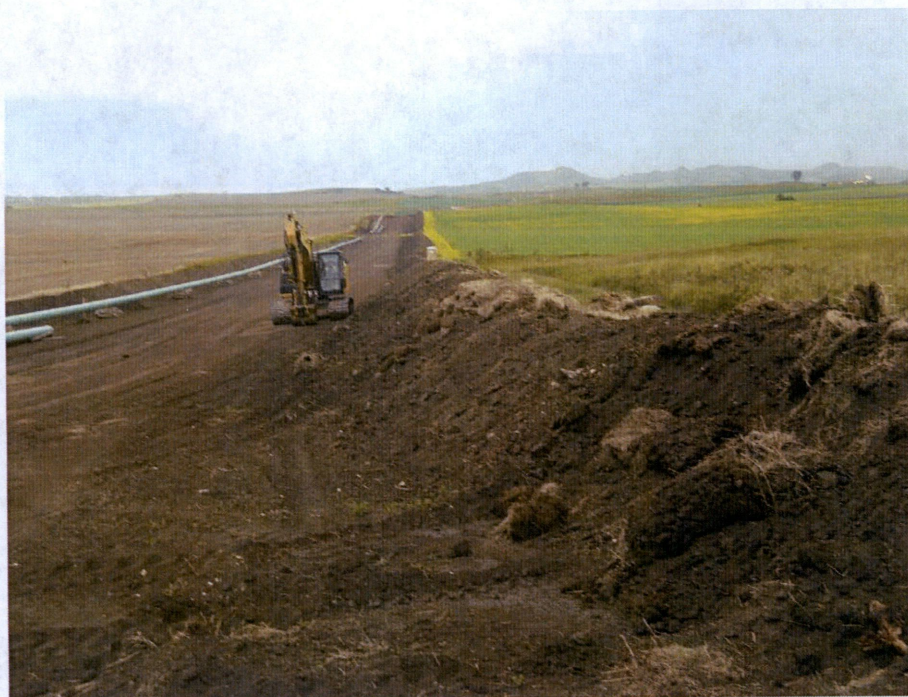
Photo 16: Located at station 162+00, Photo looking north showing stripped Right of Way. Photo showing topsoil placed on east edge of Right of Way. Subsoil is placed on west edge (left side) along Right of Way.
