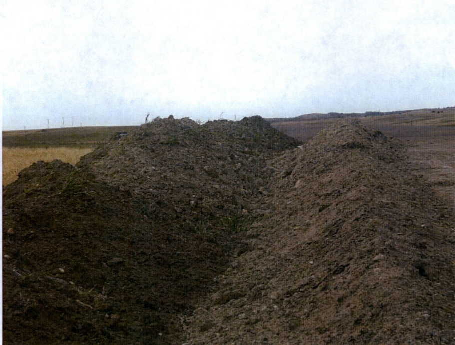
Photo 12: Located at station 324+00, looking at graded Right of Way showing subsoil and topsoil pushed off of Right of Way. Both soil types are segregated and separated as required.
