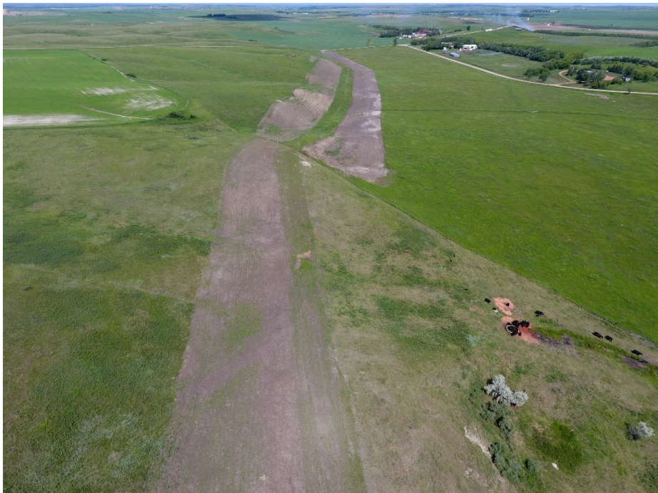
Location 32, Looking Northwest (47.886139, -102.911003) Multiple pipelines in this area. Recent work assumed to be from a different pipeline
