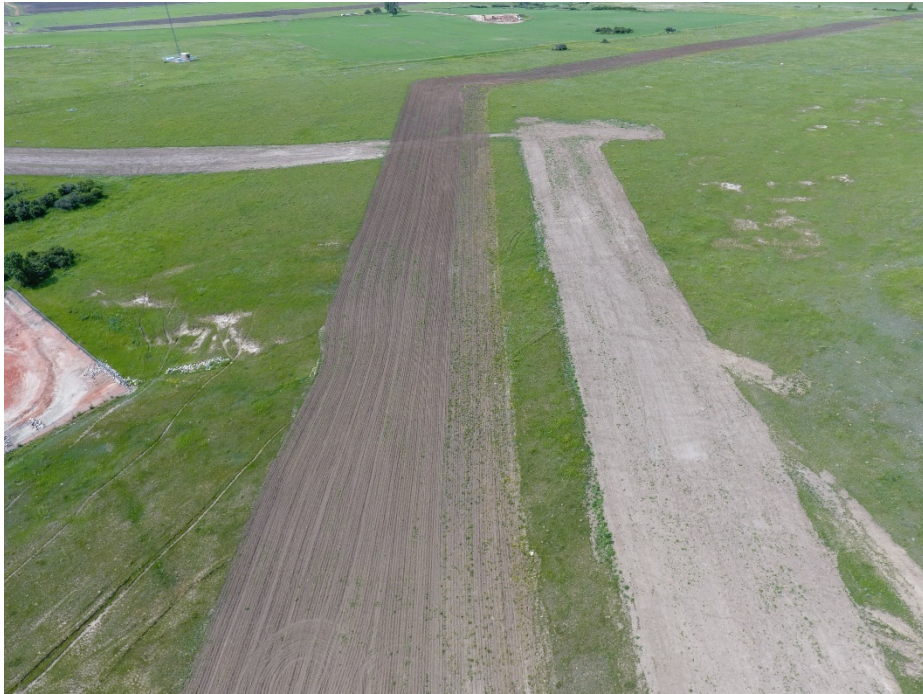
Location 27, Looking Southwest (47.857288, -102.88588) Multiple pipelines in this area.
