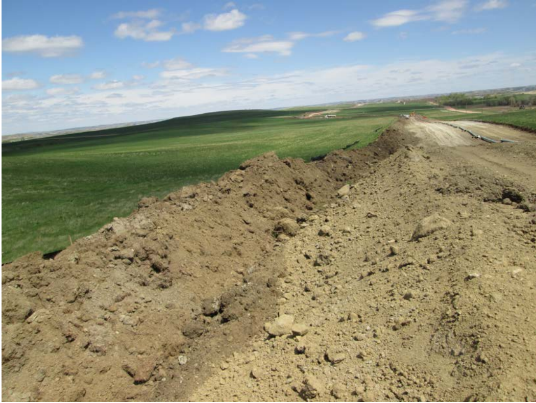
Above: Photo 11 (pt. 278) – Direction looking east. Side-sloping/two-toning area, used to level hill slope. Topsoil pile on far left of photo.
