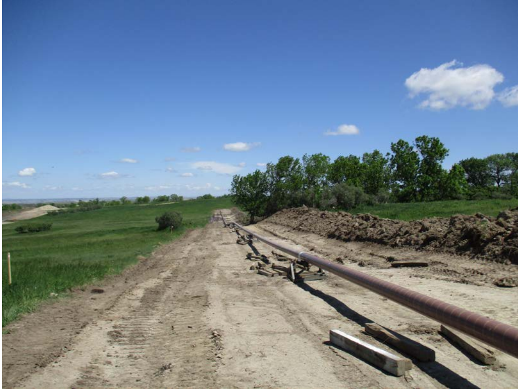
Above: Photo 17 (pt. 437) – Direction looking north. Bore area. Topsoil has been removed on additional bore pull back area, 50-ft ROW. To the far left of the photo is the pipeline ROW.
