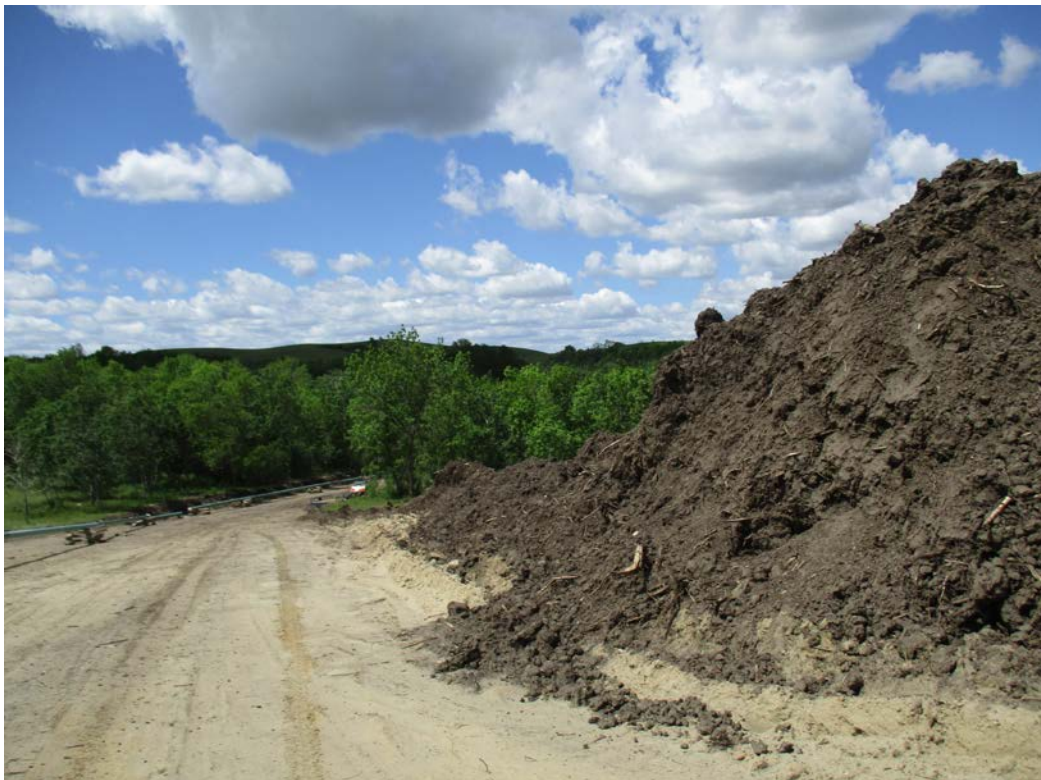
Below: Photo 18 (pt. 438) – Direction Looking west. Wooded ravine has a smaller ROW, topsoil from woody ravine brought up and piled. Woody debris in topsoil pile.
