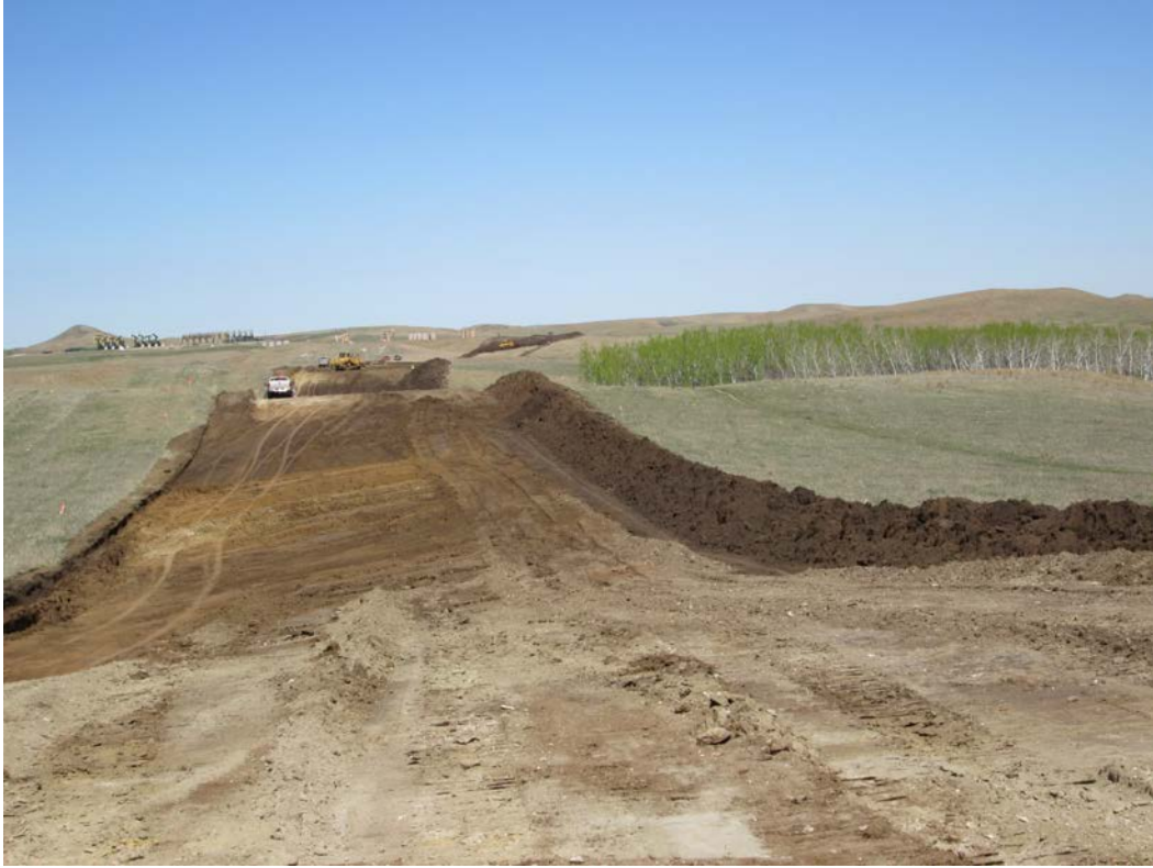
Above: Photo 5 (pt. 269) – Direction looking south. Topsoil stripped (far right) in two-toning area. There is space between topsoil and subsoil piles.
