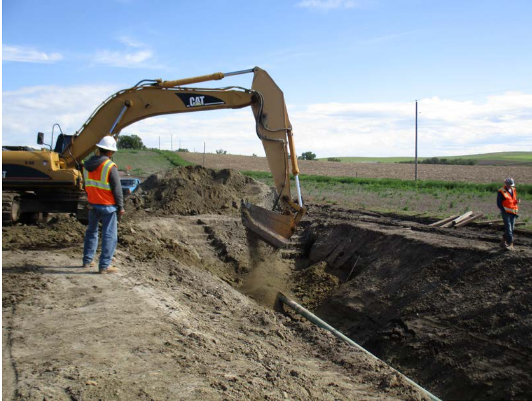
Above: Photo 15 (near pt. 433) – Direction looking north. The excavator uses a shaker with \frac{3}{4} -inch screen, used for rocky areas. The area around the pipe is padded with this finer material/soil from the shaker, 4-12 inches around the pipe, to protect the pipeline.
