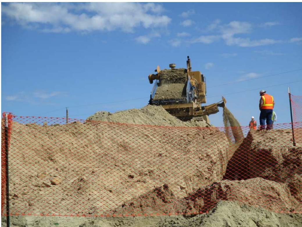
Below: Photo 16 (pt. 434) – Direction looking north. Padding machine, used to get rocks out of subsoil stratum. The loose fill will compact down around the pipe.
