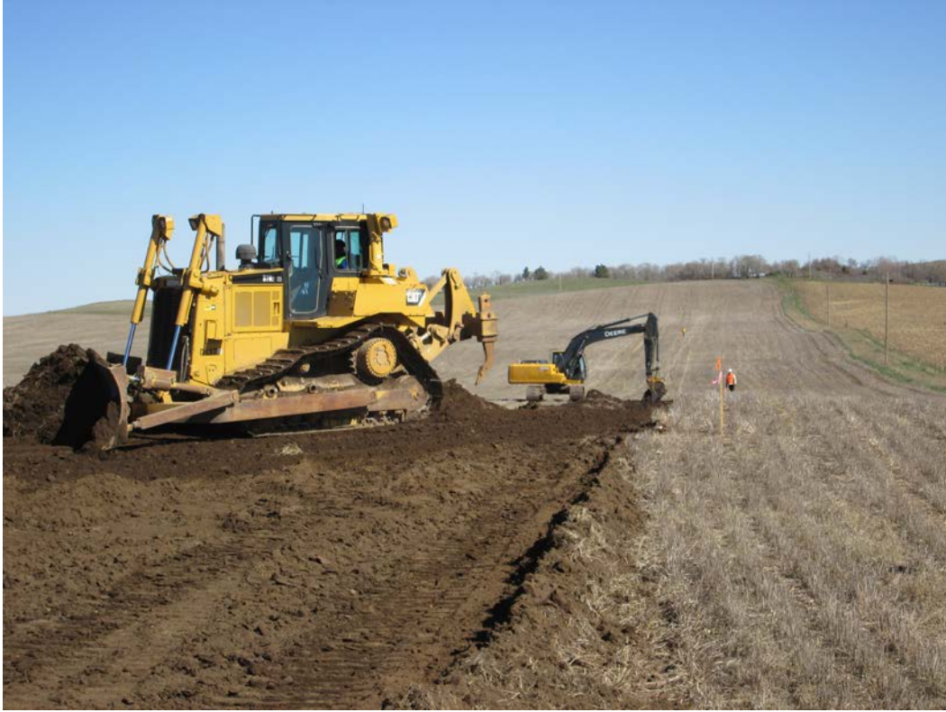
Above: Photo 1 (Point 267) – Direction looking north. Start of topsoil stripping. Dozer and excavator/hoe were used in this area, because this was a potential wet area, the excavator was used to start the topsoil stripping so the dozer could get in there, and would not twist and turn and mess up the area or take an incorrect amount of topsoil.
