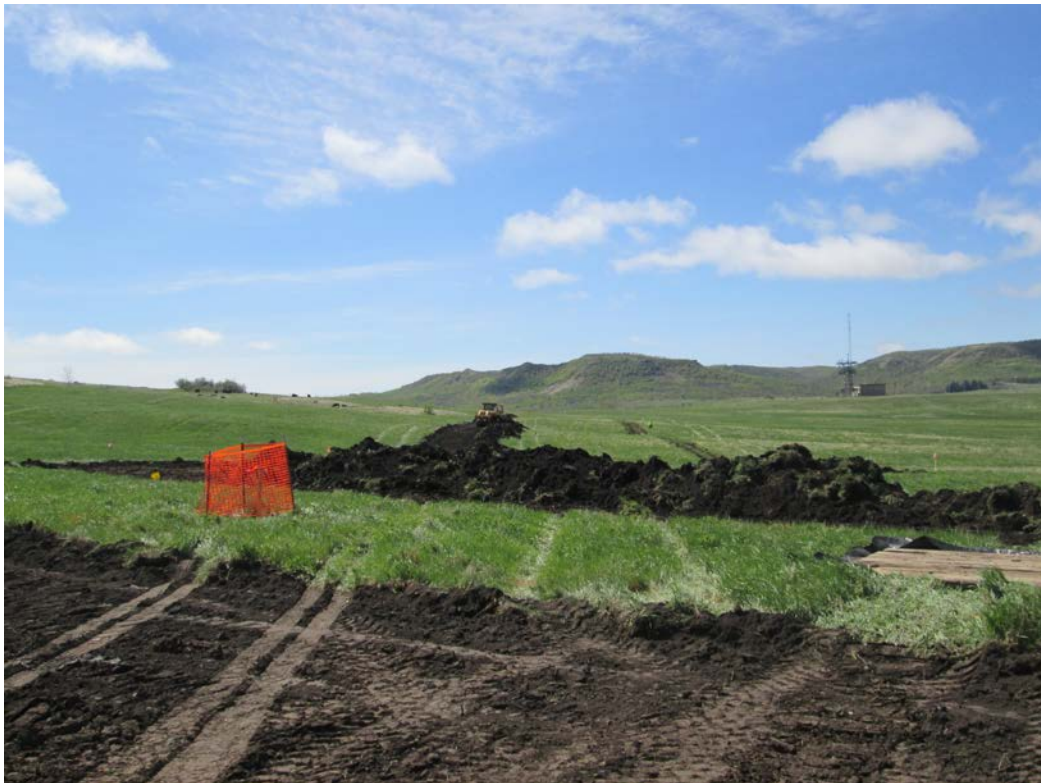
Below: Photo 22 (pt. 275) – Direction looking south. Another line runs through here, this area will be bored under. Dozer stripping topsoil.
