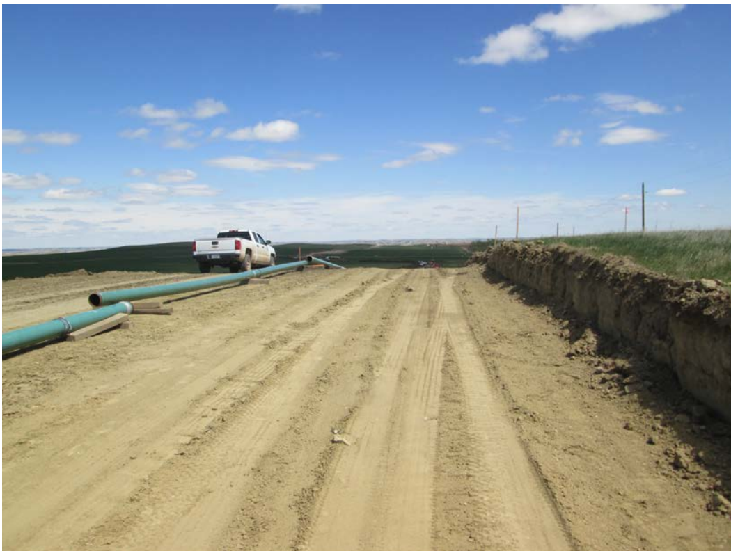
Below: Photo 12 (near pt. 278) – Direction looking east. Side-sloping/two-toning area, used to level hill slope. Can see cut into hill on far right of photo.
