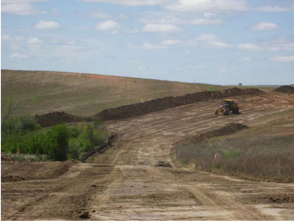
Above: Photo 9 (pt. 276) – Direction looking west. Neck down location; observe silt fences in front of trees and ravine area.
