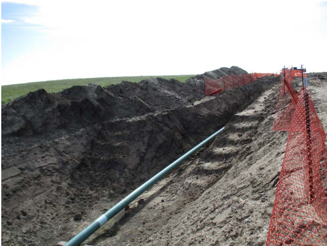
Below: Photo 14 (pt. 432) – Fence around trenched area, with stairs cut out along the sides. Subsoil pile to the left of photo.
