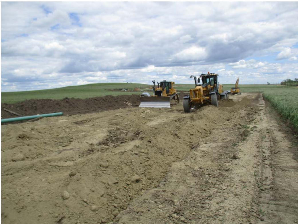
Below: Photo 20 (pt. 442) – Direction looking east. Trench just backfilled, equipment smoothing out area.
