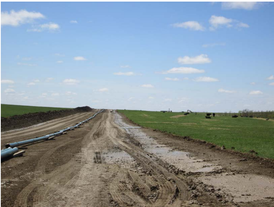
Below: Photo 10 (pt. 277) – Direction looking west. Topsoil stripped and area smoothed. The slurry from hydrovac truck was dumped and ran across edges of ROW. Clean water and mud/bentonite was used. Slurry was only dropped on ROW after topsoil stripped and if landowner approved.
